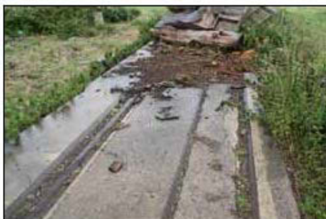
Figure 42. Detail of rails on one of the linear concrete bases of the gantry path.
