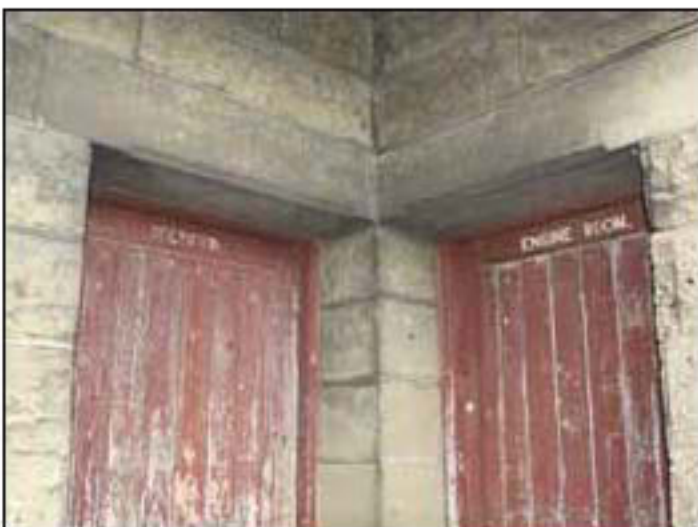
Figure 32. Detail of powerhouse doors, showing high quality of masonry and good condition of paintwork on panelled wooden doors.
