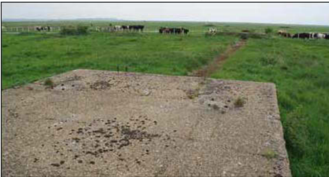
Figure 48. Looking northwest along arm of outer and longer velocity screen mast base.
