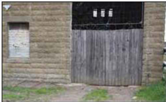
Figure 36. Detail of main workshop entrance, from the south-east. Standard gauge rails are visible on the ground heading into the workshop. Also visible are narrow gauge rails apparently heading under the walls to the left of the entrance.
