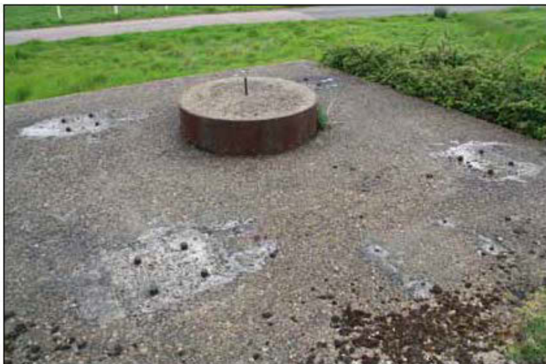
Figure 49. Footprint of velocity screen mast on concrete base.
