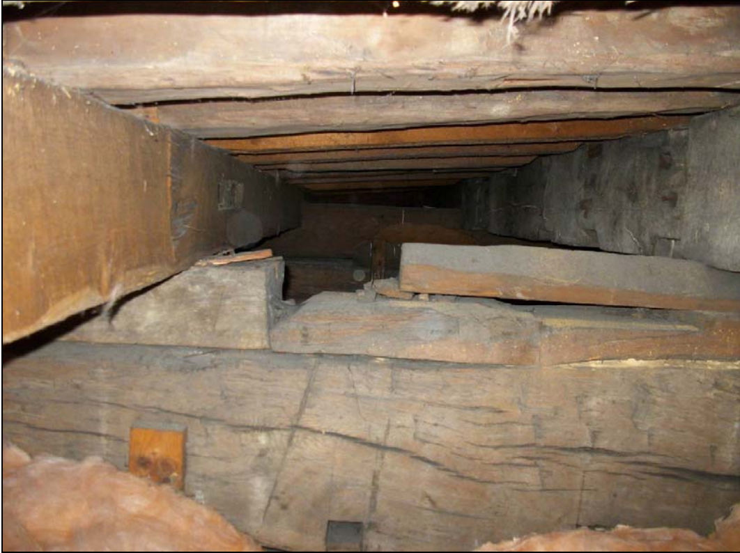
Figure 40: Infill roof, photograph taken by putting camera through entry hatch (Alison Arnold)
