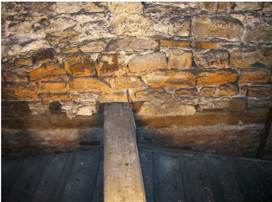
Figure 8: Photograph showing the beams in the wall between this roof (above the Throne Room) and the Long Dining Room, looking south (Alison Arnold)
