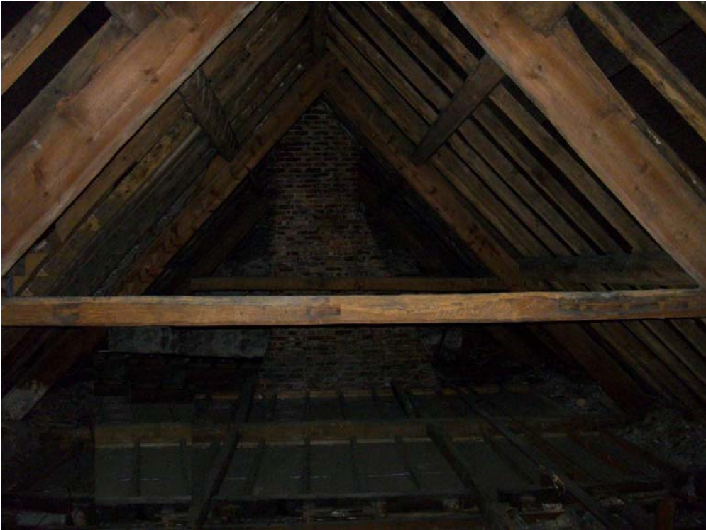
Figure 9: Principal rafter roof over the Stairway; the floor structure contains a number of reused oak timbers, looking west (Alison Arnold)
