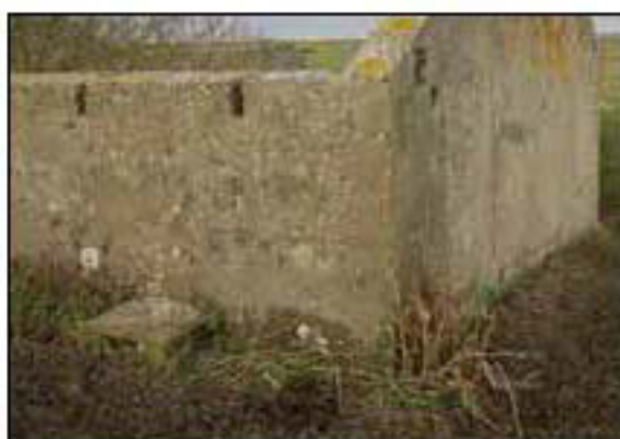
Figure 12A: An example of the concrete ventilation shafts visible buried in the bunds on the south elevation of the most northerly row of magazines.
