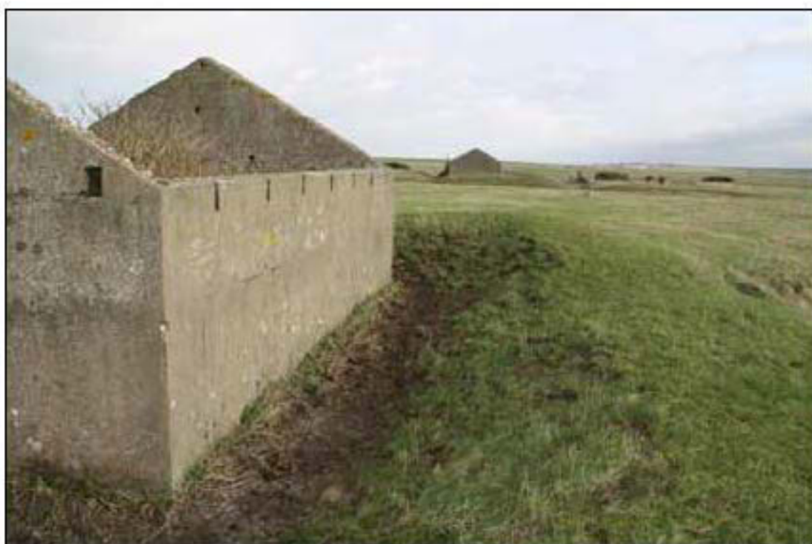
Figure 18: The western magazine of the central row has a clear gap between its southern elevation and the protective bund, in contrast to the row of magazines to the north.
