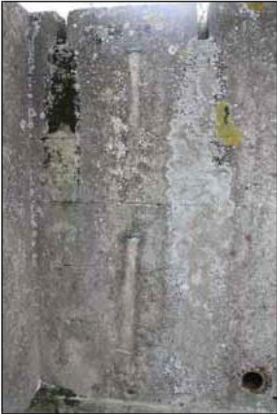
Figure 14: An example of the copper alloy fixings for the lightning conductors which were attached to each magazine. The ceramic vent pipe to the east of the entrance porch can also be seen.
