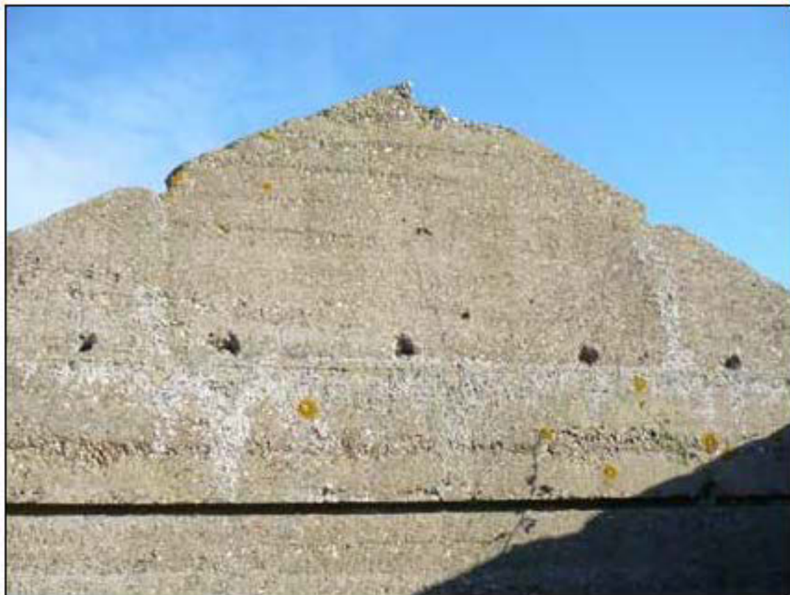
Figure 11: Small holes on the interior surface at the base of the gables that may indicate the position of a ceiling.
