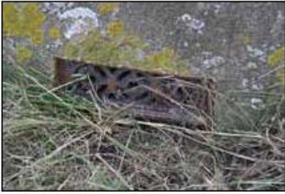
Figure 13: An example of the air bricks visible in the northern elevations of the magazines to the west and east of the porch.
