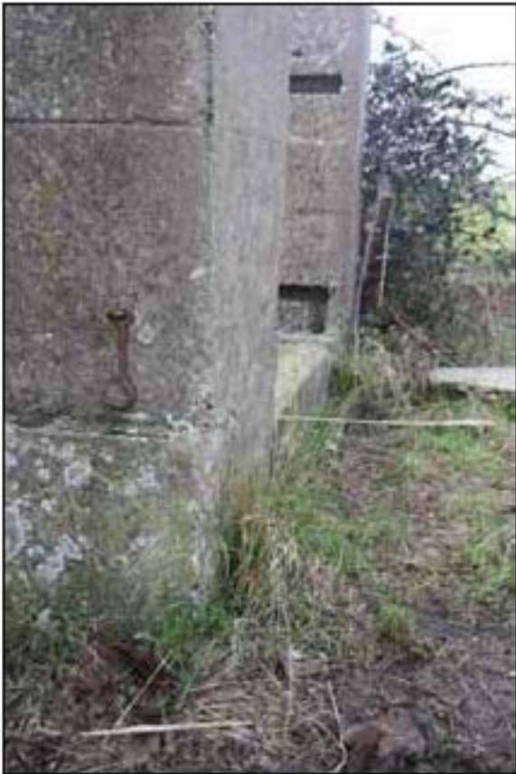
Figure 9B: Hook on east elevation of porch for securing door when open.
