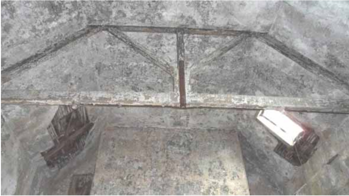
Figure 11: Sockburn Hall, north rear-range roof, photograph taken from the north-west (Alison Arnold)
