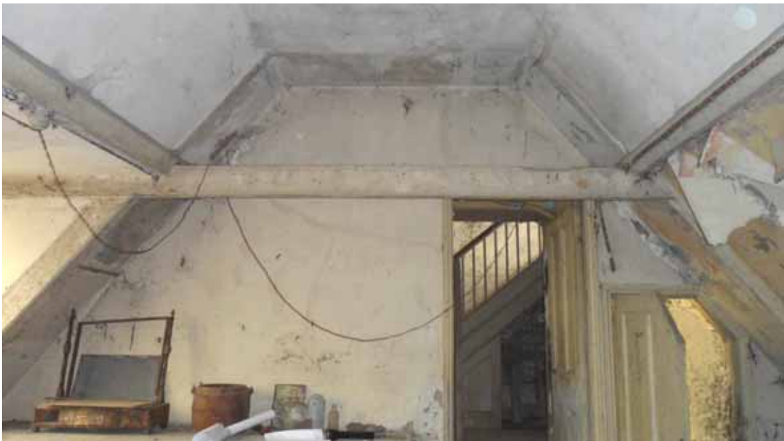
Figure 12: Sockburn Hall, south-rear range, truss 1, photograph taken from the north-west (Alison Arnold)
