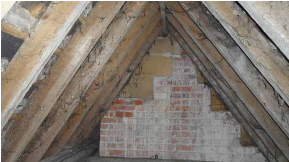
Figure 10: Sockburn Hall, north range roof, photograph taken from the south-east (Alison Arnold)
