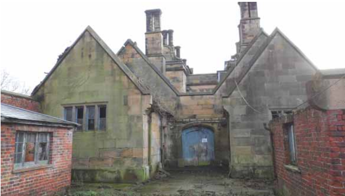
Figure 6: Rear ranges of the house, photograph taken from the north-west (Alison Arnold)
