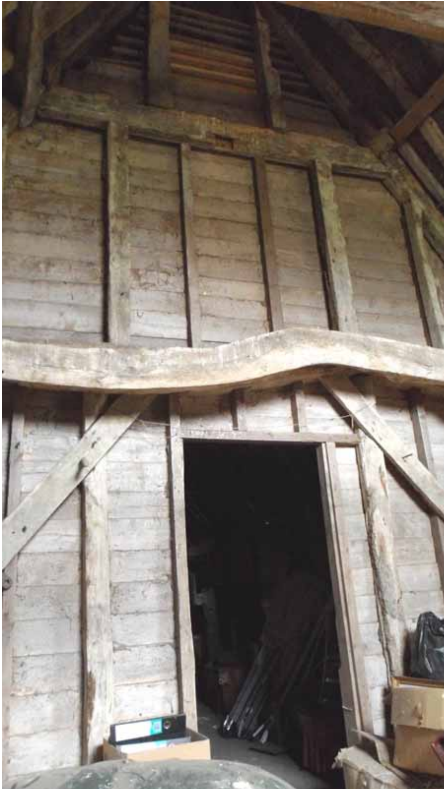
Figure 25: Truss 7 of the former stable block, with distinctive 'bend', taken from the south (Alison Arnold)
