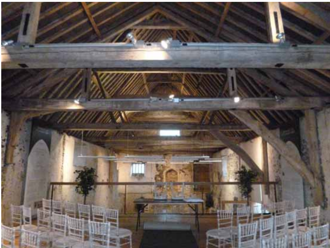
Figure 6: Former west range of the cloister, photograph taken from the south (Alison Arnold)
