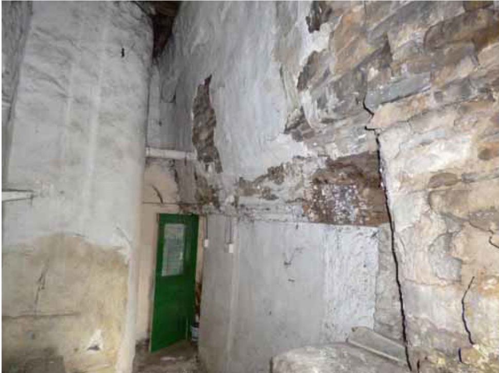
Figure 13: Service range, Kitchen, smokehood bressummer, photograph taken from the south-east (Robert Howard)
