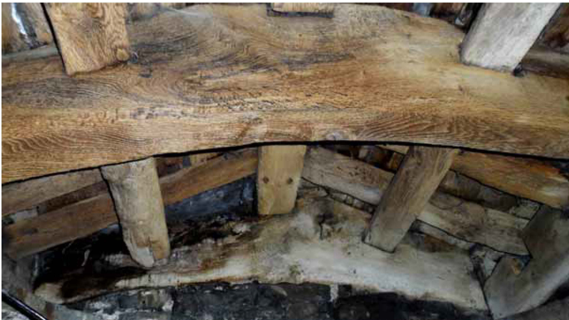
Figure 8: High-end tower, turret roof, truss 2 in foreground, photograph taken from the east (Robert Howard)
