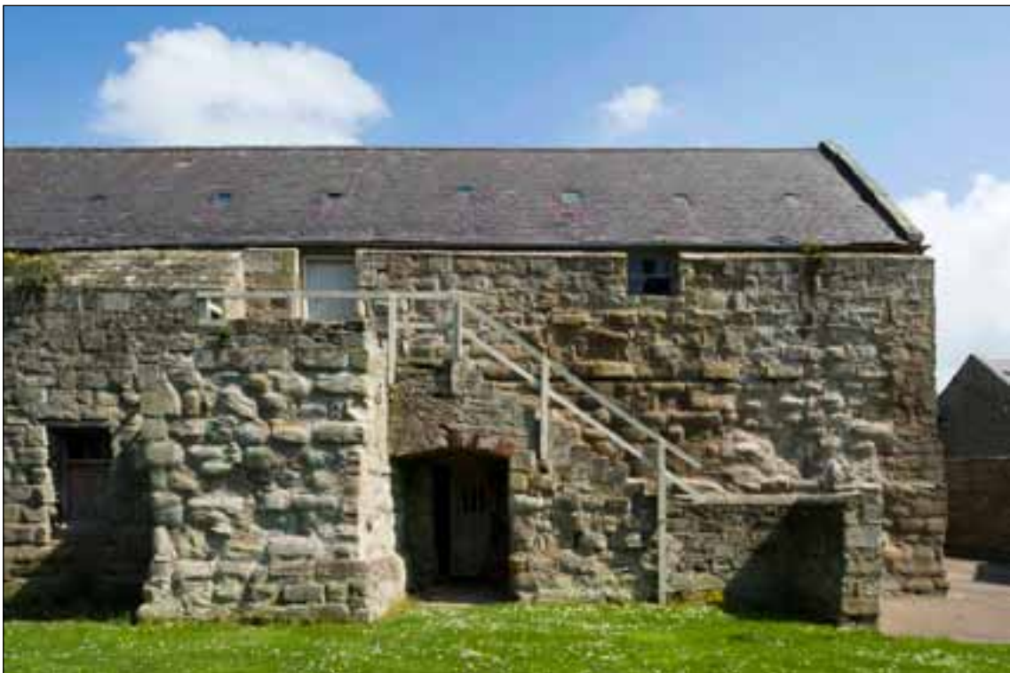
Figure 23: The steps against the south-west wall (DPI56890 © English Heritage, photograph: Alun Bull).
