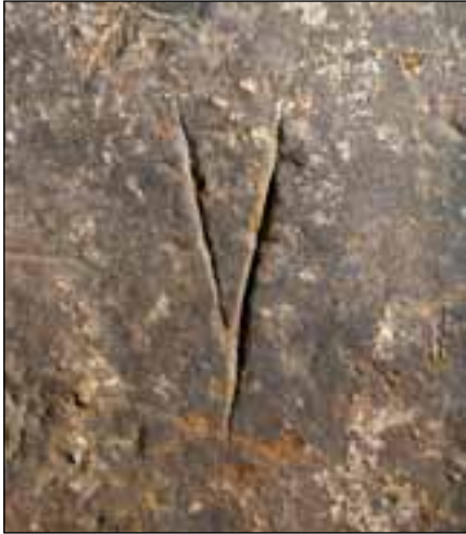
Figure 21: The Y-shaped, possible mason's mark above a recess in the interior south-west wall (DPI56889 © English Heritage, photograph: Alun Bull).
