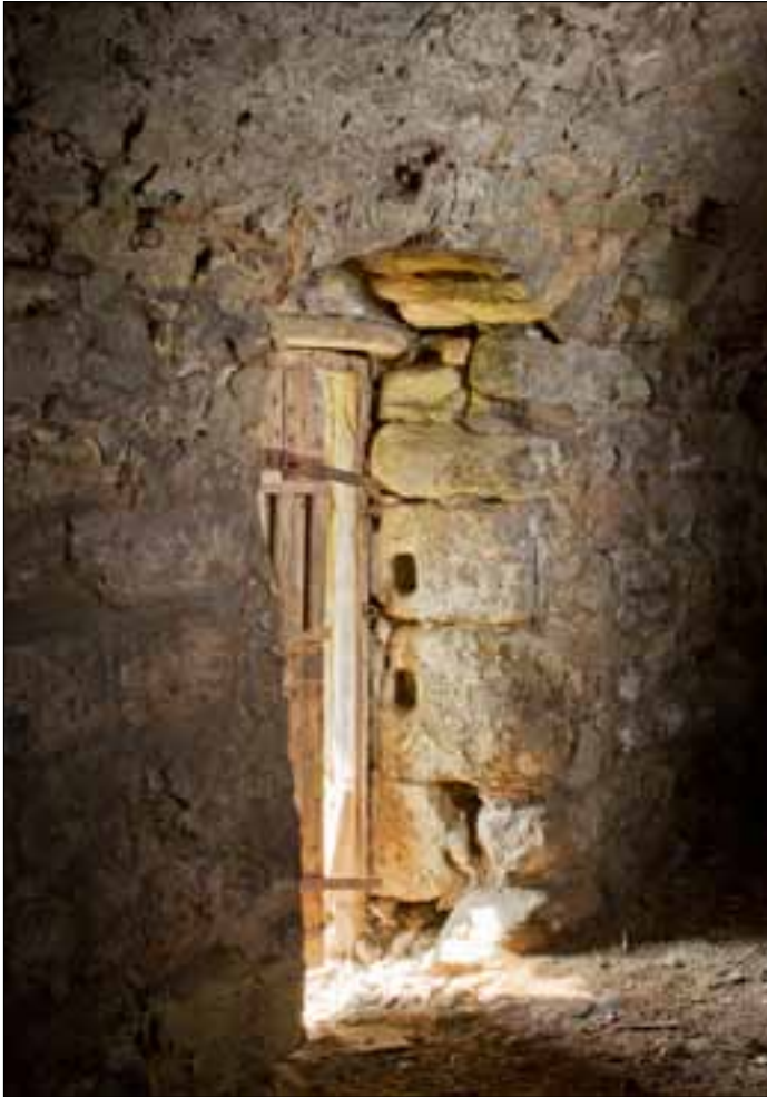
Figure 18: The doorway in the south-west wall including draw-bar holes (DPI56936 © English Heritage, photograph: Alun Bull).
