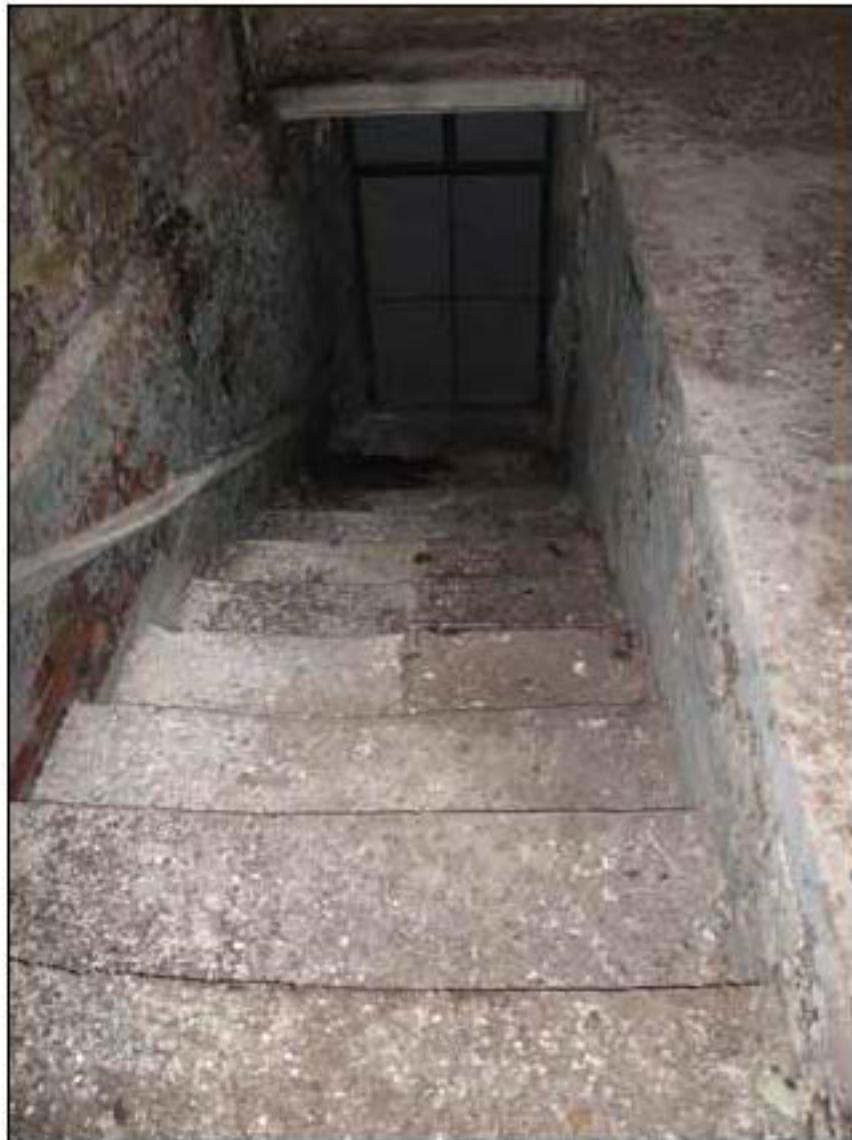
Figure 49. Stair access from engine house to the tunnel under Haslar Road (© English Heritage)
