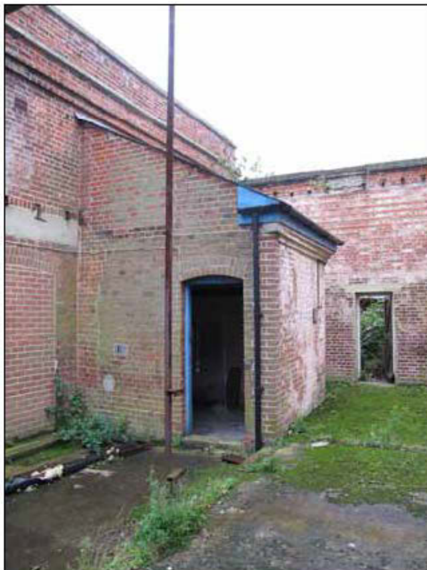
Figure 46. Modern well house, built on the site of an earlier well house which probably predates the 1854 construction of the engine house complex (© English Heritage)
