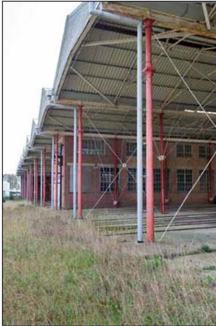
Figure 38. Columns at front of gunboat shed cast in two pieces and joined together. Ordinary cross-sectioned columns are visible behind these. (EHA DP161538)
