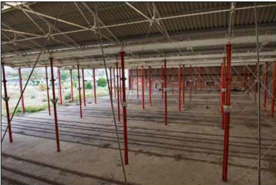
Figure 36. Gunboat shed interior from south showing the regular column spacing throughout the interior (EHA DP161553)
