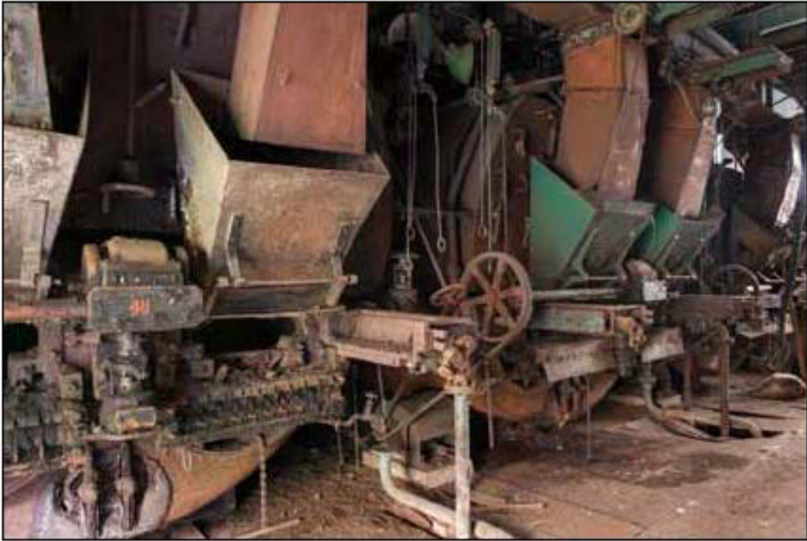
Figure 50. Lancashire boilers, with a later automated hopper system (EHA DP161559)
