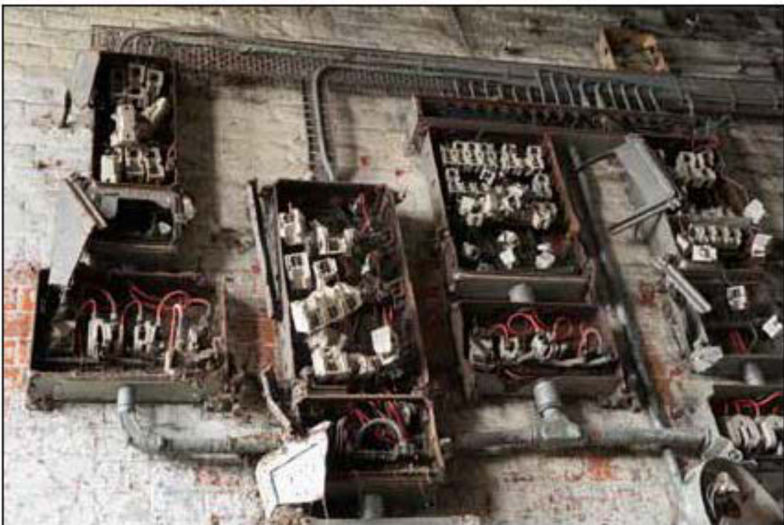
Figure 51. Fuseboxes on the west wall of the boiler house (EHA DP161563)
