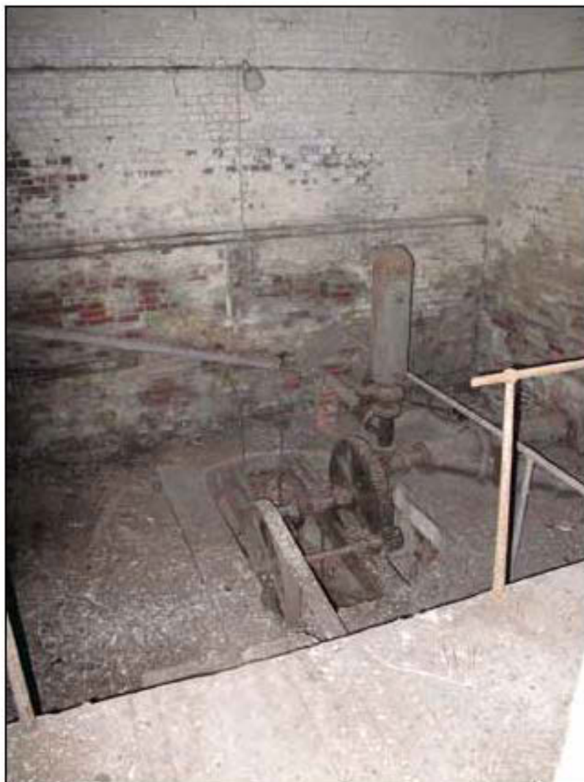
Figure 48. Interior of well house to the east of the engine house showing winch mechanism (© English Heritage)
