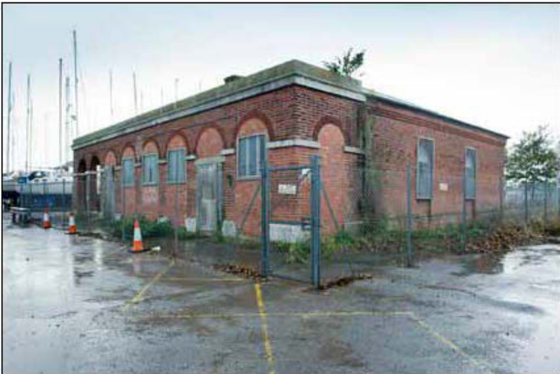
Figure 57. Former guard house to the north of the main entrance (EHA DP161570)
