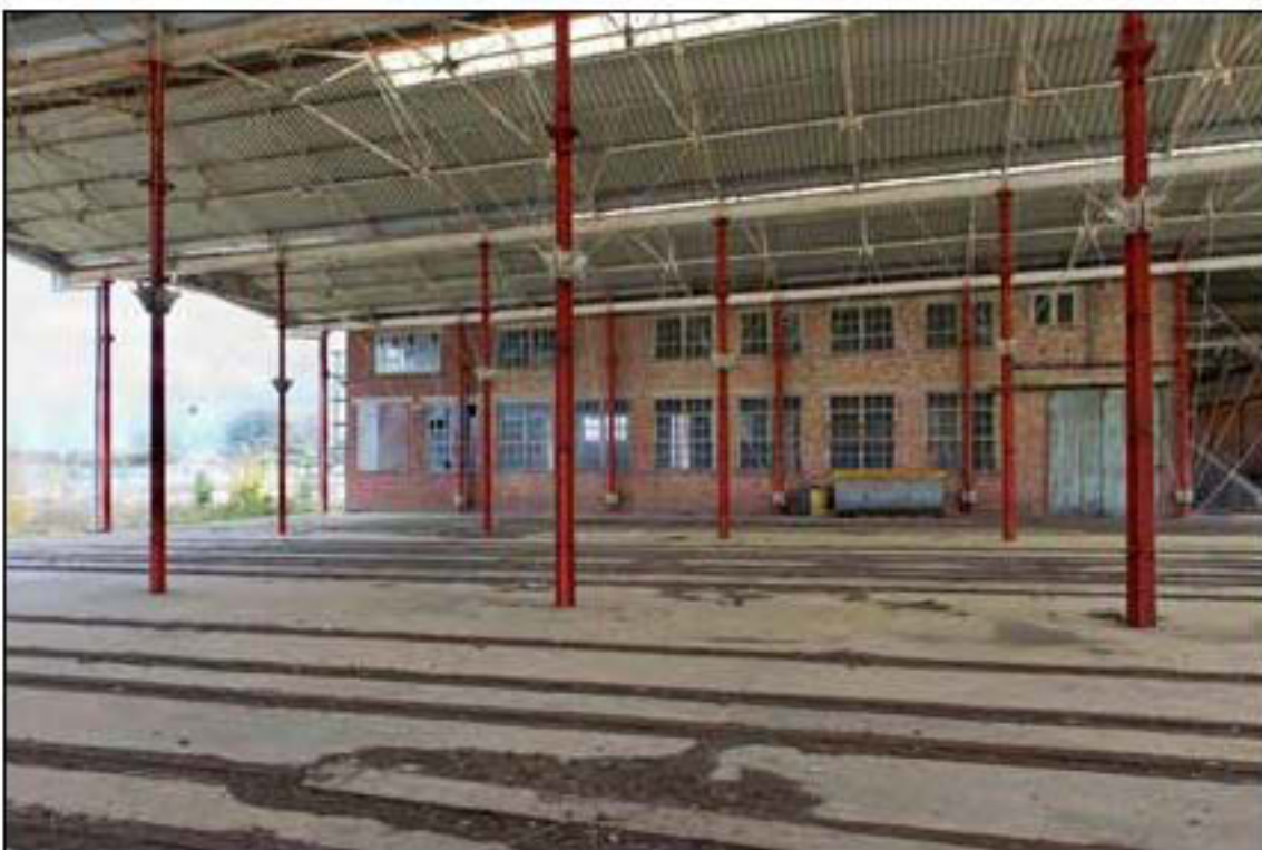
Figure 34. Interior of gunboat sheds showing the west elevation of the inserted brick building (EHA DP161558)
