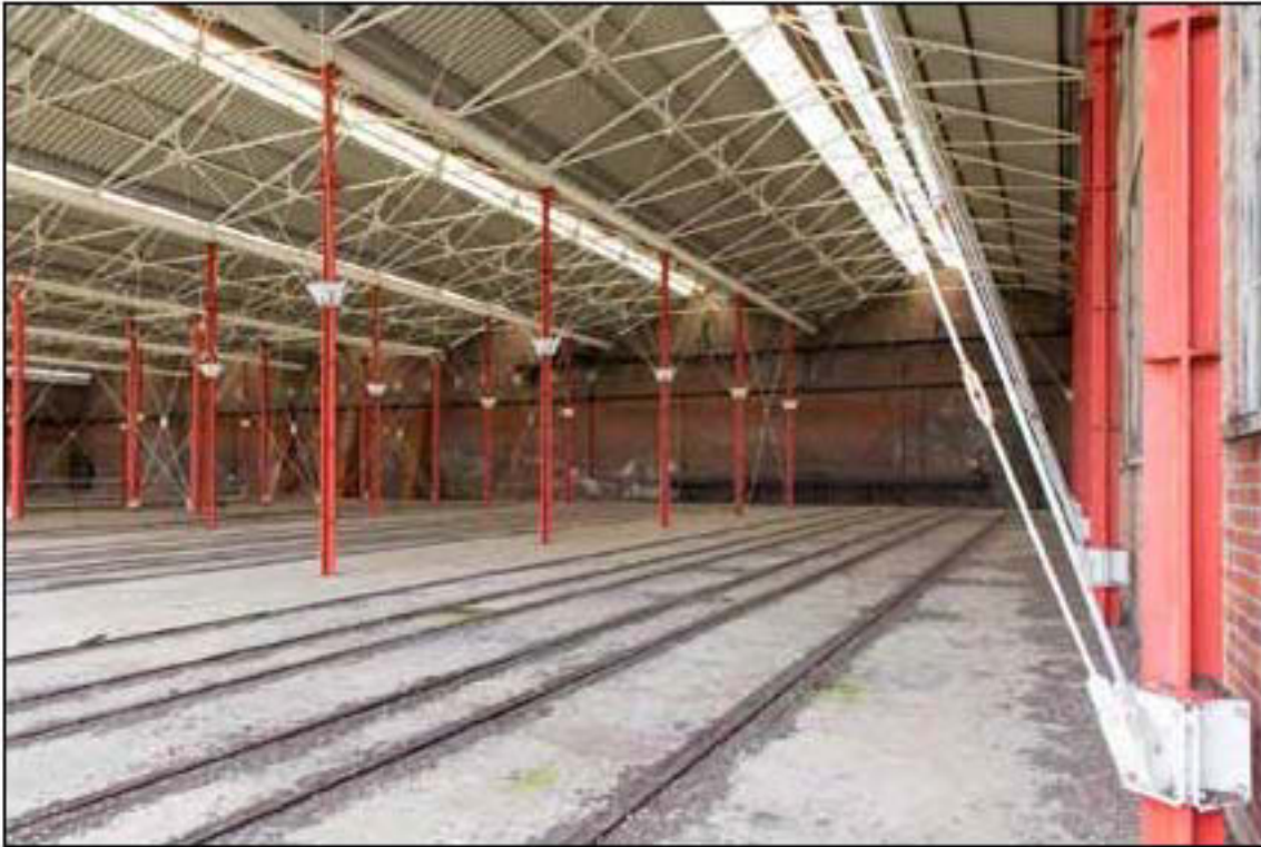
Figure 35. Gunboat shed interior from north west, showing the three sets of rails present in the standard bays (EHA DP161544)
