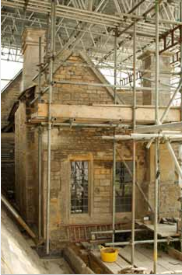
Fig 4. The 15th-century chimney stack on north side of former south lodging tower, seen on the side elevation, to the left. (DPI52835)
