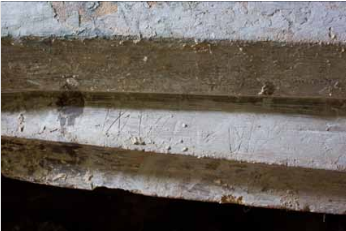
Fig 7. Graffiti or apotropaic marks on fireplace in S3.03. (DPI61399)
