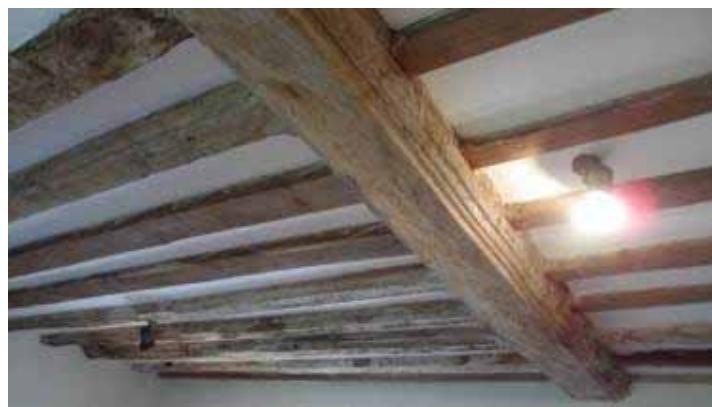
Figure 6a-c: Views of the clasped-purlin roof to the original part of the bothy (top), the roof to the extension (middle) and the ground-floor ceiling to the bothy extension (bottom) (photographs Robert Howard)
