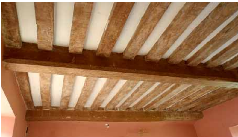
Figure 3a-c: Views of the hall range with its gatehouse (top), its roof (middle) and east-end ground-floor ceiling beams (bottom) (photographs Robert Howard)
