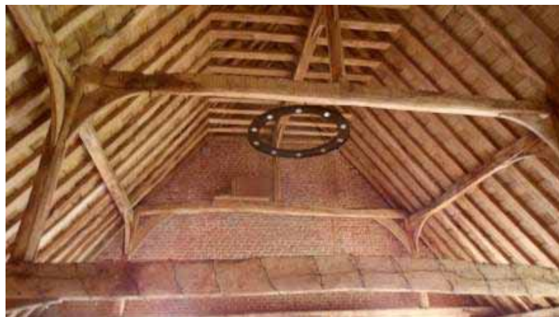
Figure 5a-c: Exterior view of the barn (top), its west-end roof (middle) and queen-post with crown-post roof trusses to easternmost four bays (bottom) (photographs Robert Howard)
