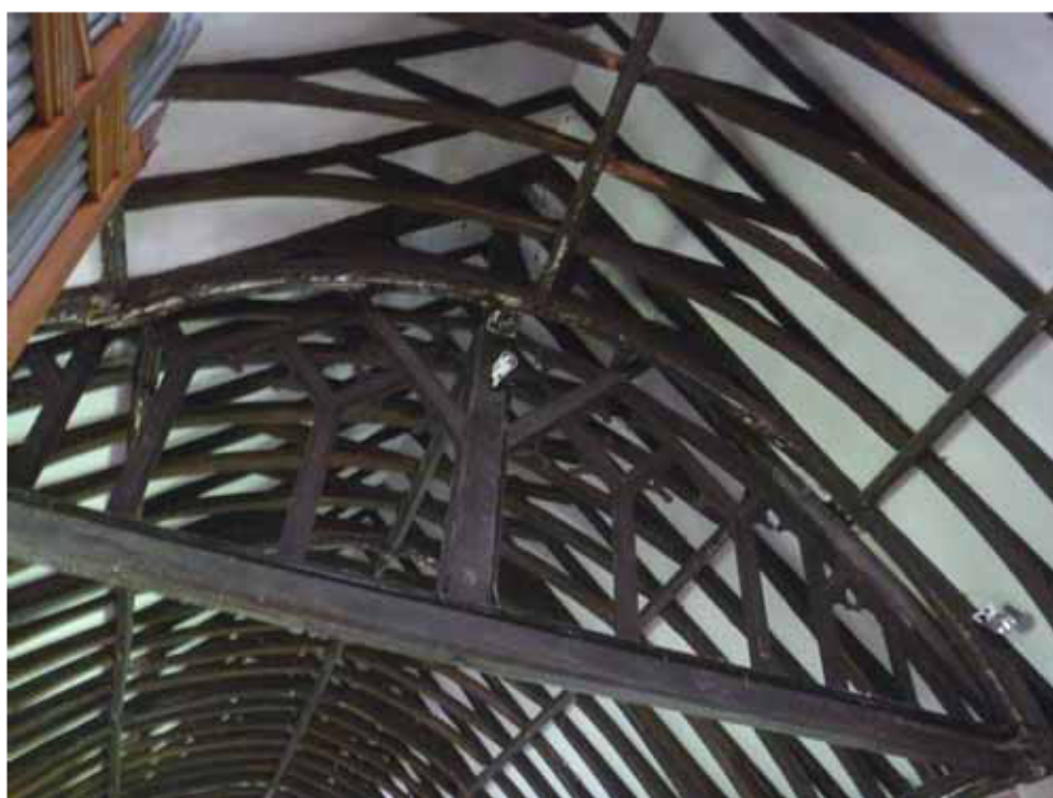
Figure 4a/b: View of the nave roof (top), looking west to east, and the screen truss at the junction of the nave and chancel roofs (bottom) (photographs Robert Howard)
