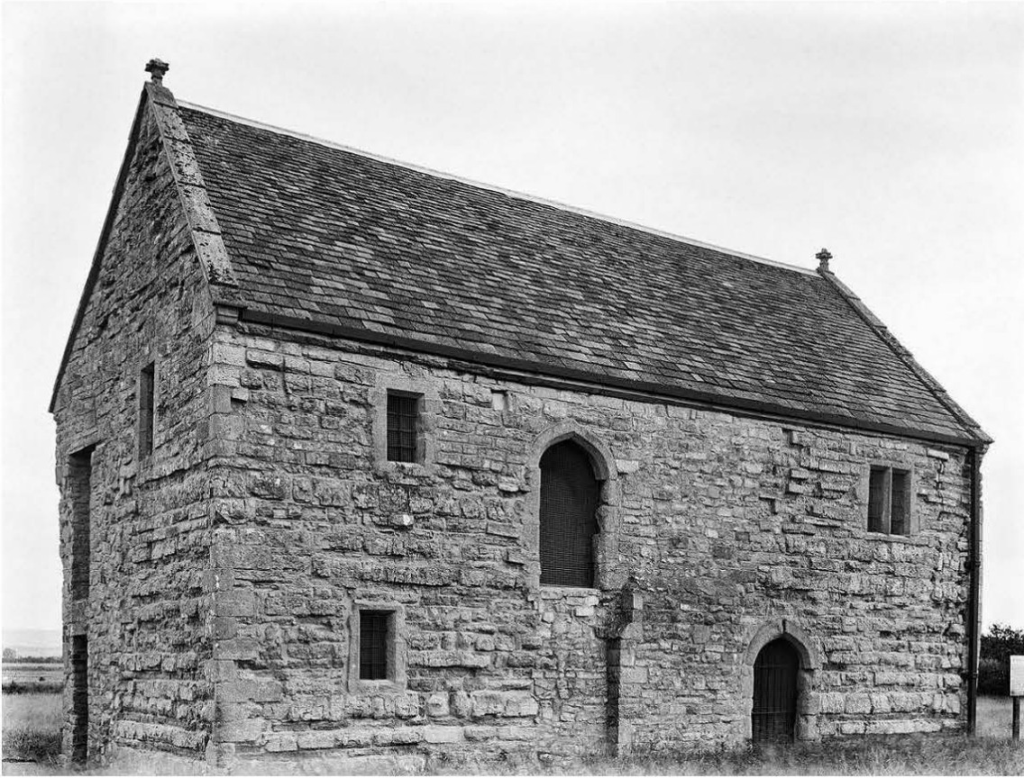
Figure 10: Meare Fish House. South Elevation 1924. Reproduced by permission of English Heritage. Reference Number: CC001334
