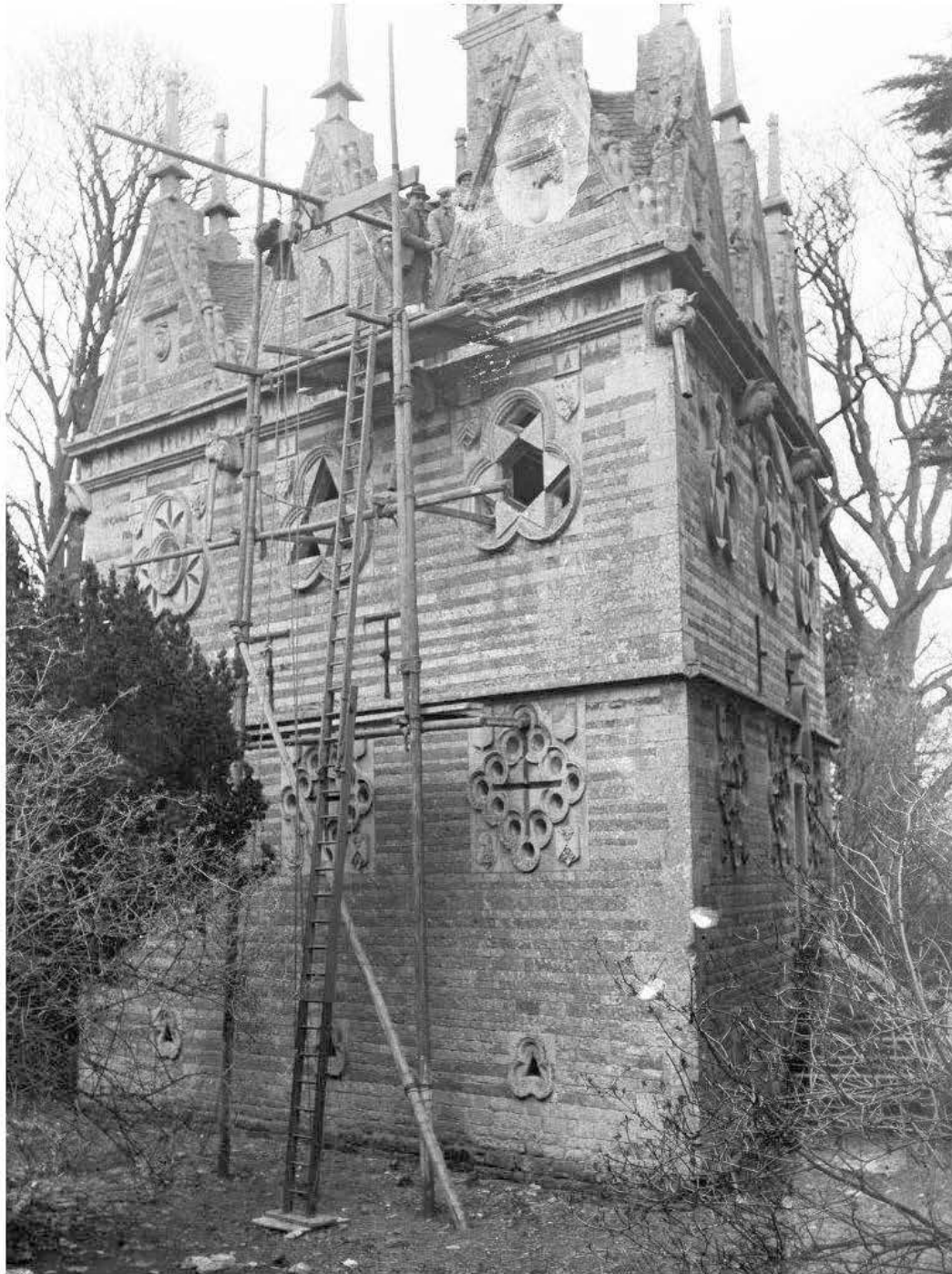
Fig 8: Rushton Triangular Lodge, Northamptonshire, in 1945, during emergency repairs carried out at the Ministry's expense. Reproduced by permission of English Heritage
