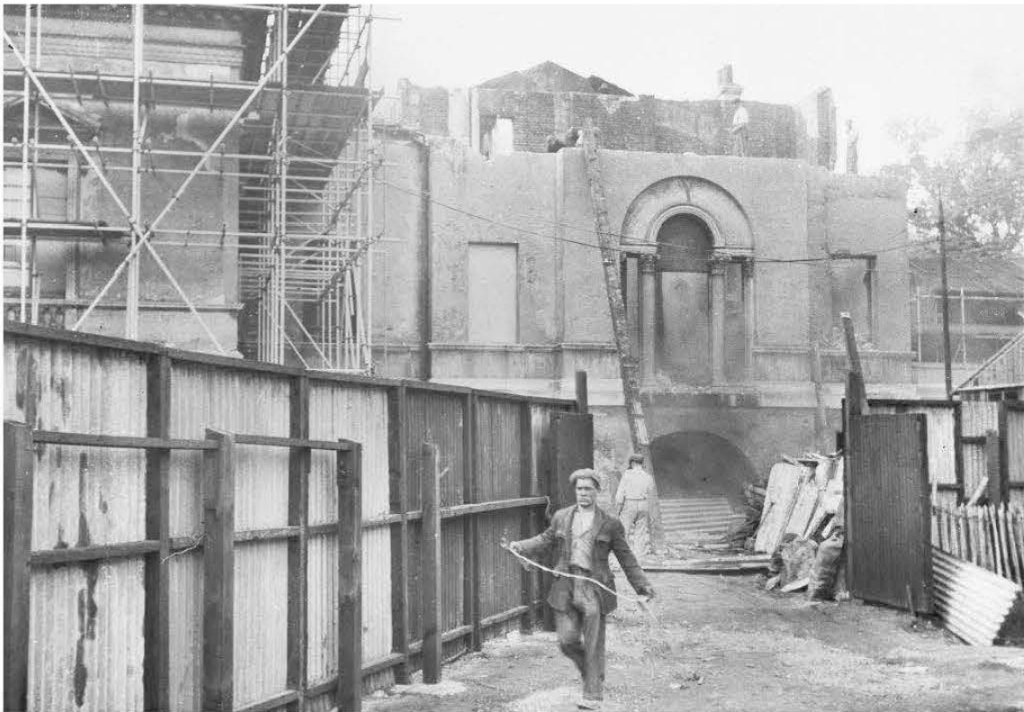
Fig 27: Demolition of the Wyatt wings at Chiswick House in progress, October 1950. Reproduced by permission of English Heritage
