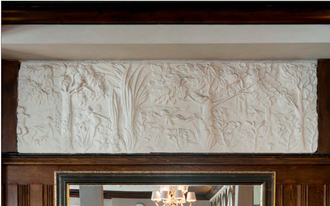
12.14.8 One of the elaborate plasterwork panels which are now located in the area of the former public bar. The panels were originally a feature of the saloon bar (see Fig. 12.14.4). (© Historic England, Derek Kendall, DPI70043)
