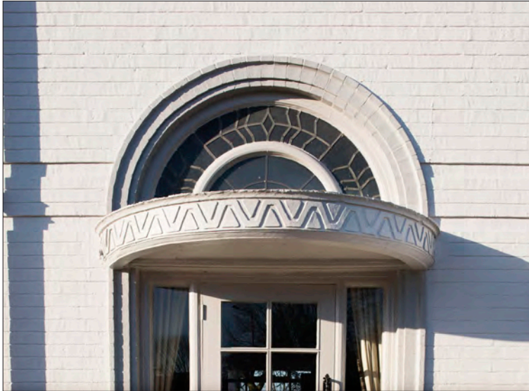
12.13.2 A detail of the Court Oak's main elevation, showing the canopied entrance to one of the side bars. (© Historic England, James O. Davies, DPI66396)
