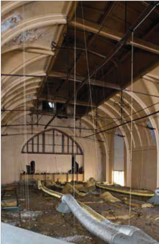
Fig 13 Roof structure and suspended false ceiling of the great hall. © Pat Payne, English Heritage, DPI61079
