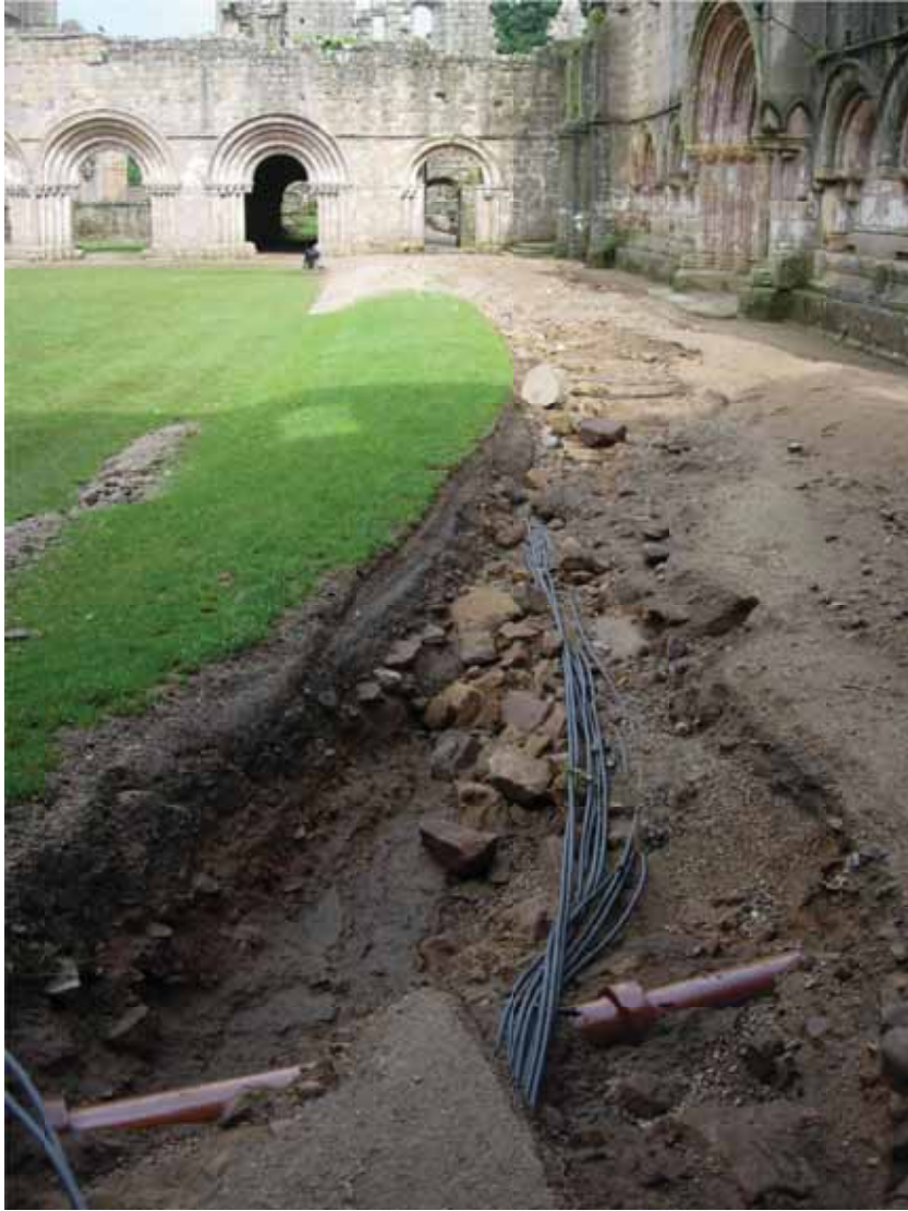
Erosion gullies at Fountains Abbey after the 2007 flood (Neil Redfern)
