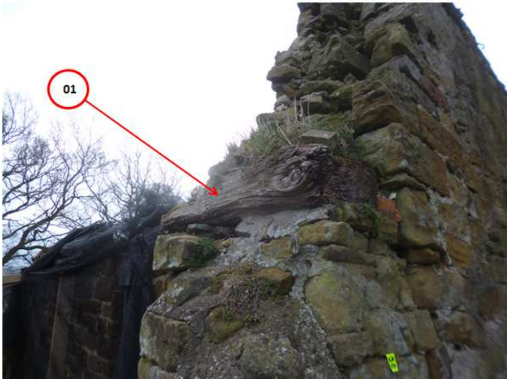
Figure 4a: View to help locate sampled timber - north wall, outer face (photograph Robert Howard)
