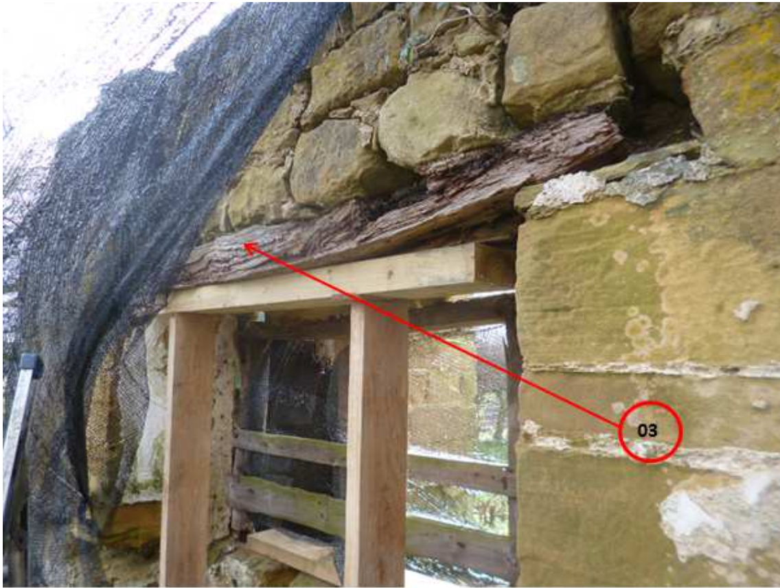
Figure 4c: View to help locate sampled timber - south wall, inner face (photograph Robert Howard)
