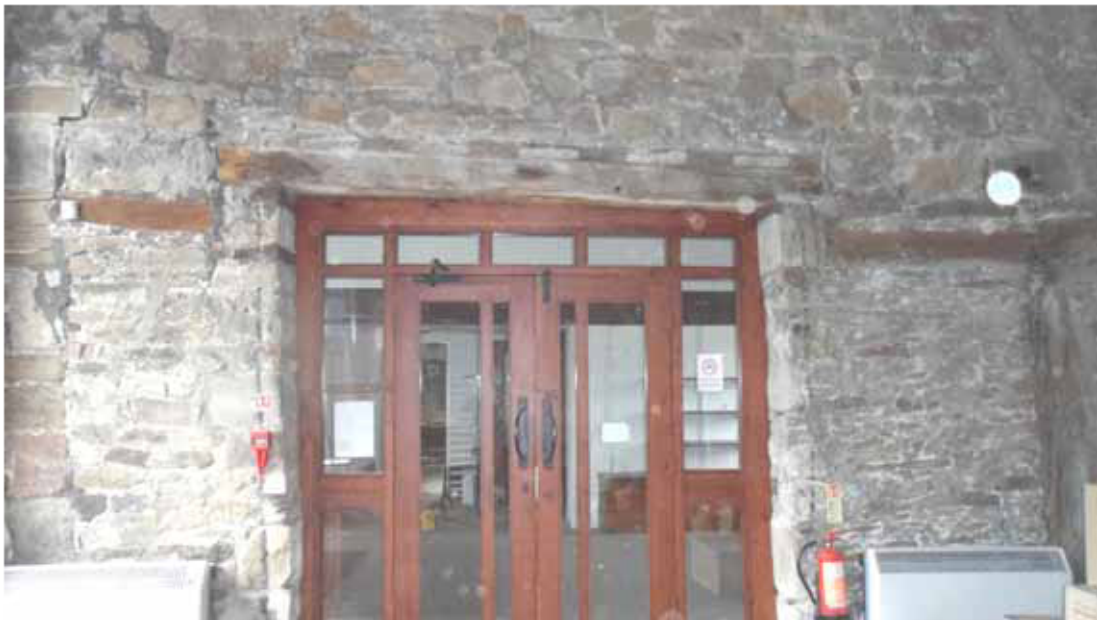
Figure 14: Partition between carriage house and lobby, photograph taken from the carriage house (Alison Arnold)
