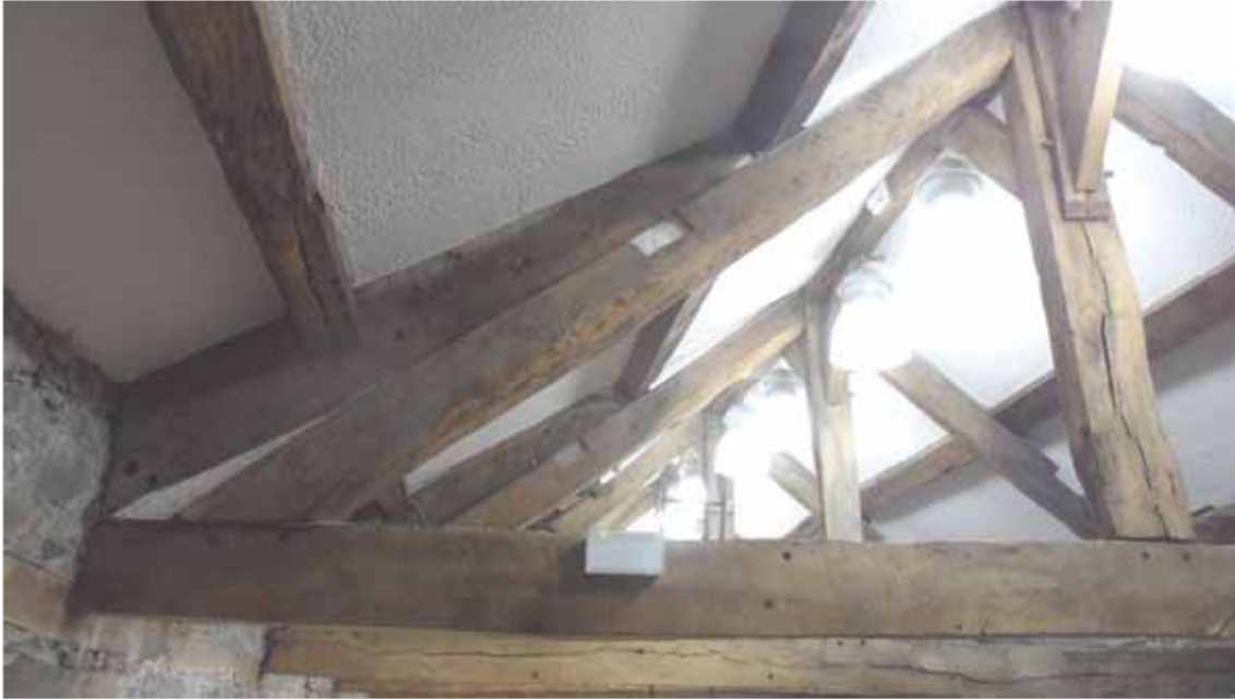
Figure 9: Stables, one of the backing rafters used to modify roof pitch, photograph taken from the west (Alison Arnold)
