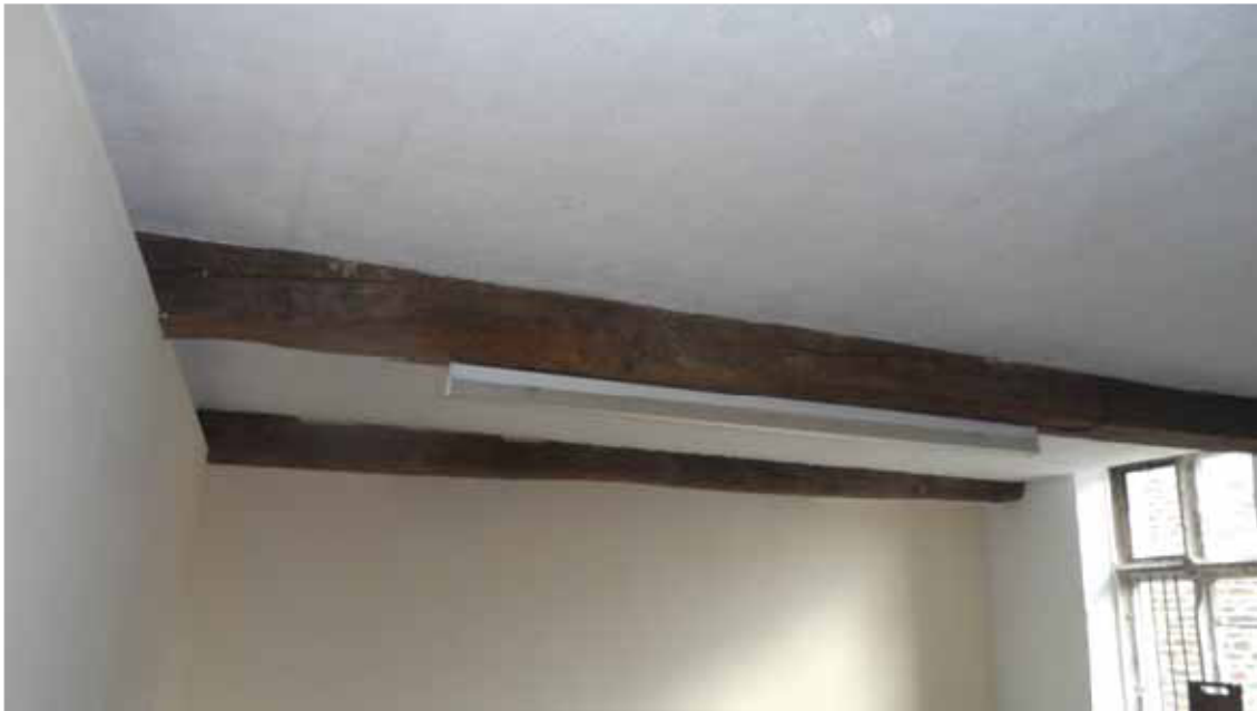
Figure 10: Stables, ground-floor ceiling beams (beam 2 in the foreground), photograph taken from the north-west (Alison Arnold)
