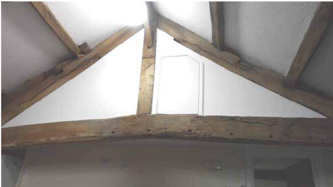
Figure 8: Stables; truss 4 with canted tiebeam, photograph taken from the west (Alison Arnold)
