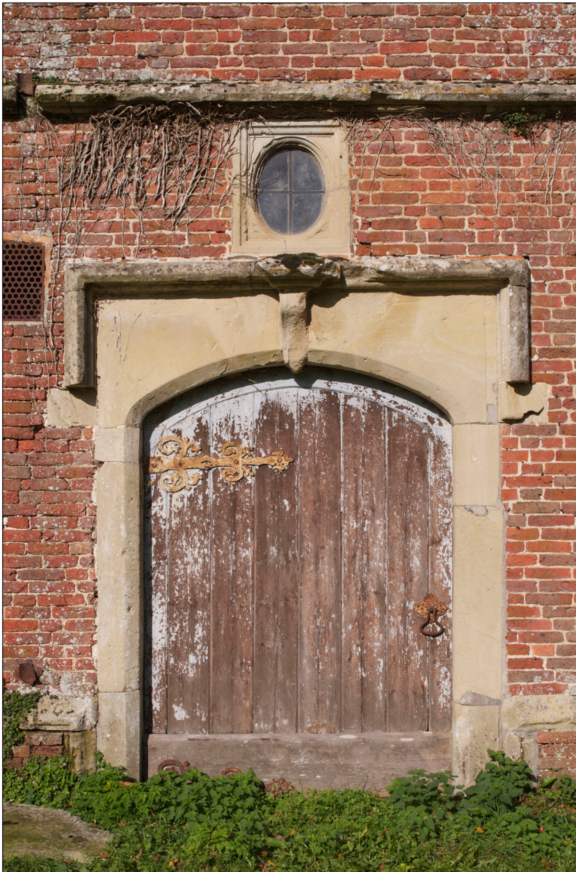
Figure 6: Relocated doorway on the south elevation (DP136166 © Historic England, photograph: James O. Davies).
