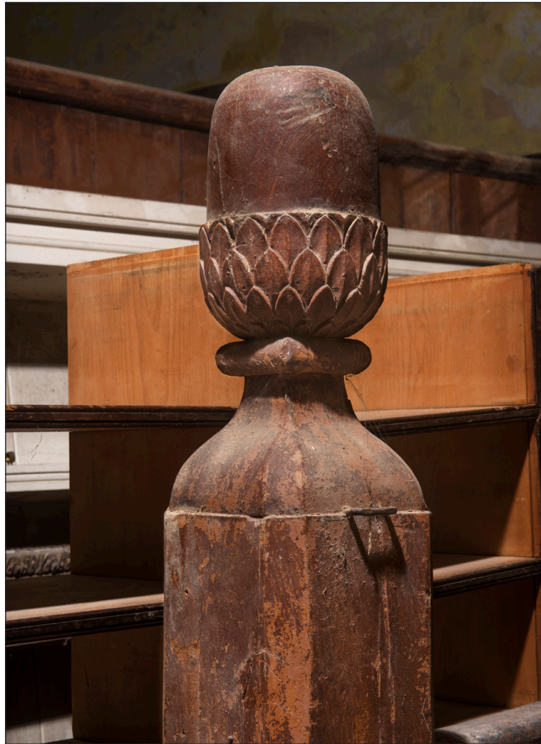
Figure 30: Detail of one of the acorn finials in the east stable (DP166183 © Historic England, photograph: James O. Davies).
