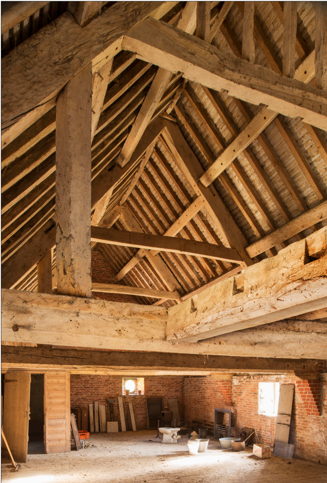
Figure 25: Roof structure looking southeast showing original spine beam (DP166163 © Historic England, photograph: James O. Davies).
