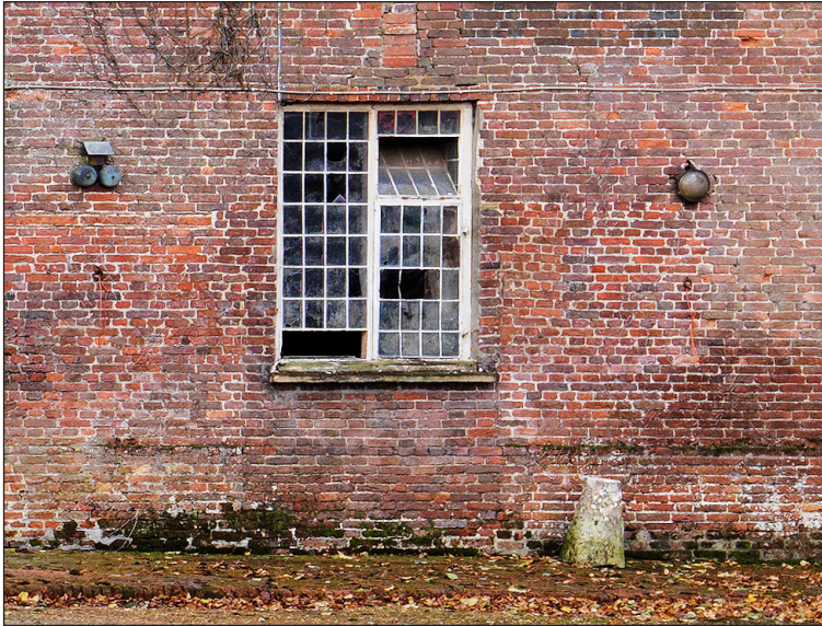
Figure 27: Detail of one of four 18th century windows inserted into the north elevation (DP166142 crop © Historic England, photograph: James O. Davies).
