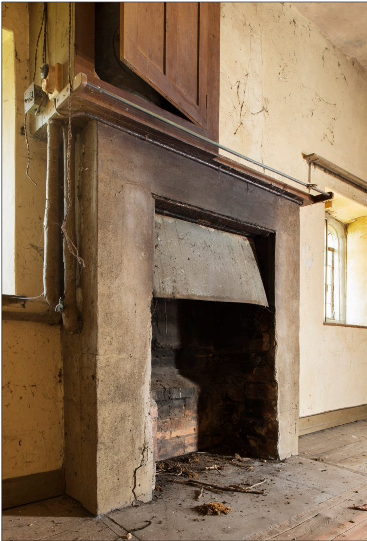
Figure 31: Detail of the fireplace in the 1st floor western room (DP166170 © Historic England, photograph: James O. Davies).
