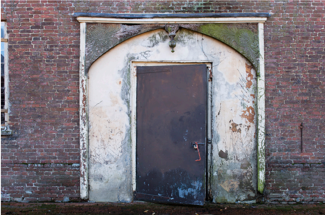
Figure 33: Detail of door surround to east stable door (DP166146 © Historic England, photograph: James O. Davies).
