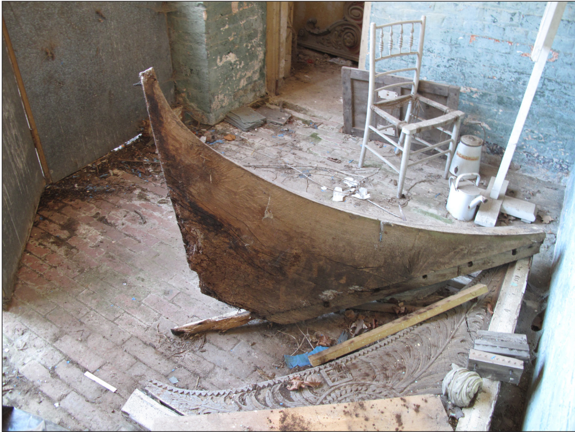
Figure 38: Rear of spandrel currently located inside the lobby of the Grooms' House, showing tenon with peg holes along the long side of the timber (© Historic England, photograph: Rebecca Lane).
