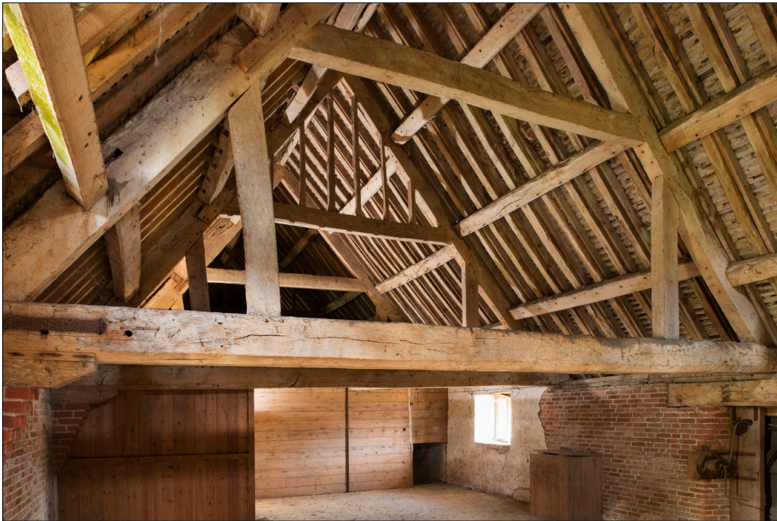
Figure 26: Roof structure looking northwest showing partition timbers above the collar of the central truss (DP166163 © Historic England, photograph: James O. Davies).
