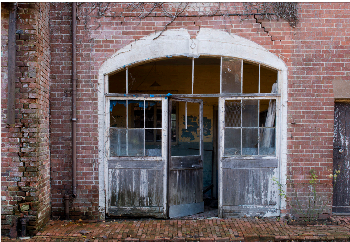
Figure 37: Former position of spandrels over doorway on the Grooms' House (DP166145 © Historic England, photograph: James O. Davies).
