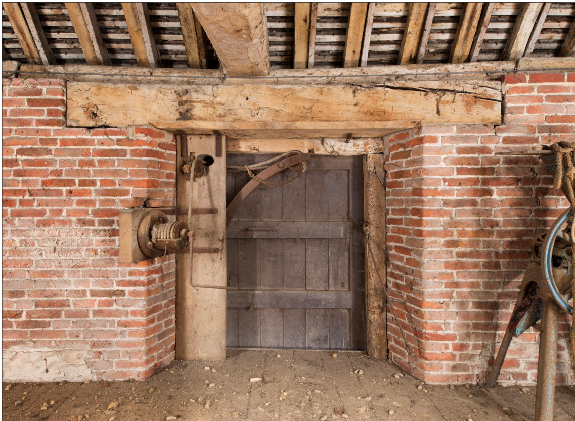
Figure 20: The original taking-in door in the north elevation (DP166168 © Historic England, photograph: James O. Davies).
