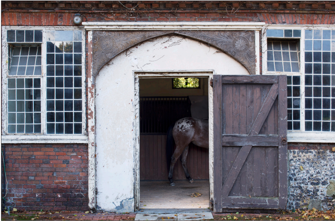
Figure 36: Detail of spandrels over the stable doorway on the western range (DP166149 © Historic England, photograph: James O. Davies).
