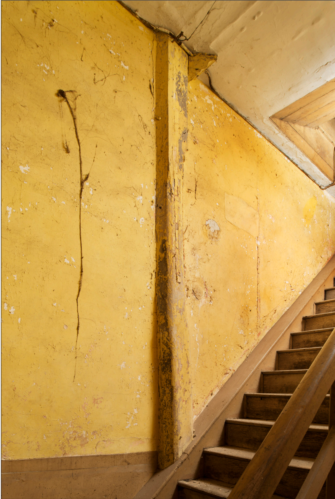
Figure 13: Stable arcade post surviving in the wall between the east stable and the stair (DP166162 © Historic England, photograph: James O. Davies).
