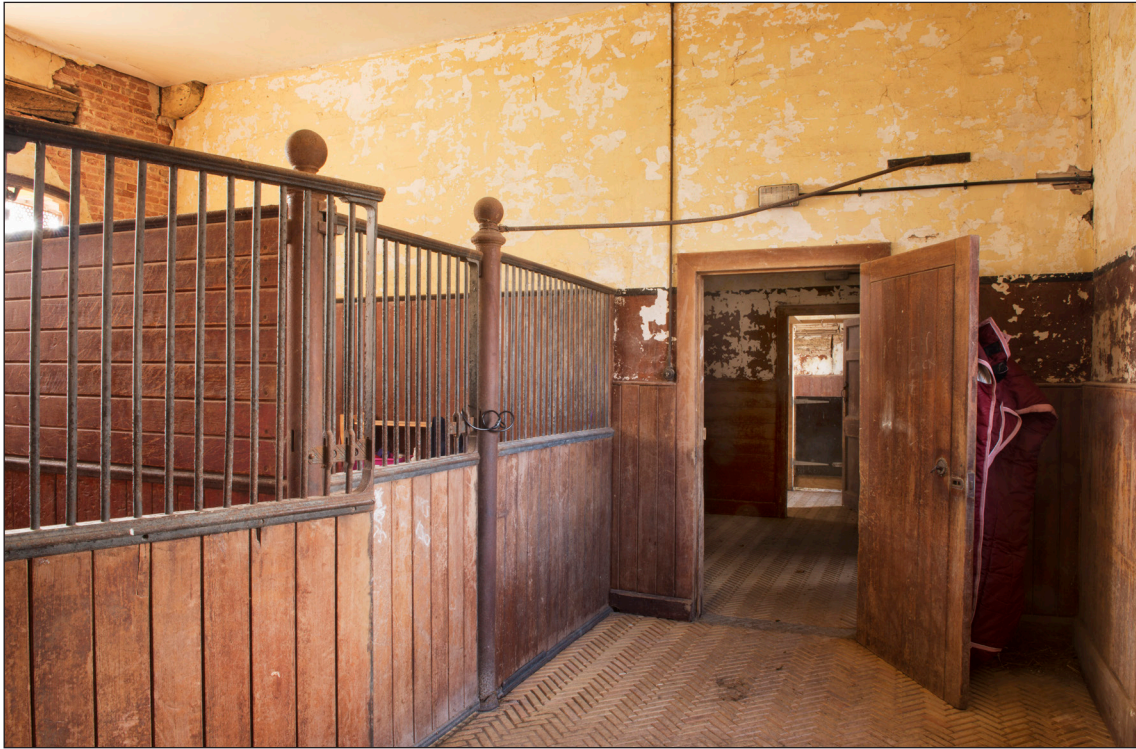
Figure 35: Detail of late 19th or early 20th century stabling in the central stable area (DP166188 © Historic England, photograph: James O. Davies).
