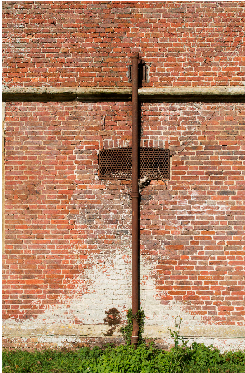
Figure 7: Original position of the south doorway, as indicated by disruption in brickwork and queen closers to the west (DP166174 © Historic England, photograph: James O. Davies).
