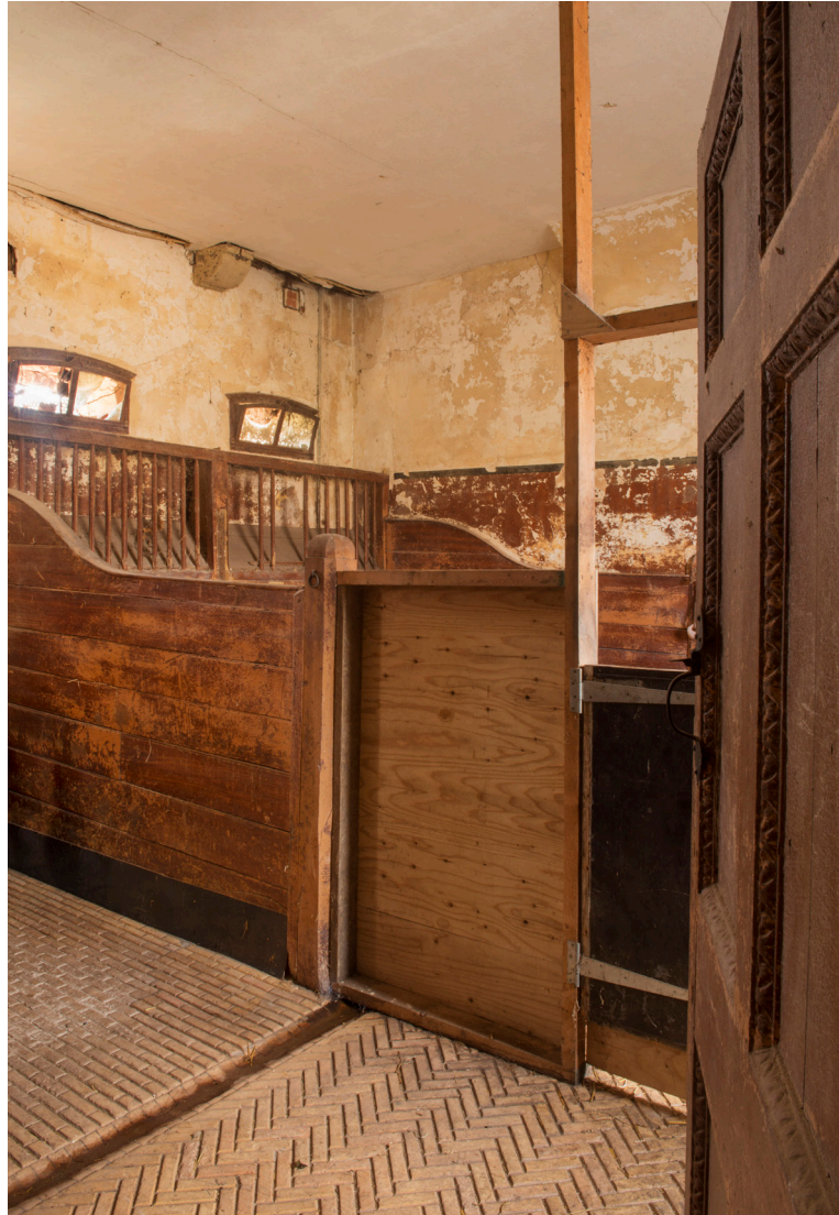
Figure 32: Detail of 19th century stalls in the western stable area (DP166190 © Historic England, photograph: James O. Davies).
