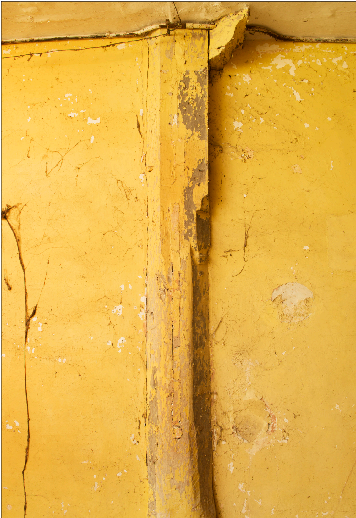
Figure 15: Detail of the side of the post, showing the infilled mortice measuring 0.99m in height (DP166161 © Historic England, photograph: James O. Davies).
