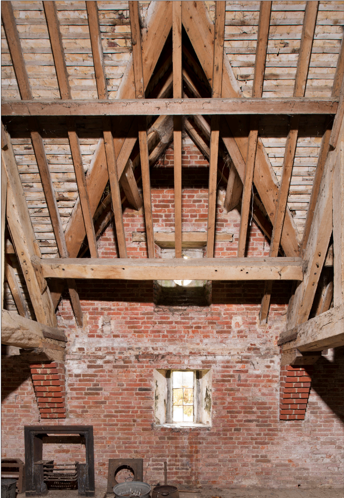
Figure 22: Interior of the eastern gable end showing the original high level opening with its timber lintel, and the inserted window opening below (DP166166 © Historic England, photograph: James O. Davies).
