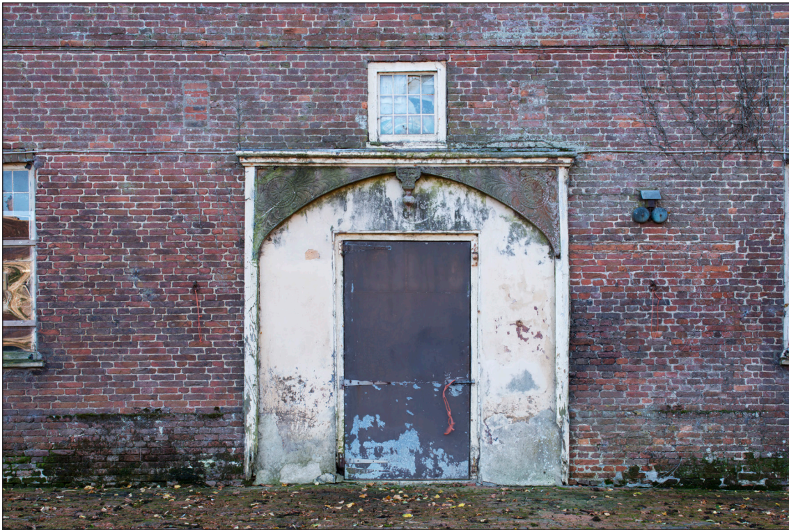
Figure 34: Detail of door surround to west stable door (DP166148 © Historic England, photograph: James O. Davies).
