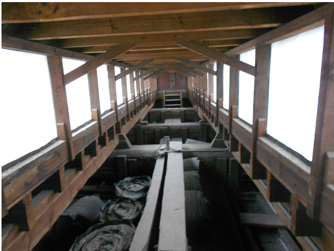
Figure 3: View looking south showing three of the four large pine beams over the Hall (Martin Bridge)
