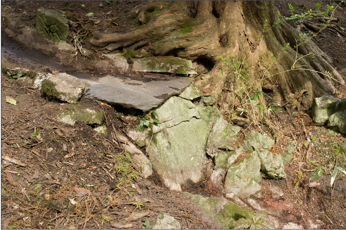
Figure 20: Detail showing the slate overhang within the channel of Farrer's 'stream' (note how the expanding roots and trunk of the adjacent yew tree are starting to push up beneath the concrete and stone). DP168981 © Historic England/Alun Bull, 28th April 2015.
