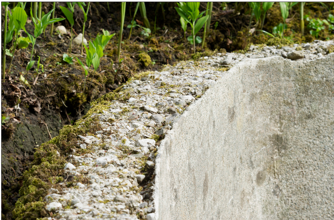
Figure 24: Detail showing the composition of the concrete wall of the pond island. DP168965 © Historic England/Alun Bull, 28th April 2015.
