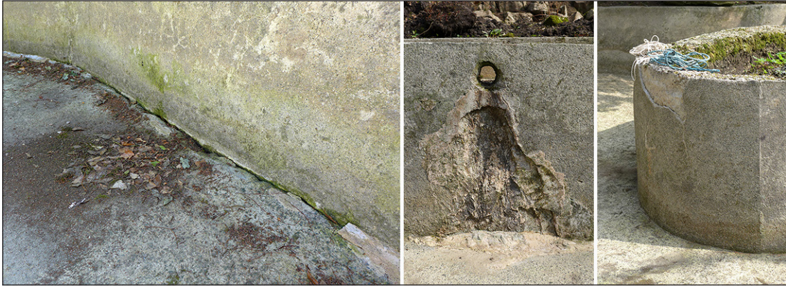
Figure 22: Details showing the deterioration of the concrete pond: (left to right) cracks forming between the wall and the base, with remnants of the unsuccessful mortar repairs; wall surface damage beneath the south example of two drainage holes between the bog garden and the pond; patches where render has flaked off the wall surface of the north end of the pond's central island. © Historic England/Rebecca Pullen, 9th May 2015.
