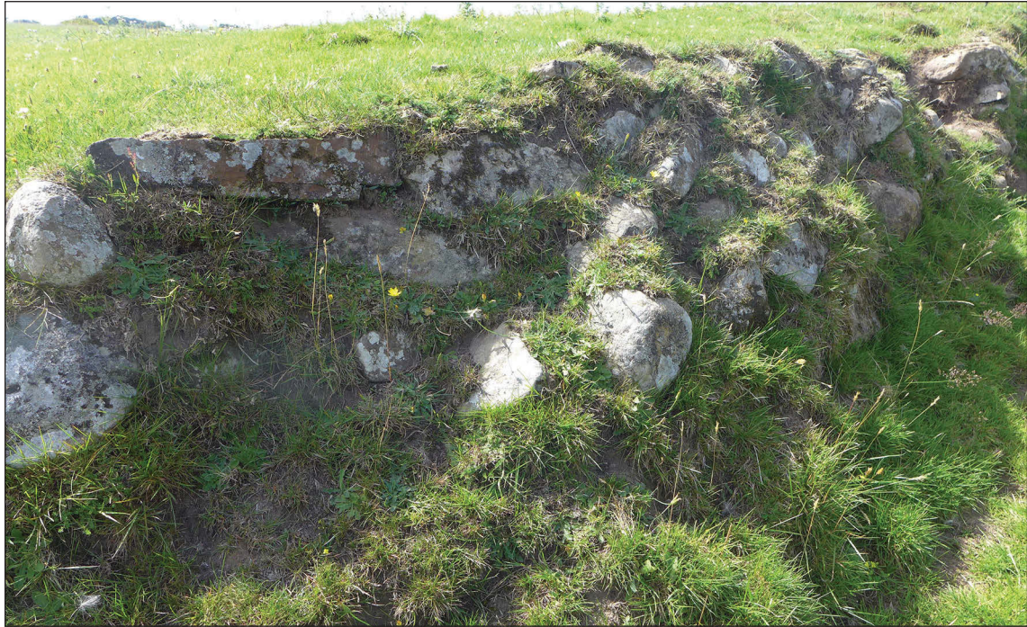
Figure 19. The revetment running below edge of the slope which separates the agricultural plateau from the bastle below, 12 August 2015. © Historic England / Rebecca Pullen.
