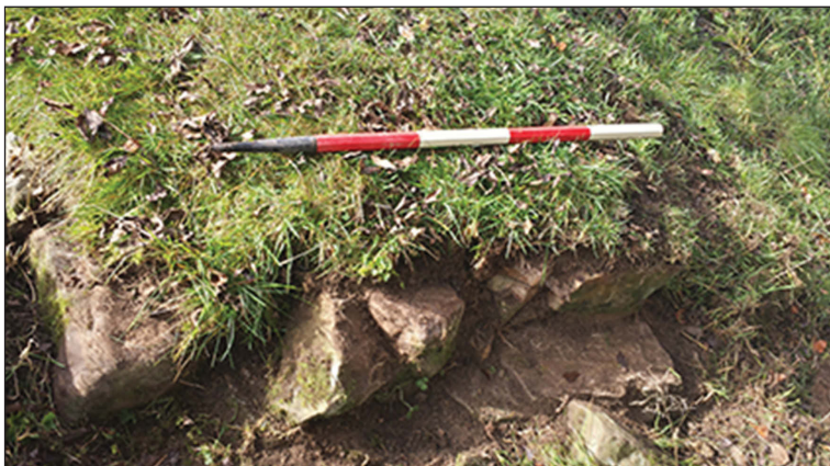
Figure 16. The north-east facing side of the possible entrance showing damage to the stonework. © Historic England / Cara Pearce
