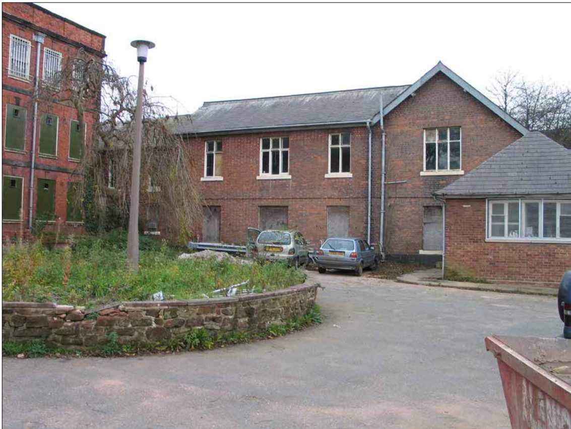
Figure 43: Range along Souter's Lane from the east (© Historic England, photograph: Adam Menuge).
