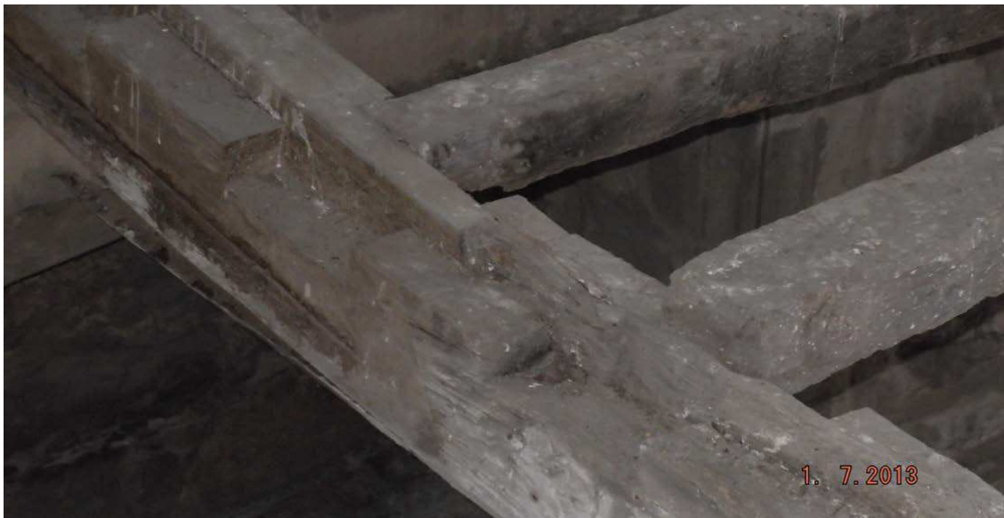
Figure 2e: Photograph of the second floor floor beam replaced in 2015 (Derrick Hodgson, English Heritage 2014)
