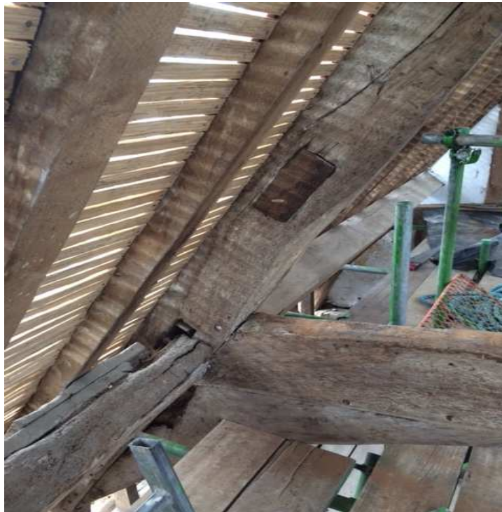
Figure 5: Photograph to show one of the blocked mortices which presumably once housed another purlin and the ill-fitting surviving purlin, photograph taken from the north-east (Alison Arnold)
