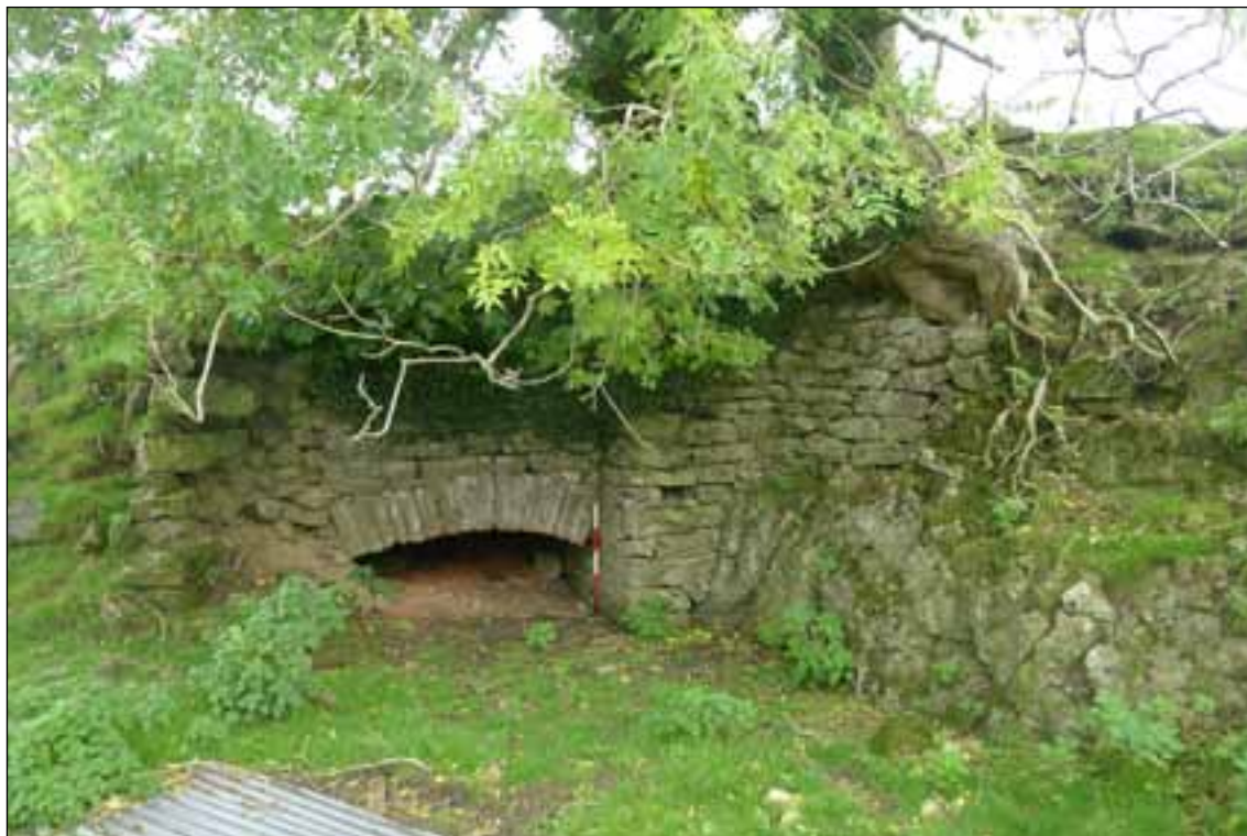
Figure 14: The small single pot lime kiln (36) included in the scheduled monument at Ashnott. Photo: Rebecca Pullen, © English Heritage.
