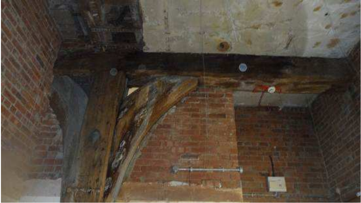
Figure 4a: View of the support timbers to the undercroft of the Keep (photograph Robert Howard)
