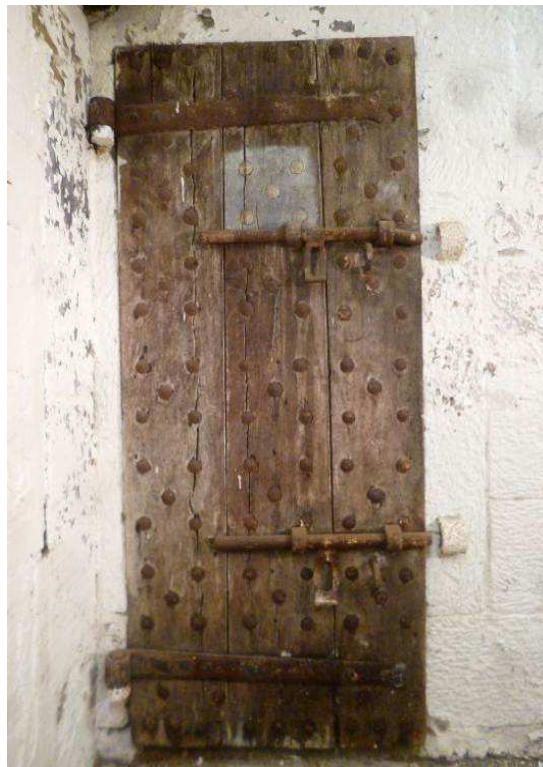
Figures 4b and 4c: Views of the doors to the solitary confinement cells in the undercroft of the Keep (photographs Robert Howard)
