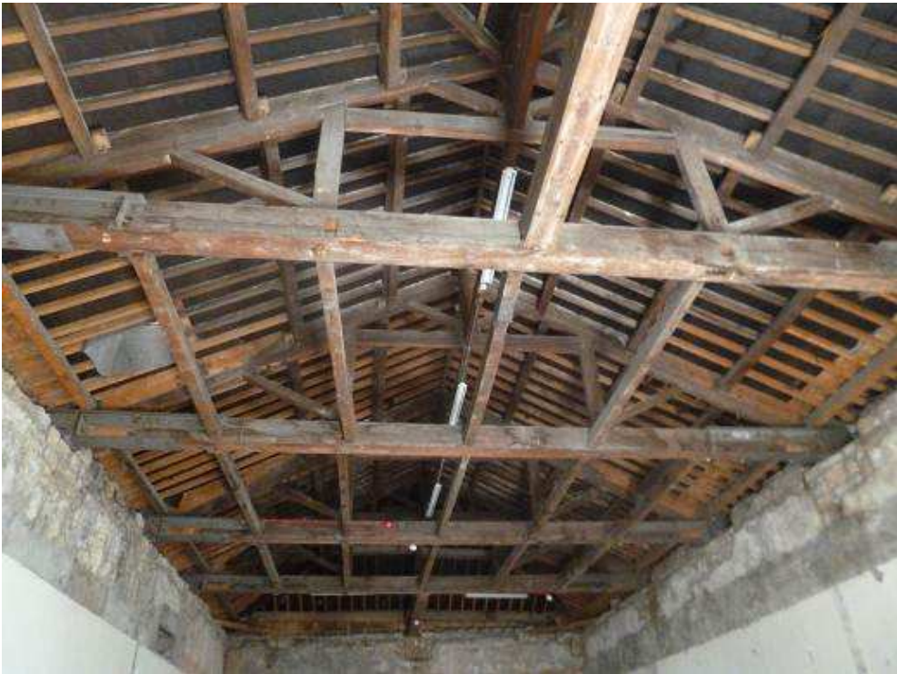
Figures 4d and 4e: Views of the timbers later inserted into the Great Hall of the Keep (top) and its later pine roof (bottom) (photographs Robert Howard)
