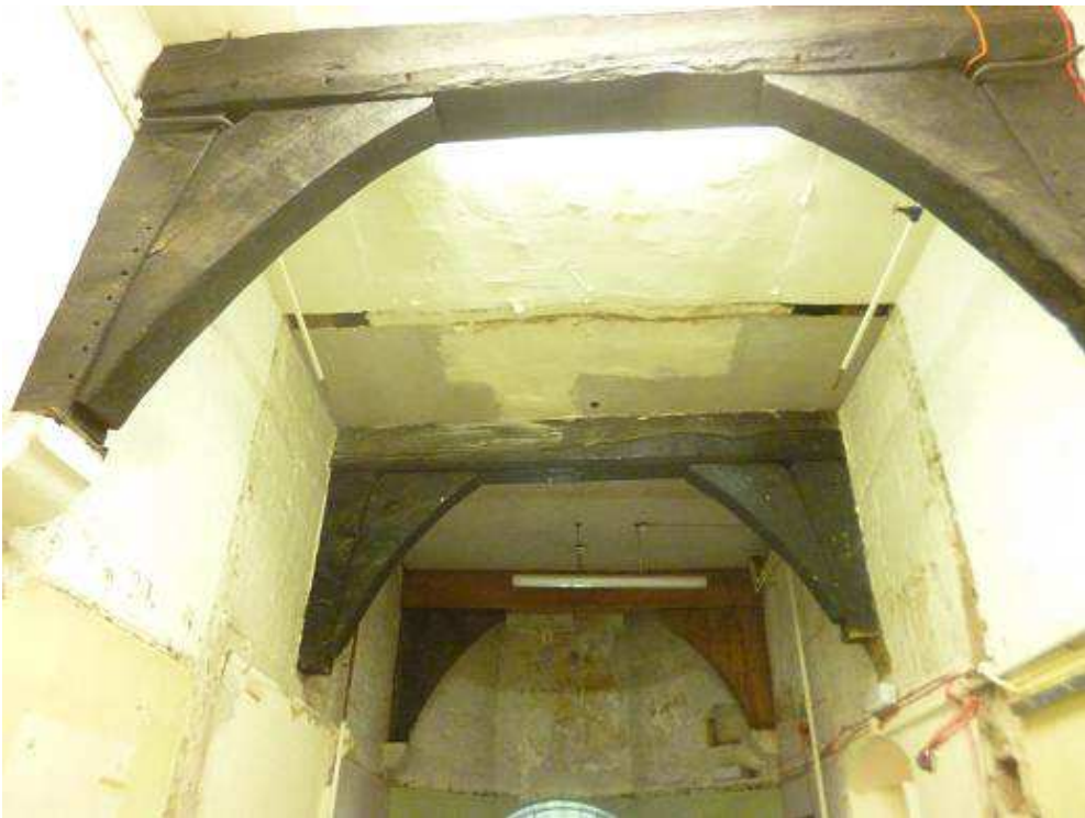
Figures 4f and 4g: View of second floor timbers to the Gatehouse (top) and those to the first floor (bottom) (photographs Robert Howard)
