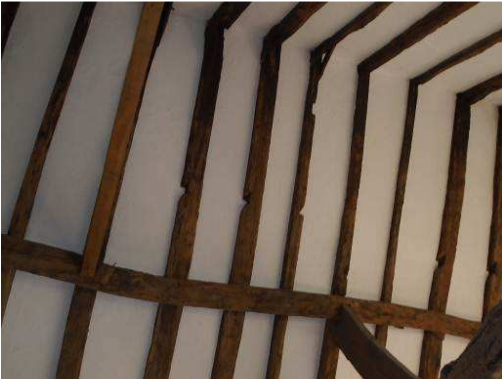
Figure 3a–b: Views of the timber framing to the north-south barn (photographs Robert Howard)
