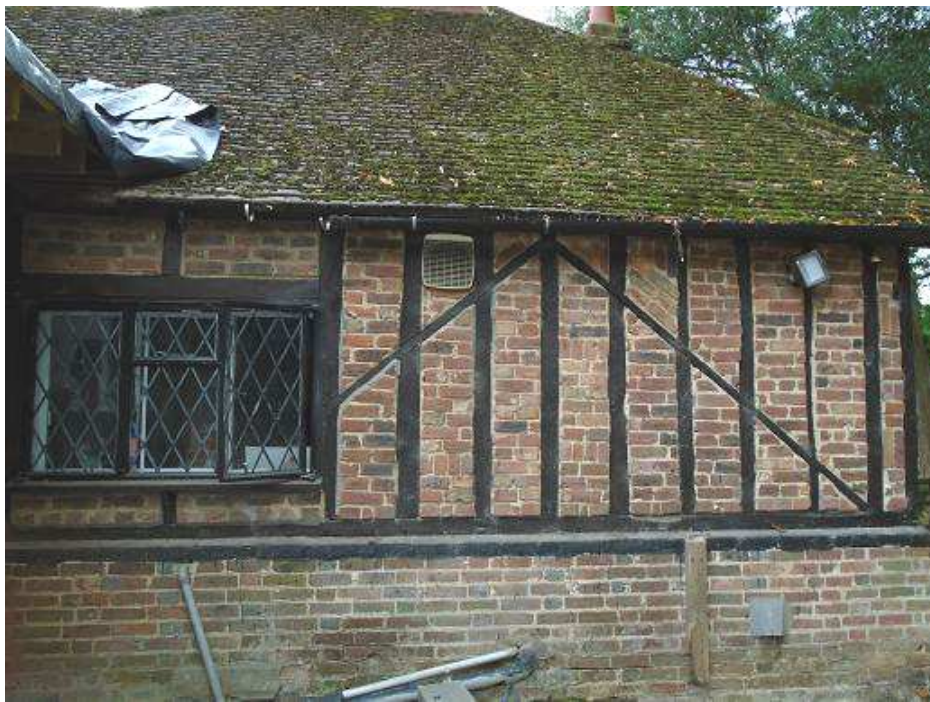
Figure 3c–d: Views of the framing to the west wall of the north-south barn (top) and the north wall of the later extension (bottom) (photographs Robert Howard)
