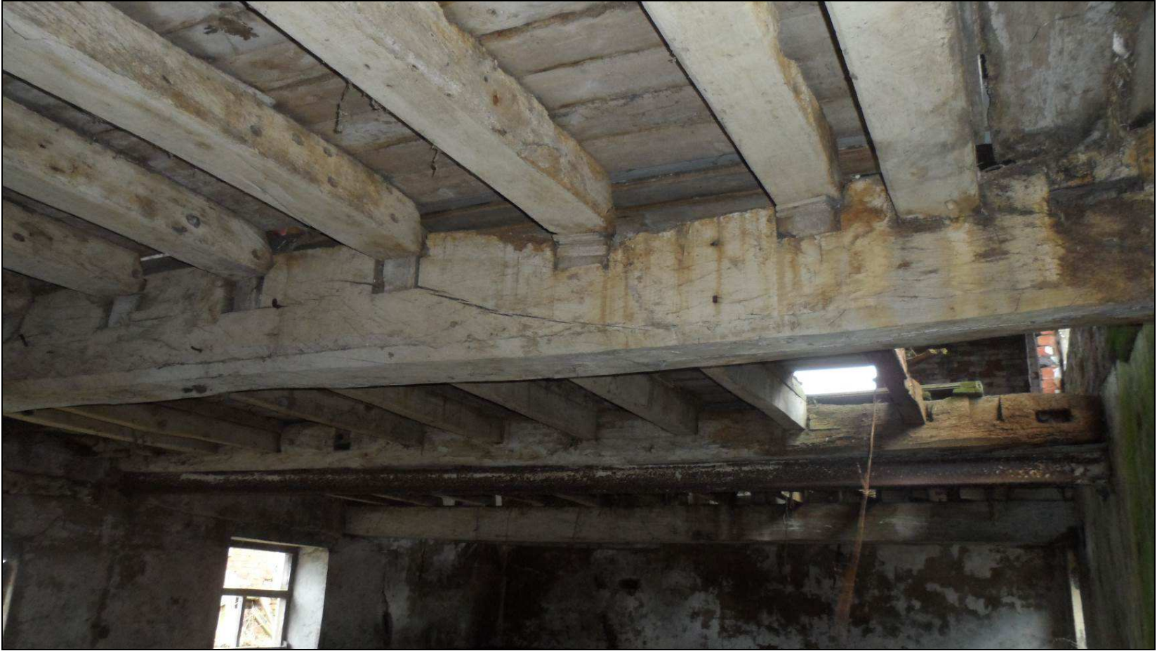
Figure 10: Barn, floor frame with beam 2 and bay 3 in the foreground; it can be seen that the joists of bay 3 do not sit in the original housings, photograph taken from the north (Alison Arnold)
