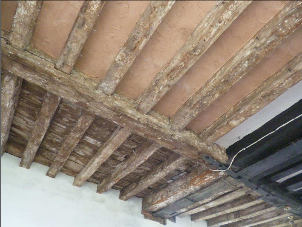
Figure 6: Farmhouse, primary floor frame (left of photograph), photograph taken from the north-west (Robert Howard)
