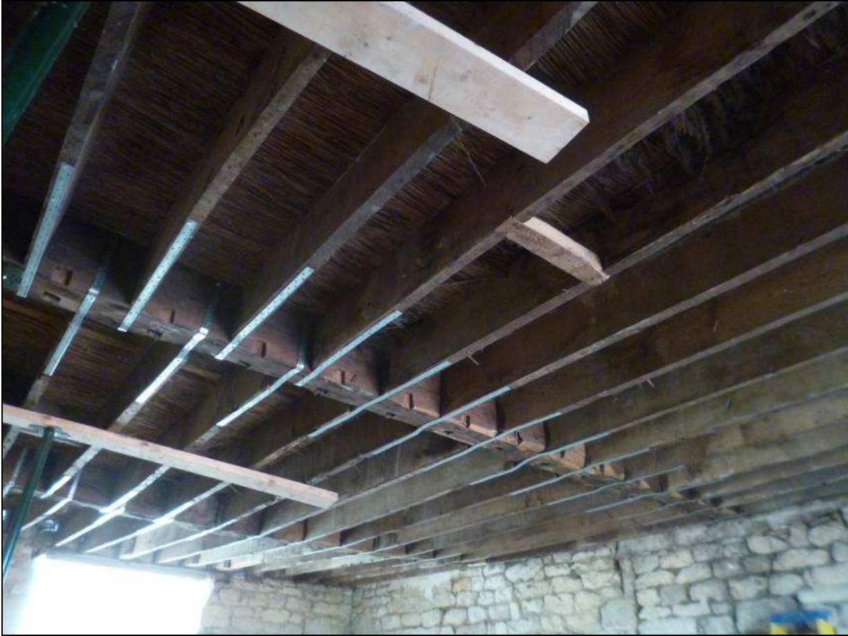
Figure 6: West wing, ground-floor ceiling, photograph taken from the north (Alison Arnold)
