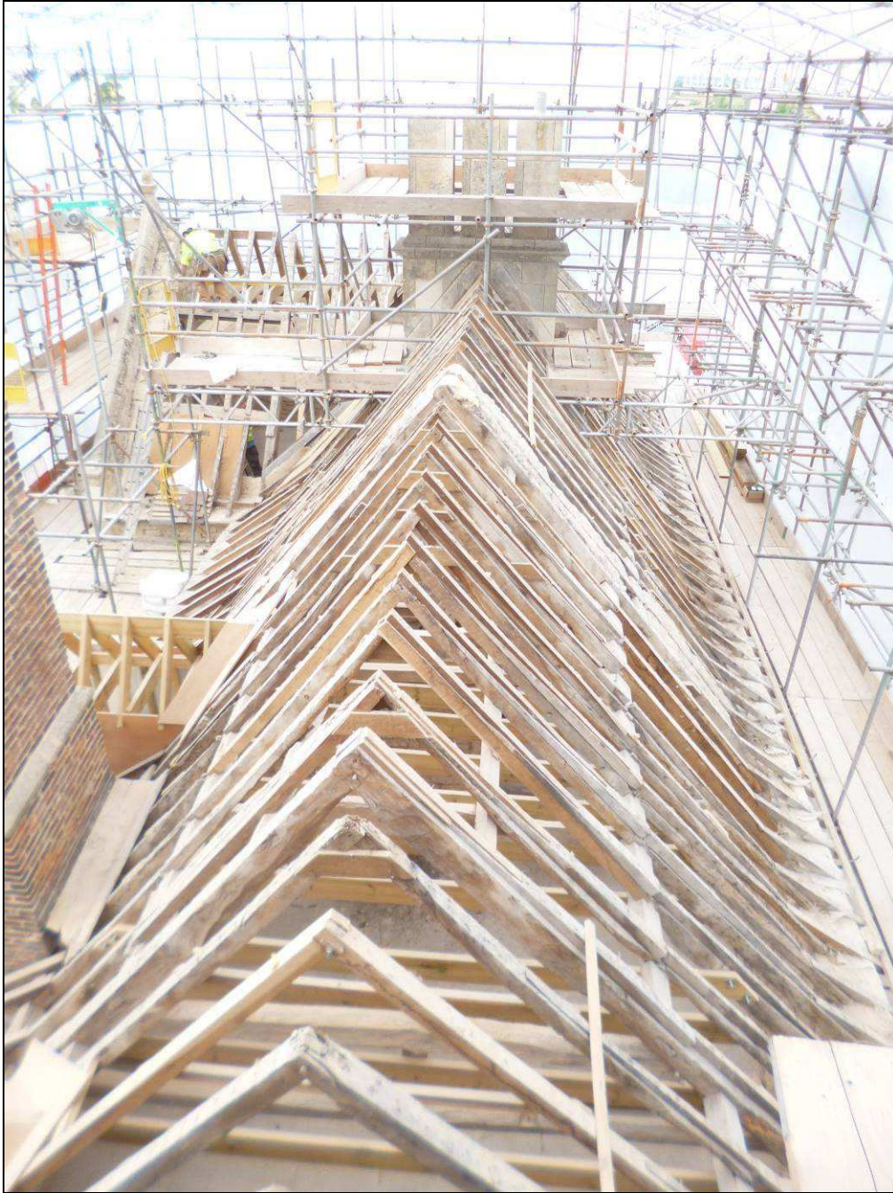
Figure 4: Main range (foreground) and west wing roofs, photograph taken from the east (Alison Arnold)
