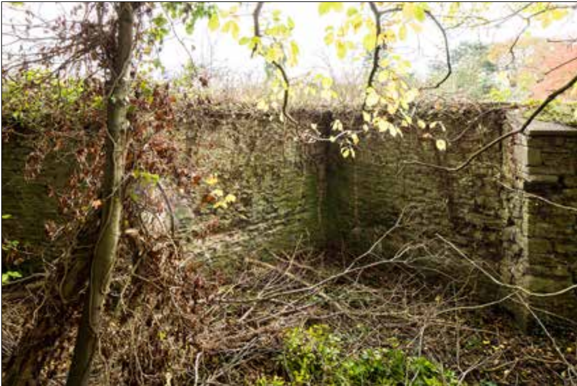
Figure 19: North side of the triangular projection (D) showing alternative method of construction (DP174240 © Historic England, photograph taken by Alun Bull)
