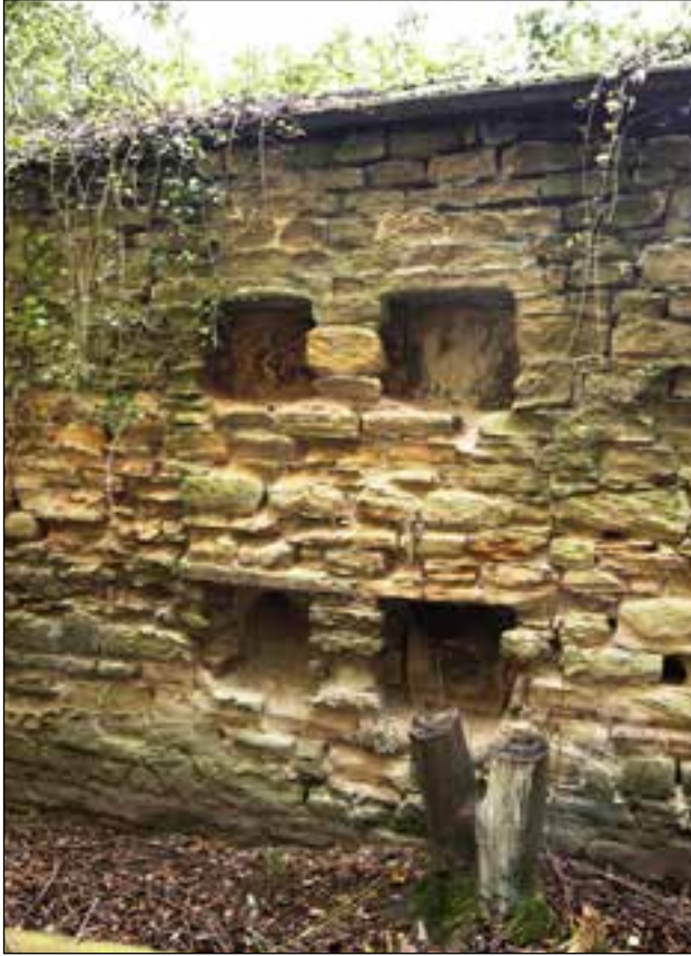
Figure 21: Flue openings on the north side of the garden wall, west of projection E (DP174238 © Historic England, photograph taken by Alun Bull)
