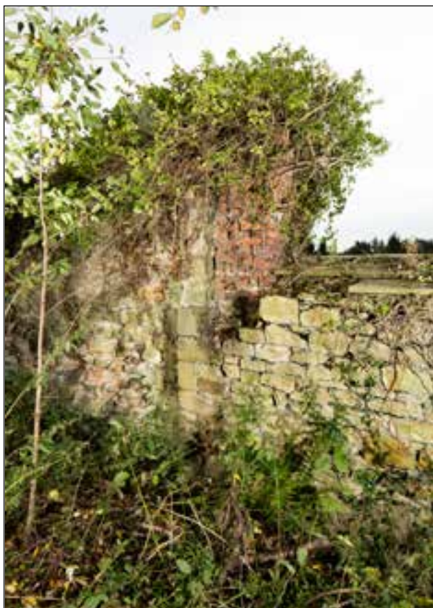
Figure 20: Straight joint (I) on the north face of the garden wall (DP174242 © Historic England, photograph taken by Alun Bull)
