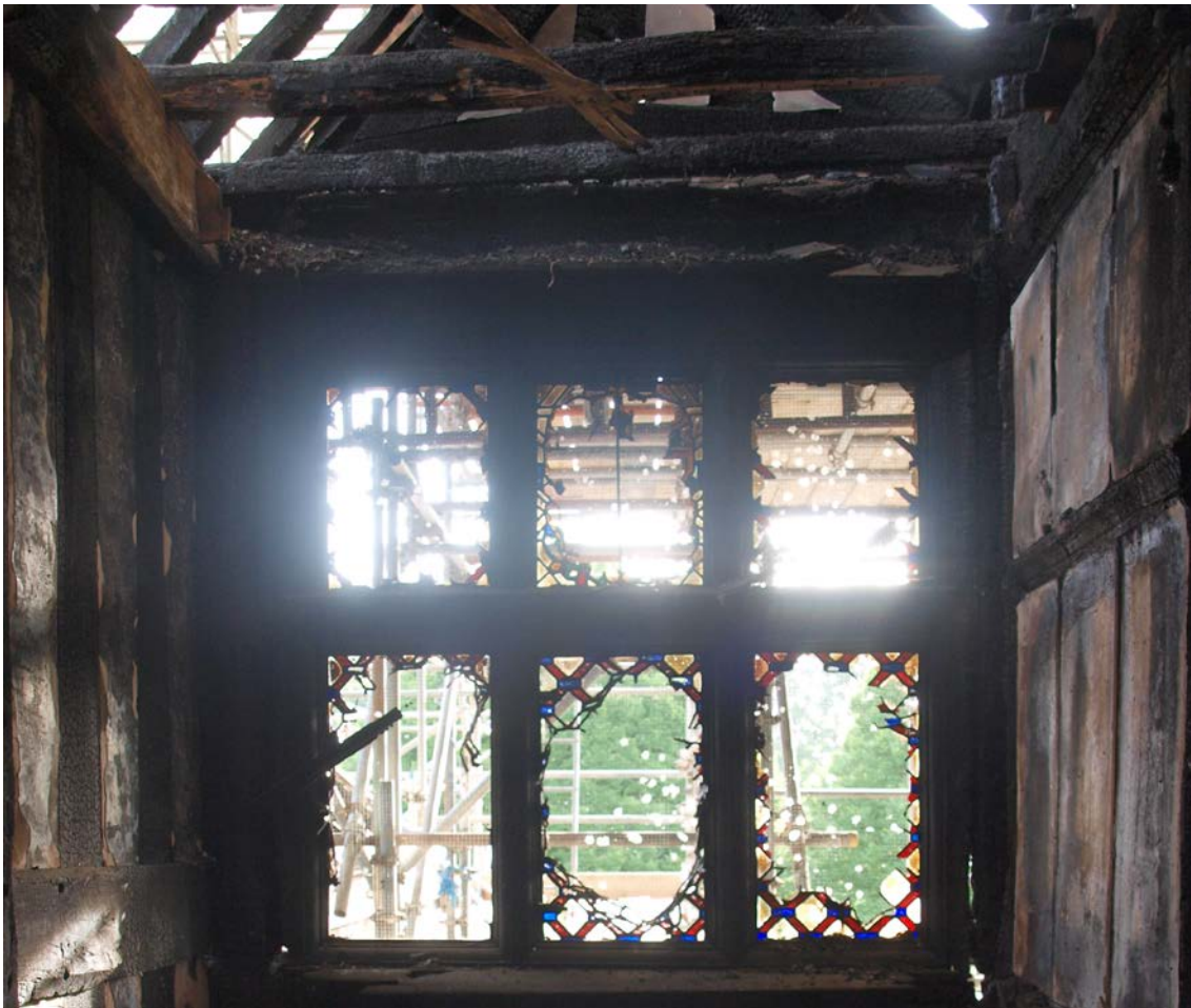
Figure 1. Wythenshawe Hall, window F9 showing extensive fire damage
