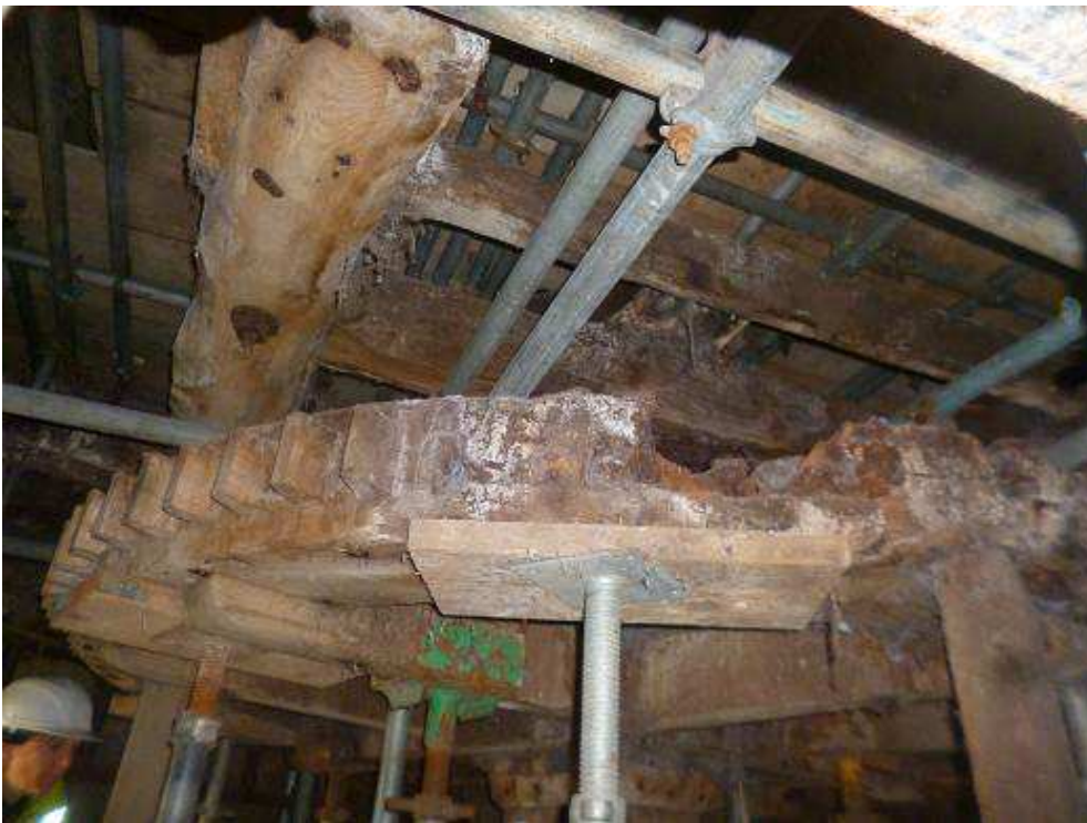
Figure 2a–b: Interior views of Sneath’s Mill showing timber structure and scaffold support (photographs Robert Howard)
