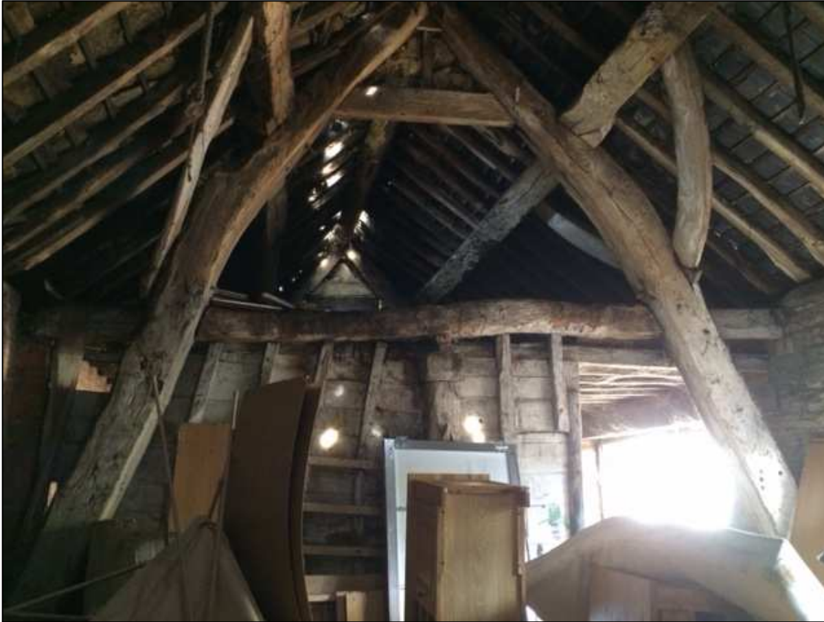
Figure 6: Timber partition separating bays 1 and 2, photograph taken from the south (Alison Arnold)
