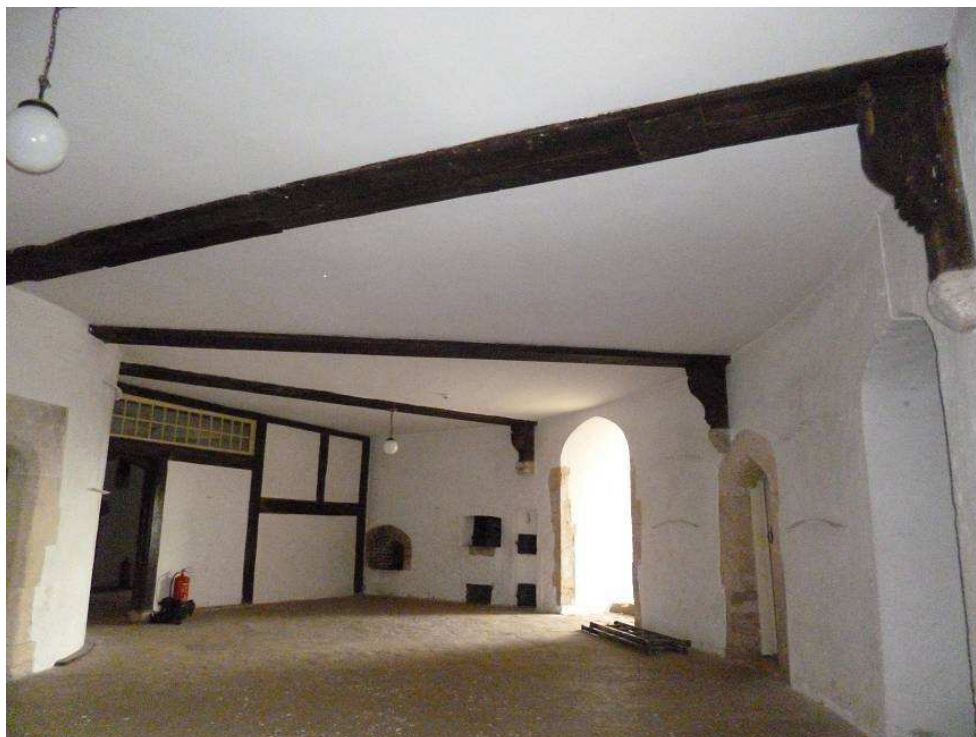
Figure 2a–b: View of the timbers to the Gatehouse roof (top), and the ceiling beams, consoles, and partition wall timbers of the Central Tower (bottom) (photographs Robert Howard)
