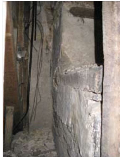
Figure 25.3 Looking north under the stair to the Cock Loft, showing long beam, embedded in rubble wall.
