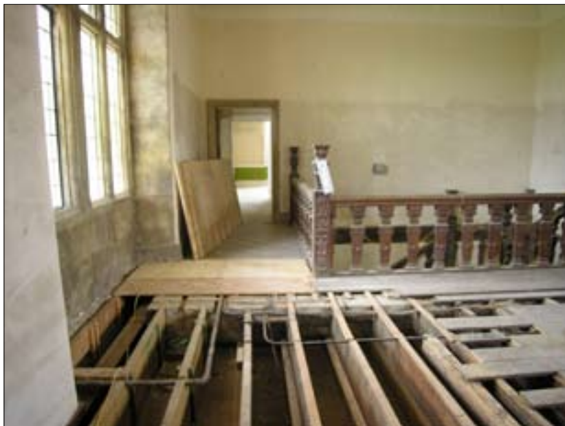
Figure 39.1 Removal of floorboards has revealed main east-west beam. Taken from the north.
