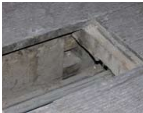
Figure 39.3 Detail showing construction of mortise in the wrong position. Taken from the north.
