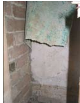
Figure 40.2 Straight joint between brick wall of fireplace and back wall. Taken from the east.
