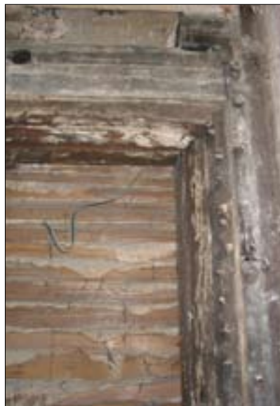
Figure 38.2 Detail of door jamb incorporated into stud walling. Taken from the west.
