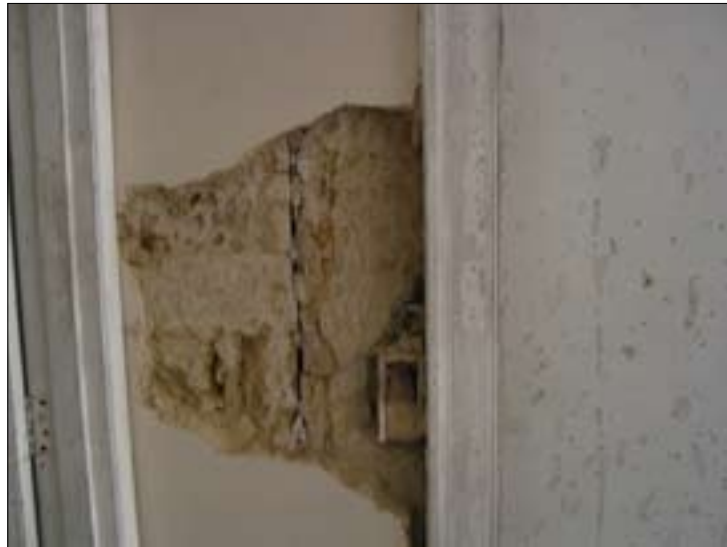
Figure 23.1 Straight joint between ashlar quoins and rubble walling. Taken from the north.
