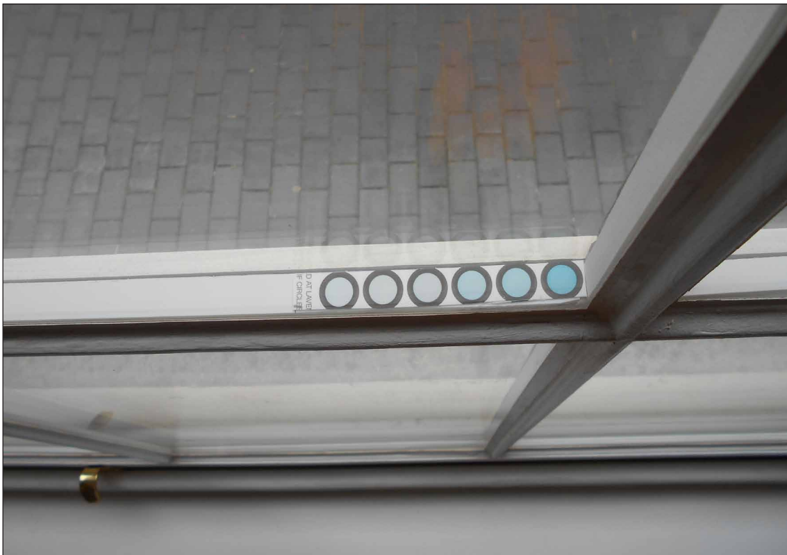
Figure 16: A humidity card inserted between the original glazing and the acrylic pane of the double glazing system in the ground floor reception area.
