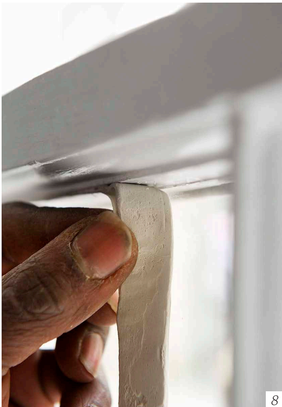
Figure 6: An acrylic pane being fitted between the glazing bars of the original window.
