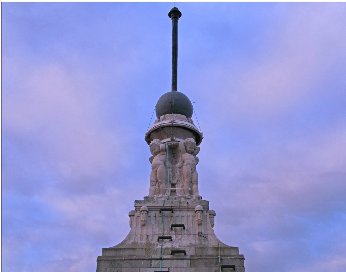
Fig. 23: Drone footage of the step irons leading up to the putti on the north face of the tower. HGH16V052 © Historic England
