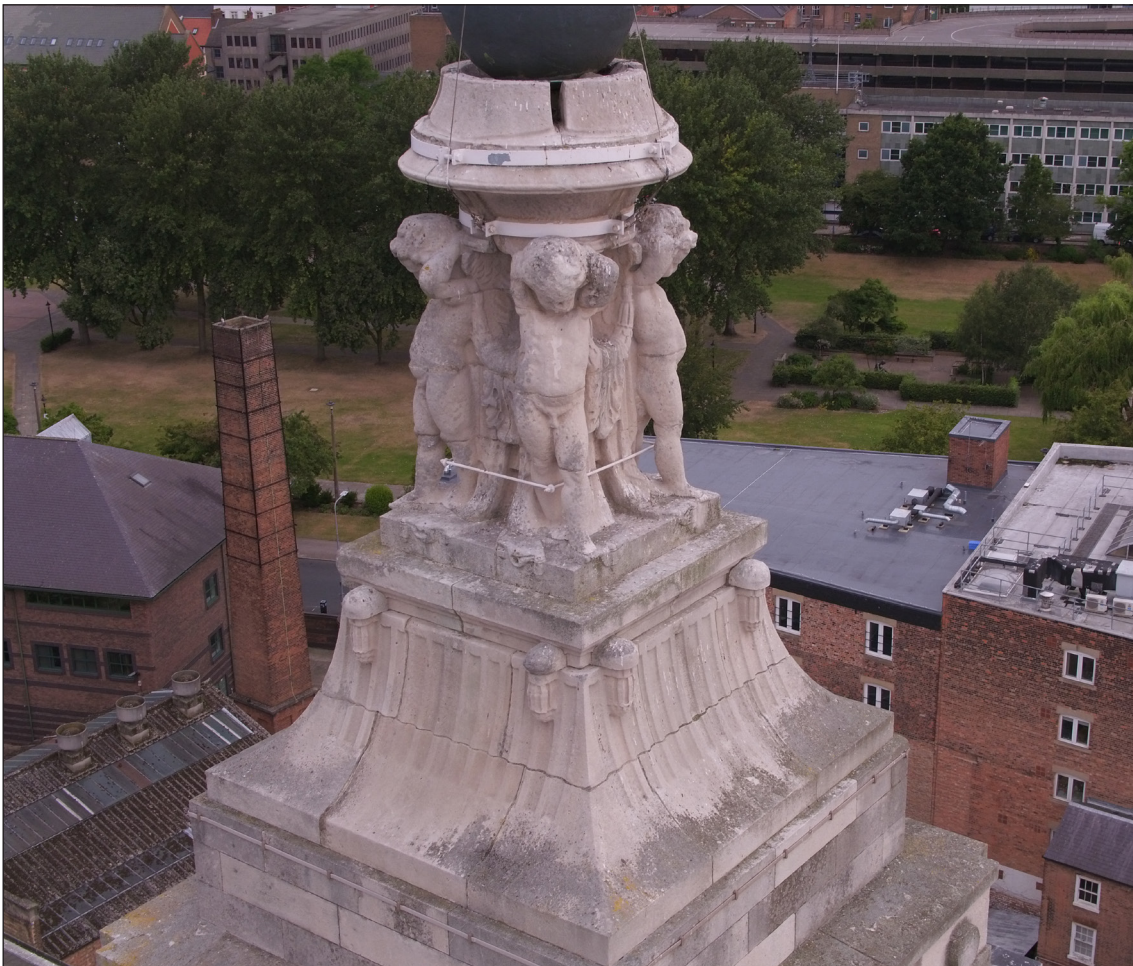
Fig. 19: Drone photograph of the putti supporting the 'cup' into which the time ball drops. HGH16V540 © Historic England
