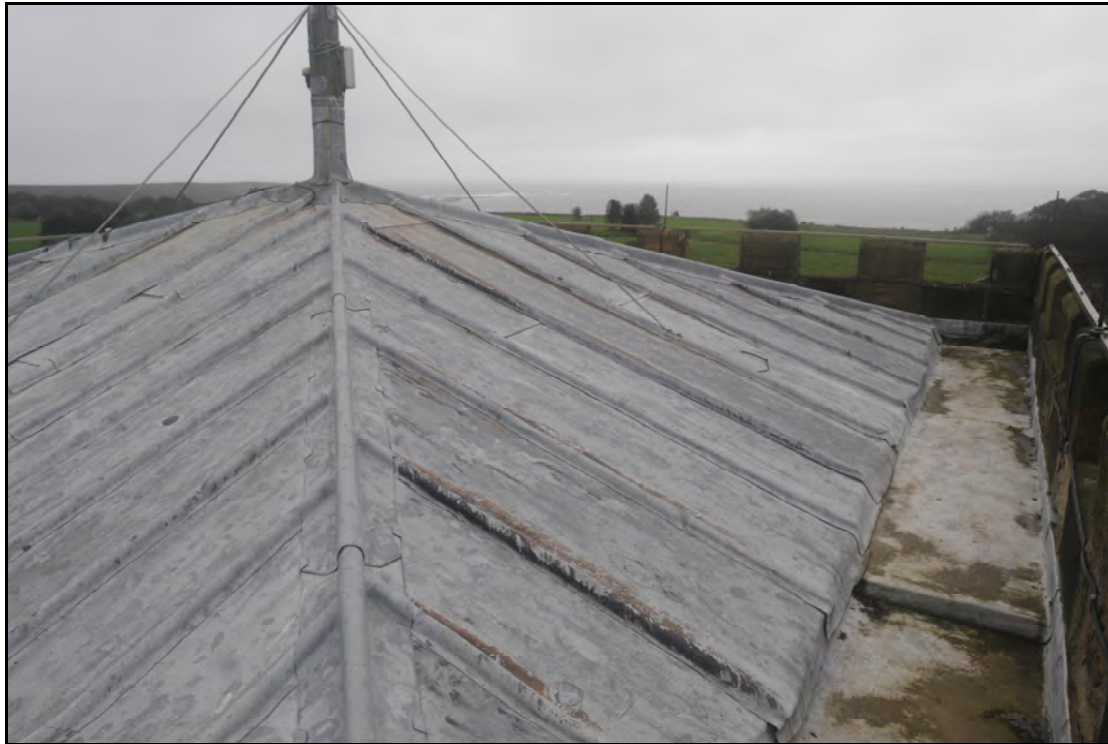
Figure 3. General view of south side of tower roof showing roll joints in lead
