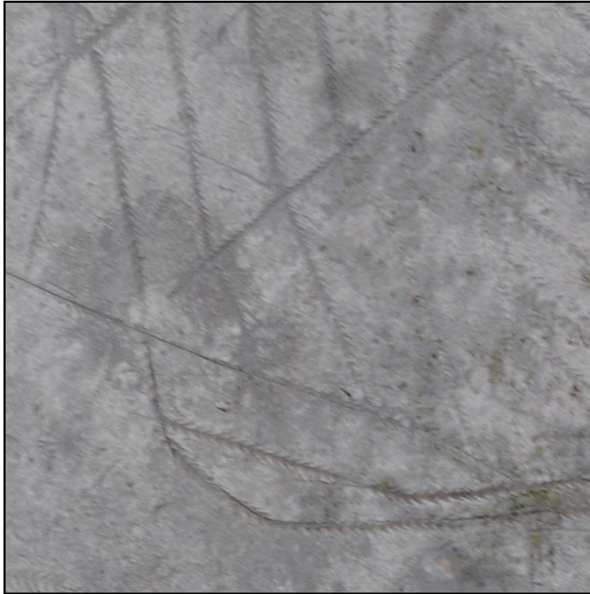
Figure 65. Panel S3 with setting out lines for the wriggle work to follow
