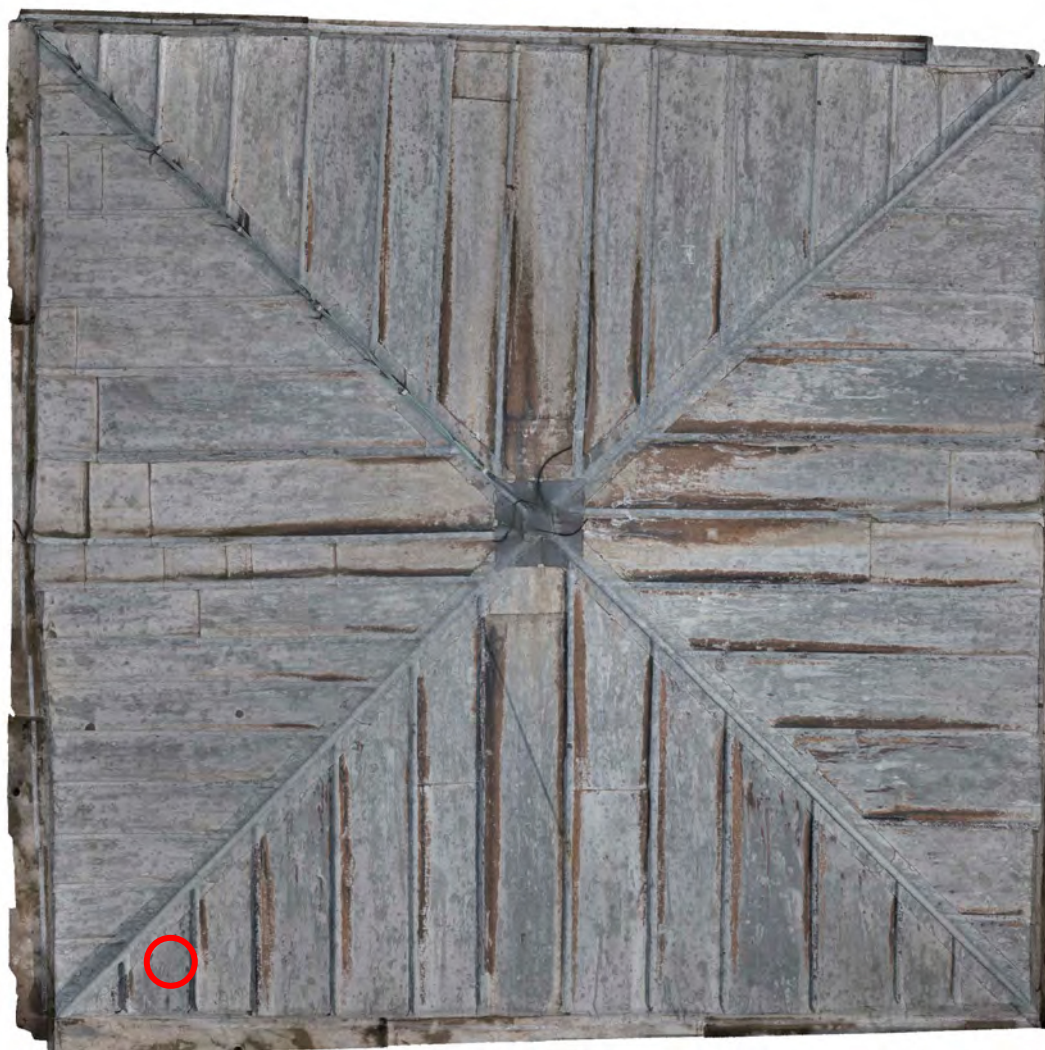
Figure 5b. Photomosaic of the whole roof generated by the photogrammetry with shoe graffiti marked in red reproduced below
