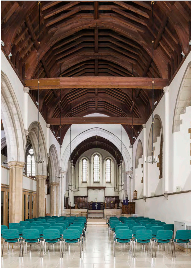
Figure 107: The nave of the Church of All Saints, Highcliffe, taken from the west (DP172525 © Historic England, photograph: James O Davies).
