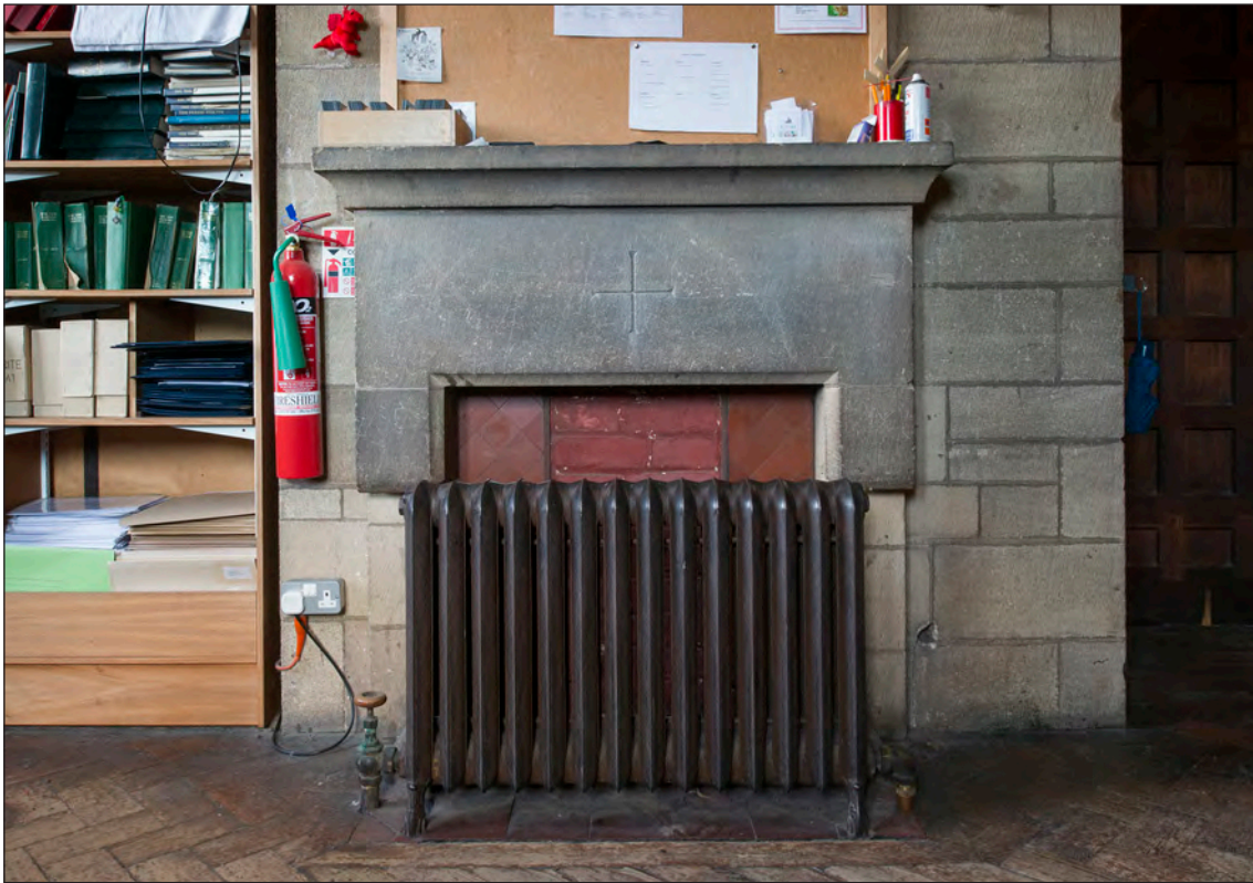
Figure 41: A radiator inserted in front of a fireplace in the vestry at the Church of St George, Cullercoats (DPI68612 © Historic England, photograph: Alun Bull)
