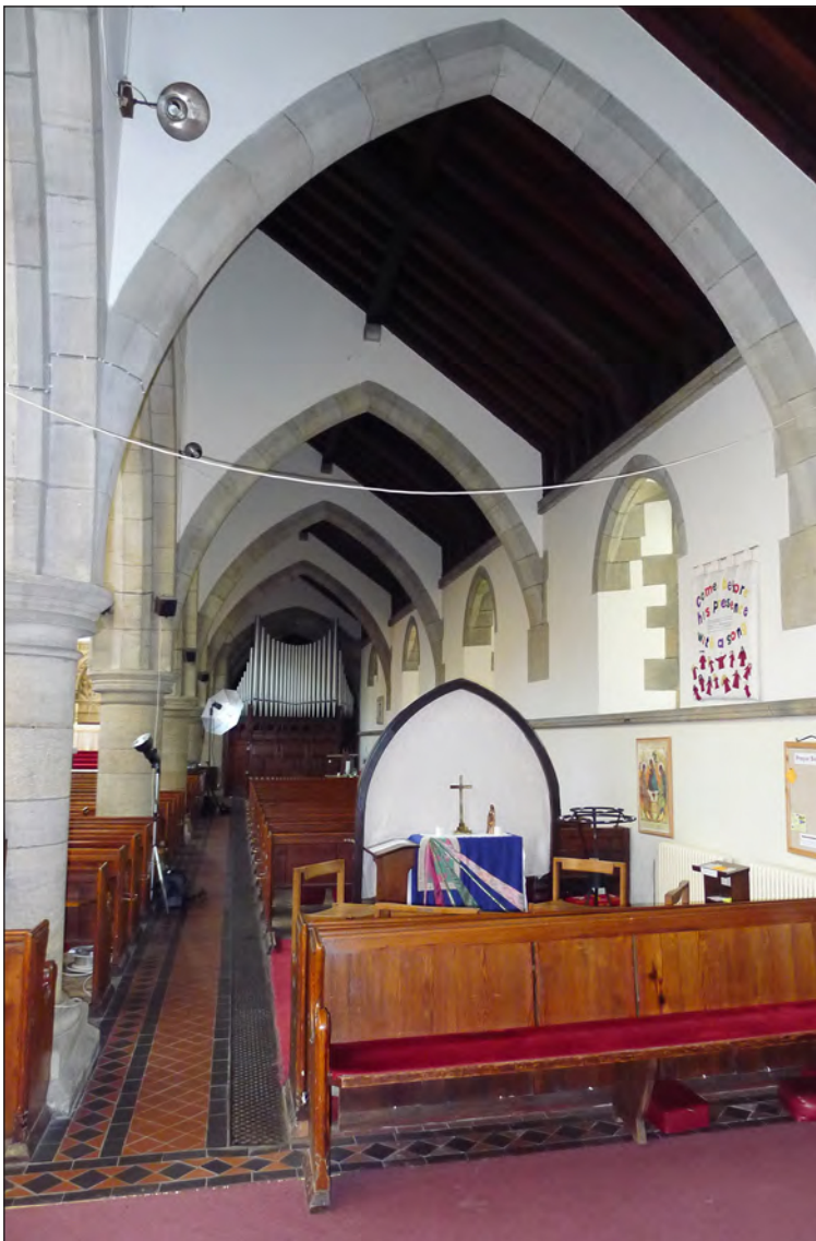
Figure 77: The north aisle of the Church of St Margaret, Horsforth, taken from the south east (© Historic England, photograph: Clare Howard)
