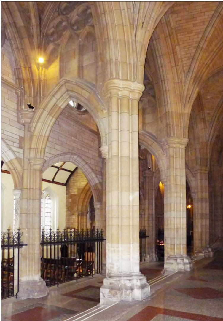
Figure 22: Stone vaulting between the chancel aisle and the incorporated St Mary's Aisle at Truro Cathedral (© Historic England, photograph: Clare Howard)
