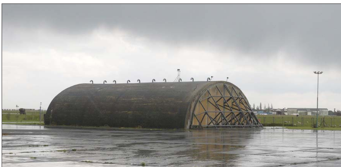
Figure 15: RAF Upper Heyford, a typical third generation hardened aircraft shelter. (c) W D Cocroft
