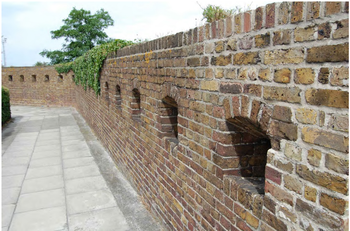
Photograph 10: HCA03 – section of former Ravelin lying between Bridge Road and Tesco carpark
