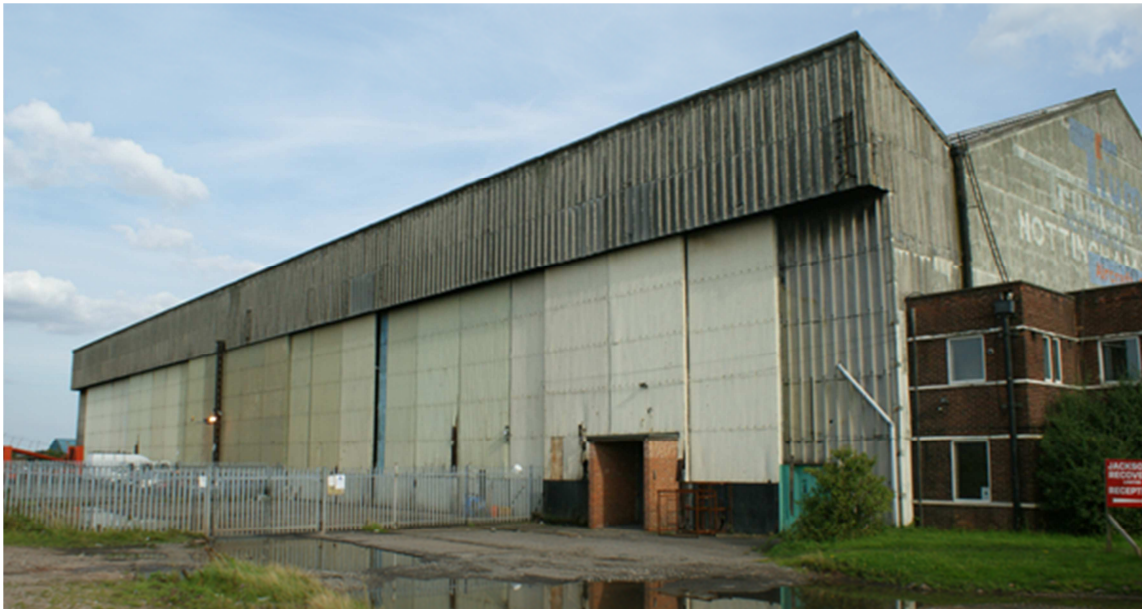
Figure 26: Main hangar, airfield elevation (Bldg.43). Note the roof access ladder positioned close to the fire watcher's shelter (which is hidden behind the wall cladding). [Paul Francis 07-08- 2009]
