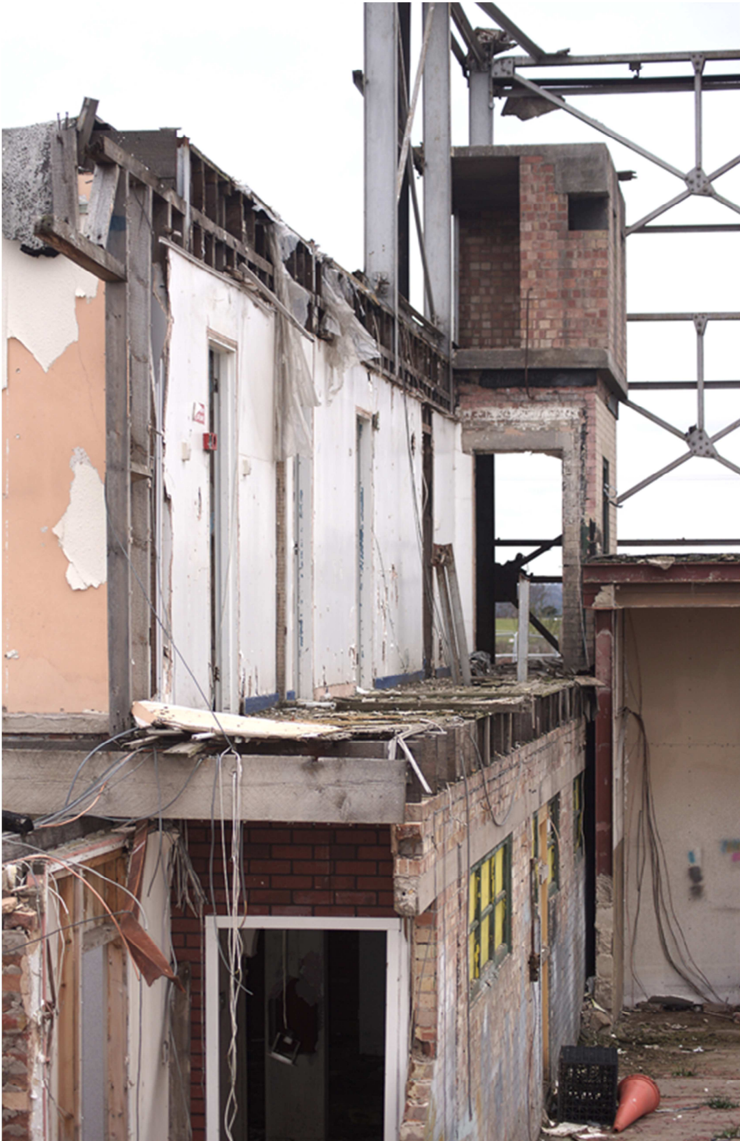
Figure 8: The ground floor and first floor offices and their relationship with the fire watcher's post. [Paul Francis 05-12-2017]
