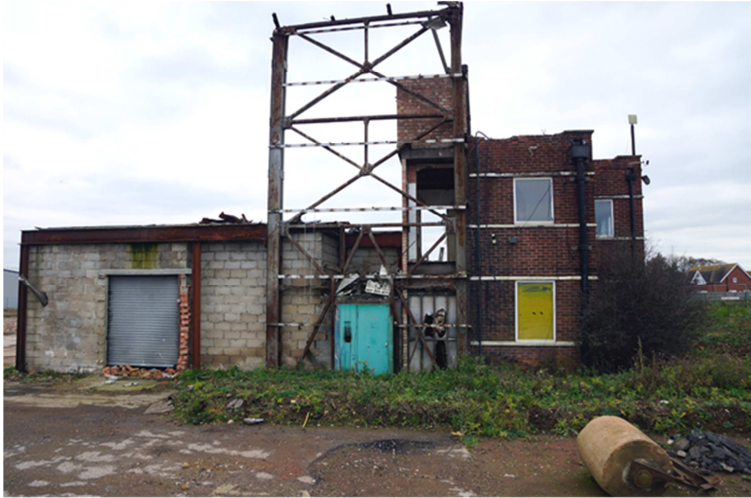
Figure 8: Exterior view looking south showing blind end of the fire watcher's post and door wind bracing. [Paul Francis 05-12-2017]
