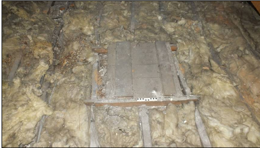
Fig 36: Disused hatch in the floor of Bay 2, viewed from the north (© Historic England, photograph: Dan Elsworth)
