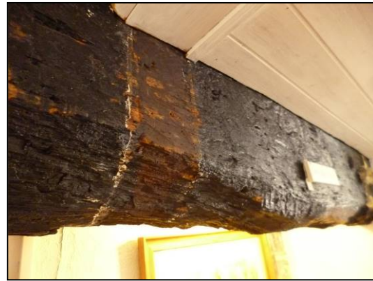
Fig 18: position of former partition on beam in Number 65 (© Historic England, photograph: Marion Barter)
