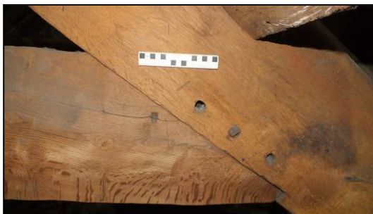
Fig 45: Carpenter's marks at the west end of Truss 4, viewed from the north (© Historic England, photograph: Dan Elsworth)
