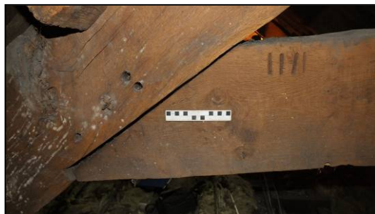
Fig 46: Carpenter's marks at the west end of Truss 4, viewed from the south (© Historic England, photograph: Dan Elsworth)
