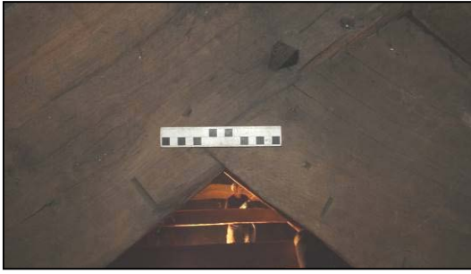
Fig 28: Carpenter's marks at apex of Truss 1, viewed from the north (© Historic England, photograph: Dan Elsworth)
