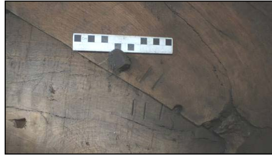
Fig 29: Carpenter's marks on west side of Truss 1, viewed from the north (© Historic England, photograph: Dan Elsworth)
