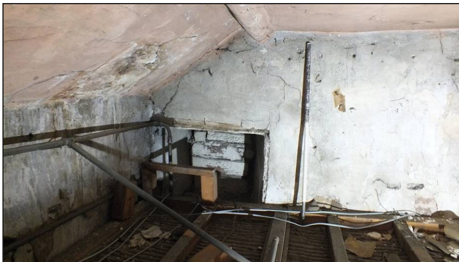
Fig 48: The western blocked window in the north elevation of the space above the current ceiling of the Mayor's Parlour, viewed from the south
