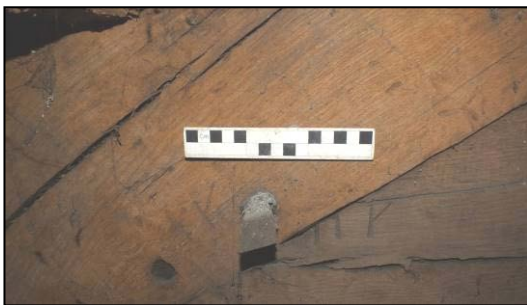
Fig 26: Carpenter's marks on east side of Truss 1, viewed from the north (© Historic England, photograph: Dan Elsworth)
