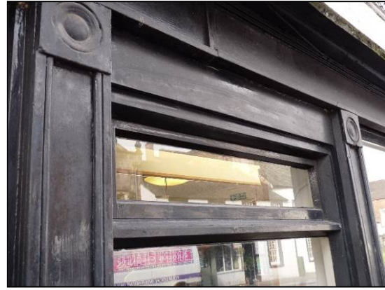
Fig 53: shopfront details include paterae and moulded pilasters, typical of the early 19th century (© Historic England, photograph: Marion Barter)
