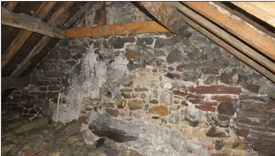
Fig 24: The south gable showing the change in wall height, viewed from the north-west (© Historic England, photograph: Dan Elsworth)
