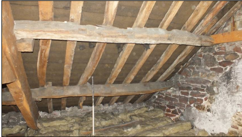
Fig 47: Re-used timbers forming purlins on the east side of Bay 5, viewed from the north-west (© Historic England, photograph: Dan Elsworth)
