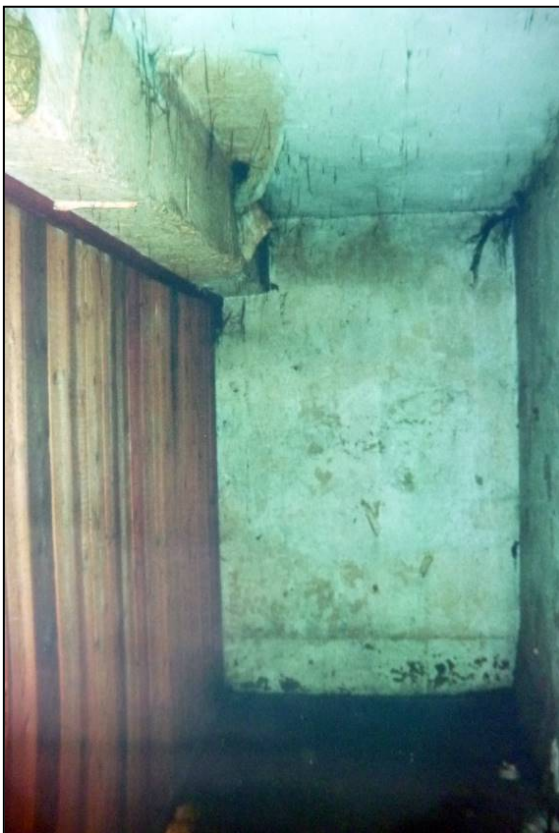
Fig 19: the interior of the gallery from the west, with roof truss tie-beam to top left (Appleby Town Council collection)
