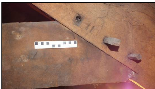
Fig 34: Carpenter's marks at west end of Truss 2, viewed from the north (© Historic England, photograph: Dan Elsworth)
