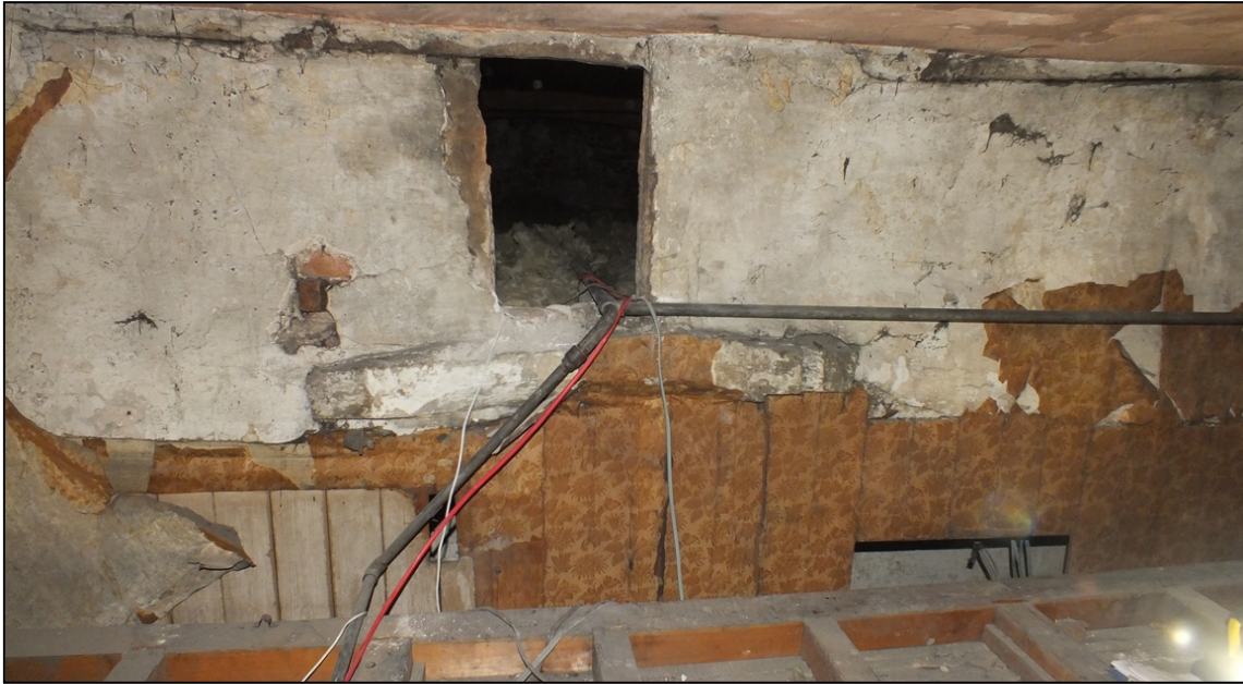
Fig 50: The south elevation in the space above the Mayor's Parlour showing access into the attic above the council chamber in the timber partition wall, viewed from the north (© Historic England, photograph: Dan Elsworth)
