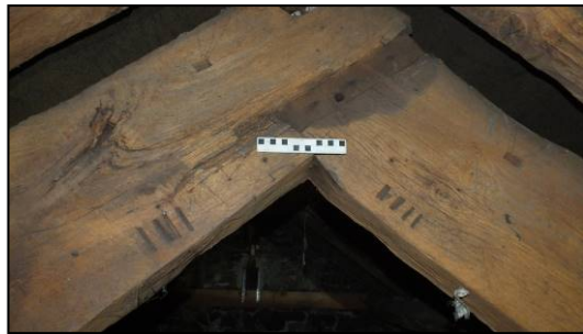
Fig 44: Carpenter's marks at the apex of Truss 4, viewed from the north (© Historic England, photograph: Dan Elsworth)
