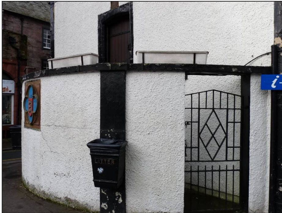
Fig 57: the screen wall to the external south staircase, from the east (© Historic England, photograph Marion Barter)
