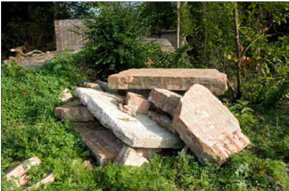
Battery Observation Post from the south east showing portions of brick walling.
