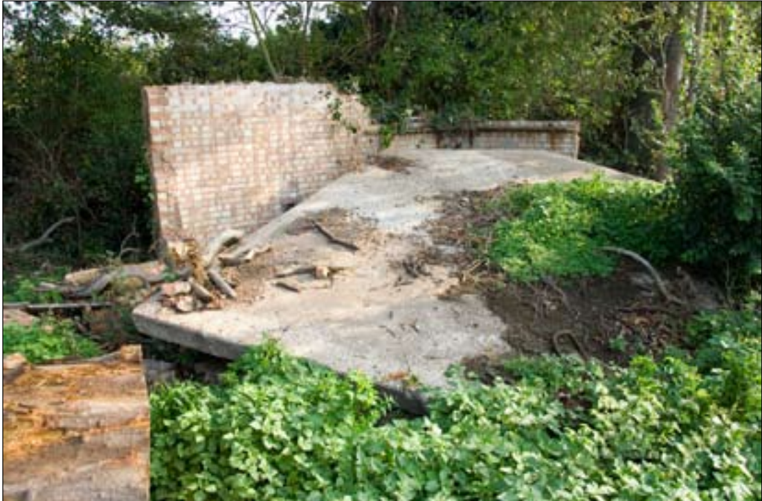
Battery Observation Post following demolition from the north west. Roof slab in foreground.
