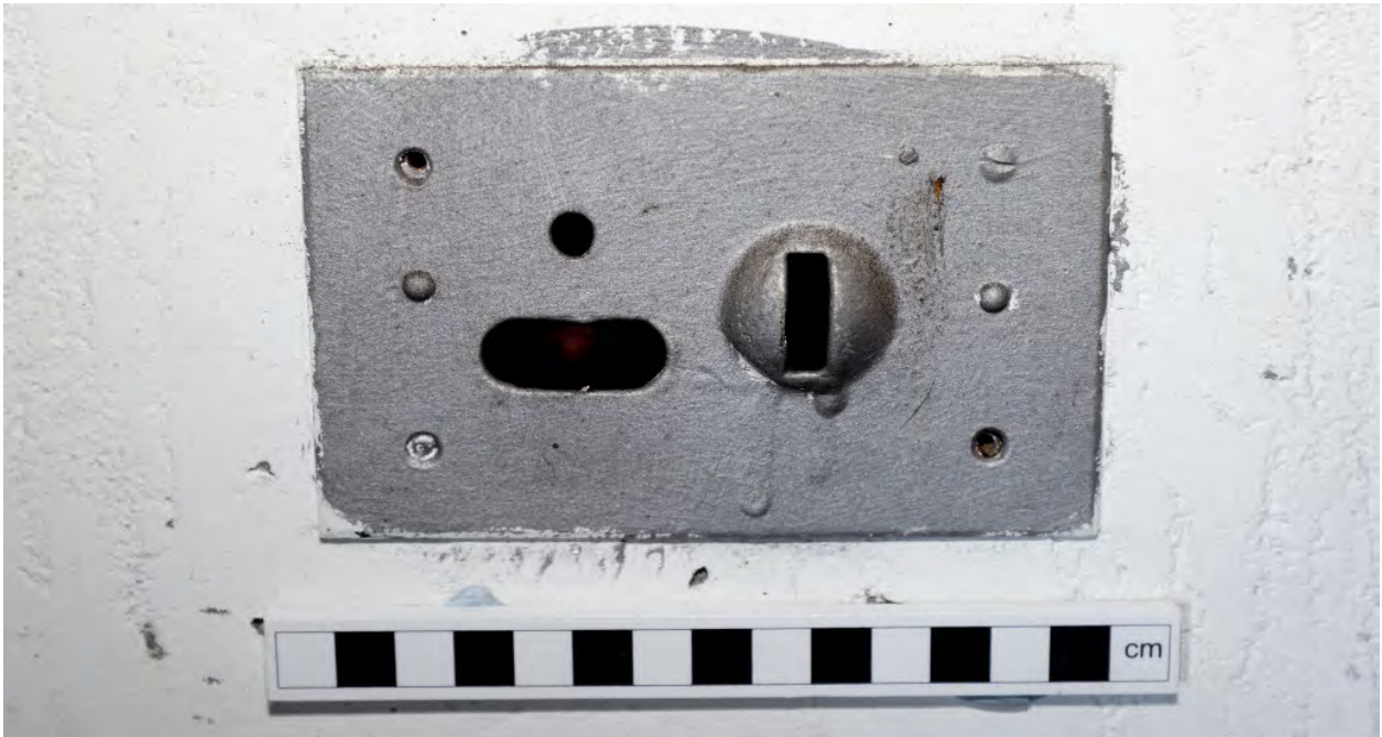
Plate 38: Wall mounted electrical switched socket plate of a type found in various rooms
