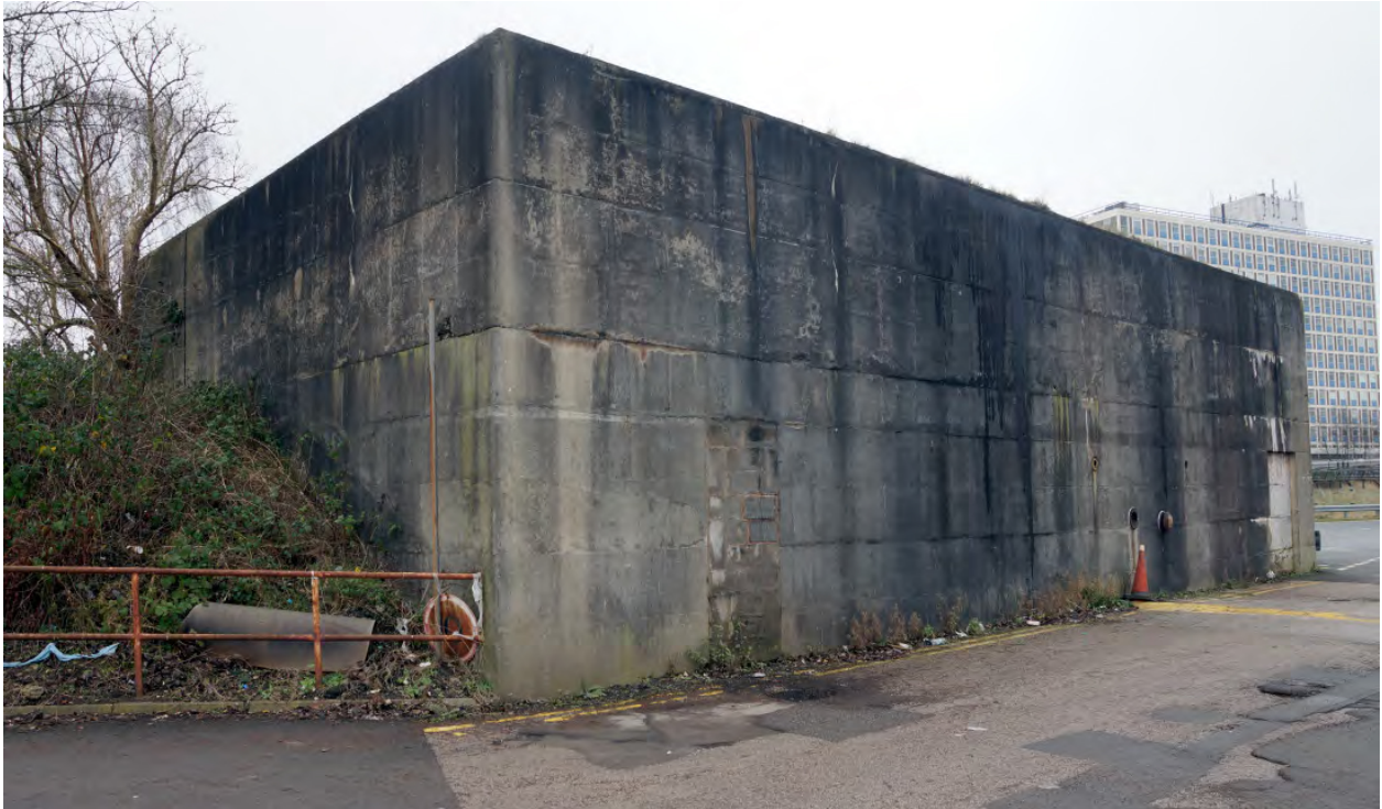
Plate 12: Type A1 Divisional Control Room, Crewe – view looking at the emergency exit end.
