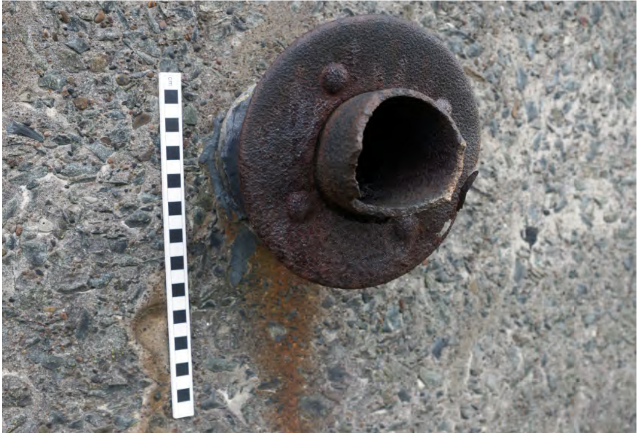
Plate 41: Exterior wall DERV fuel inlet pipe and flange
