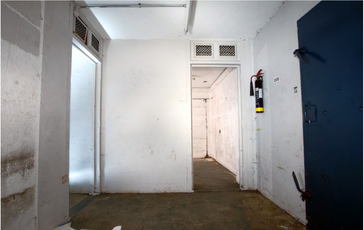
Plate 33: Exit air-lock with splinter-proof steel door and two door frames with exhaust vents above
