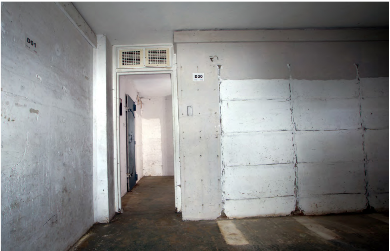
Plate 34: View looking towards the exit air-lock from the control room
