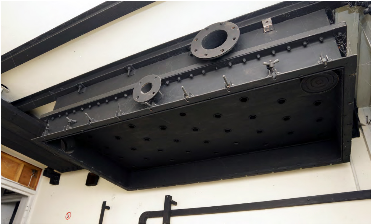
Plate 43: Post-war ceiling mounted ventilation filter
