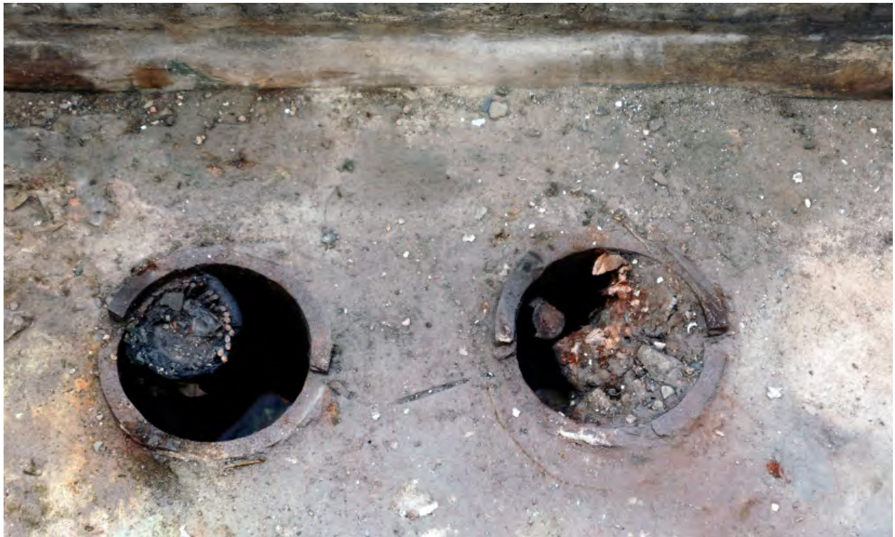
Plate 36: Auxiliary room 3 – underground communication cables and conduit
