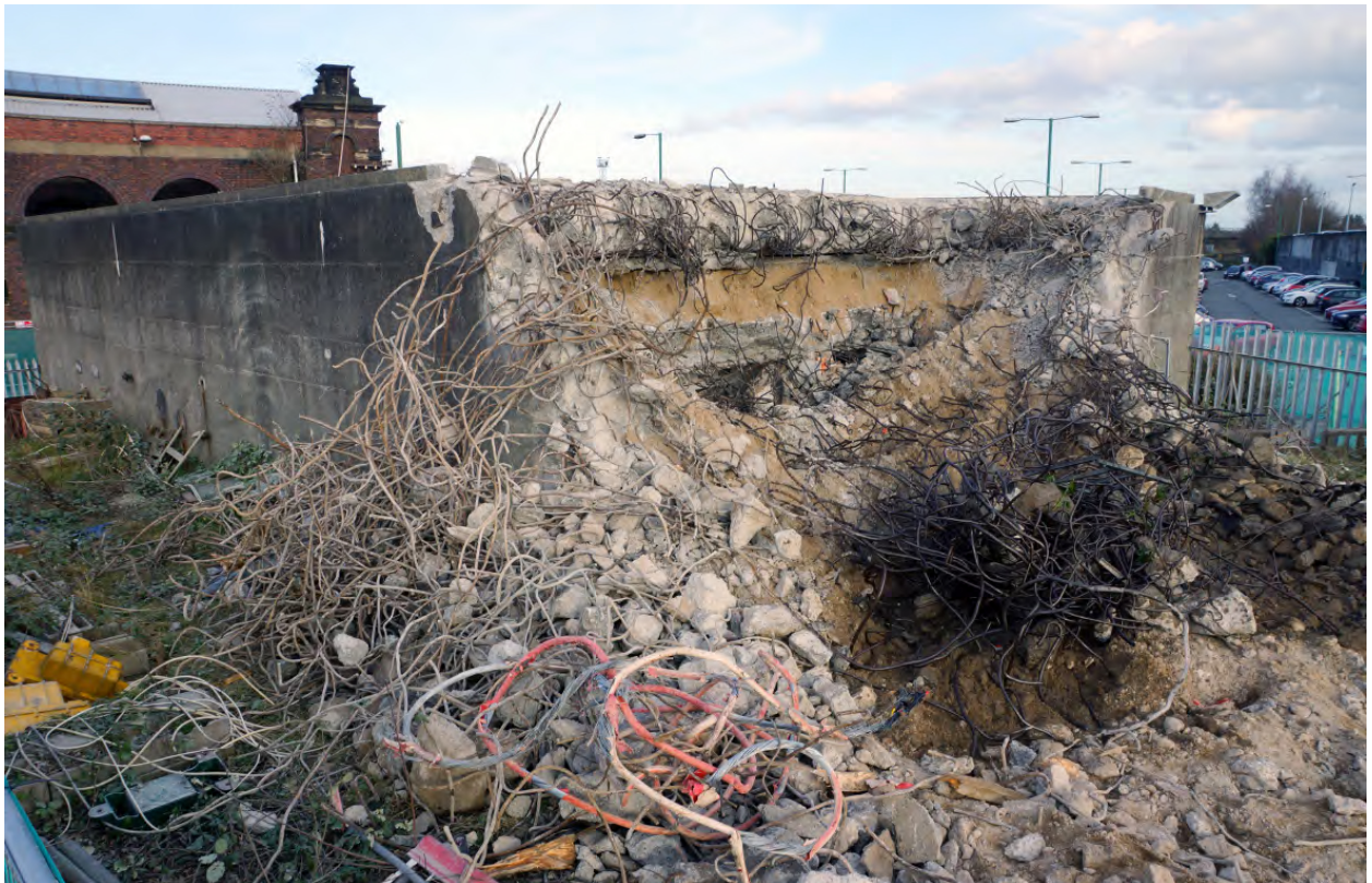
Plate 56: A tangled mess of rebar, concrete and sand
