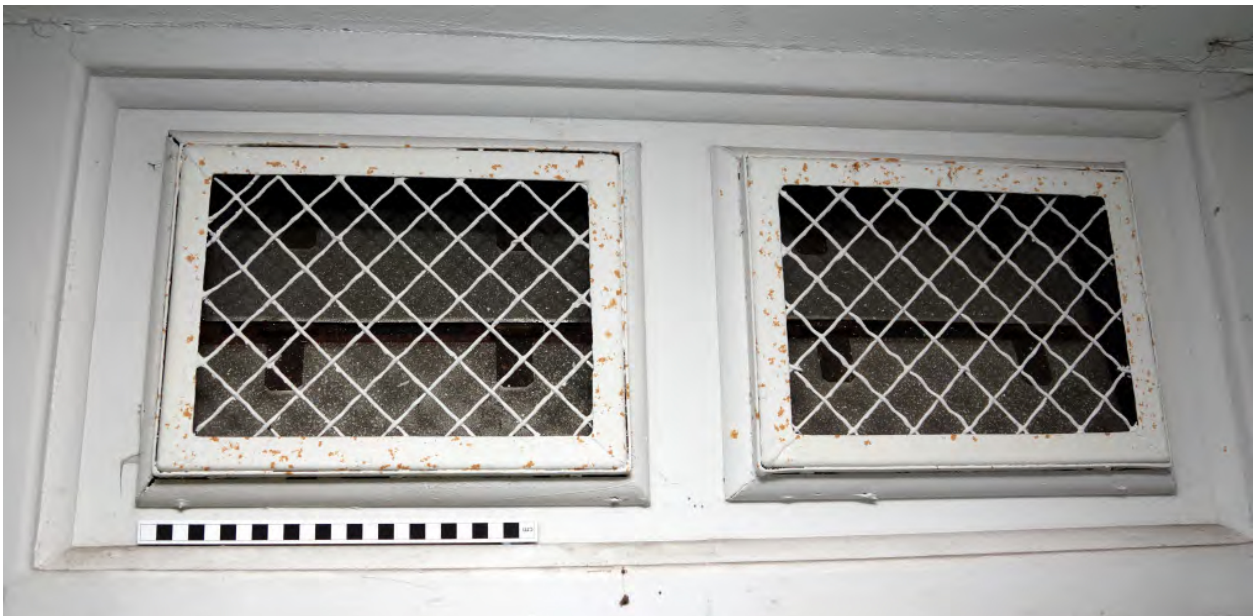
Plate 40: Non-return exhaust valves above the air-lock doors to the control room
