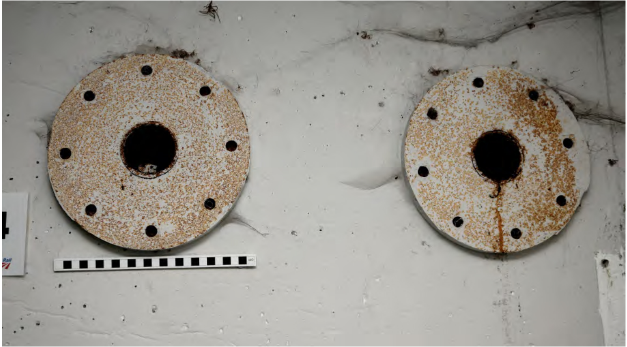
Plate 39: Believed to be vent flanges inside the exit air-lock
