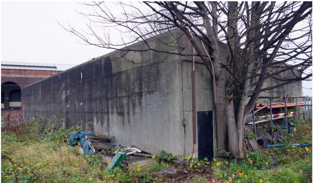
Plate 23: View looking north with exit in end wall It just possible to make out the curb on the roof which is set back from the wall perimeter. Marks made by the shuttering process of laying the concrete can clearly be seen.
