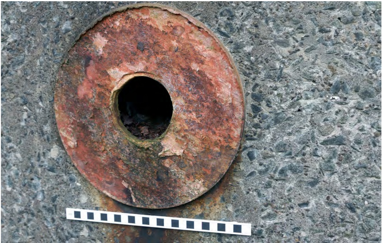
Plate 42: Exterior wall steel flange of what is believed to be a clean air vent - If this is the case then the vent would have risen vertically to take air from above a possible gas cloud. -
