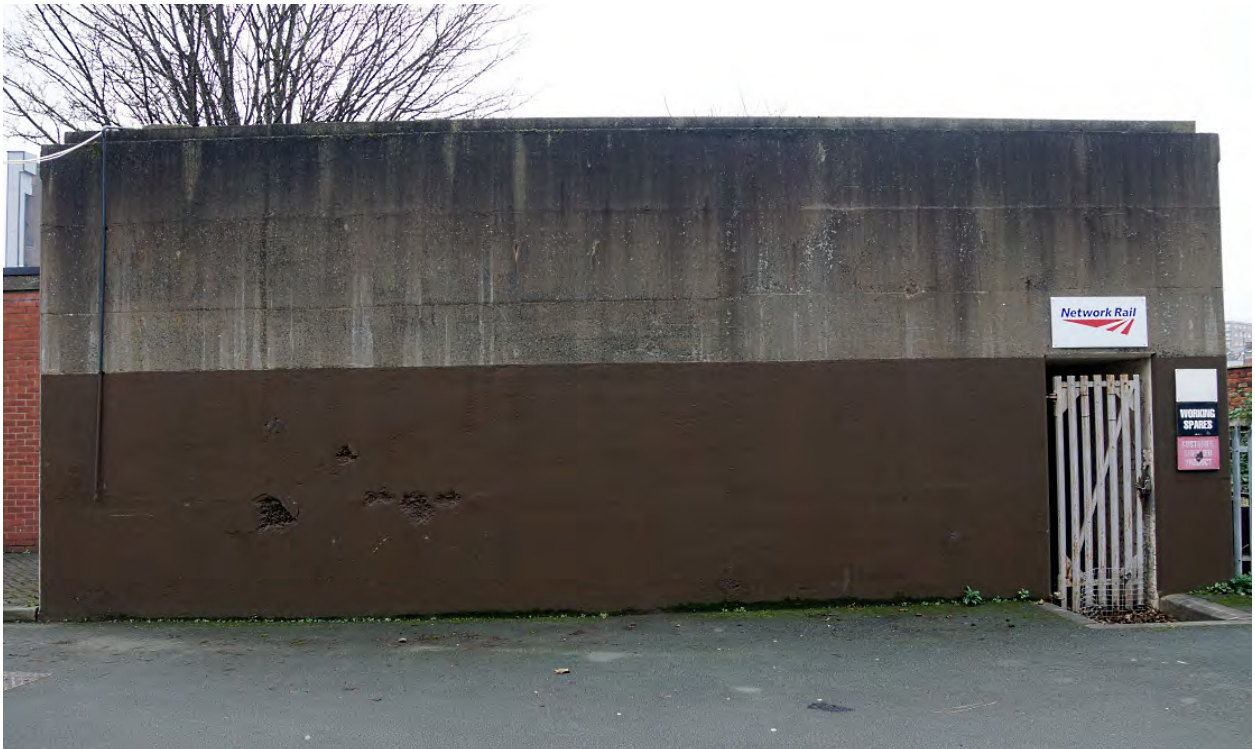
Plate 21: Type A2 District Control Room at Chester – front elevation Note the minor damage to the concrete surface on the left.
