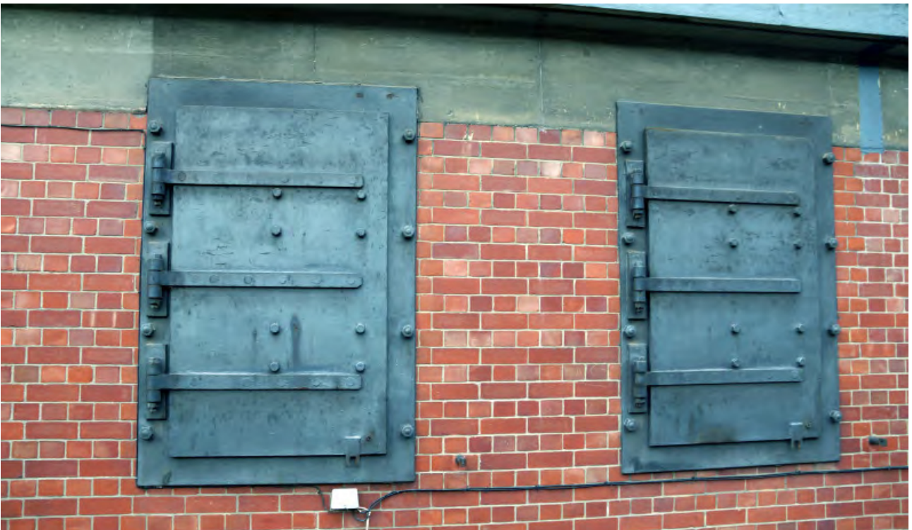
Plate 17: 'Whitegates', Shenfield LNER New Office Building, close-up Showing the substantial metal frames and anti-blast shutters – note too, the English bond brickwork
