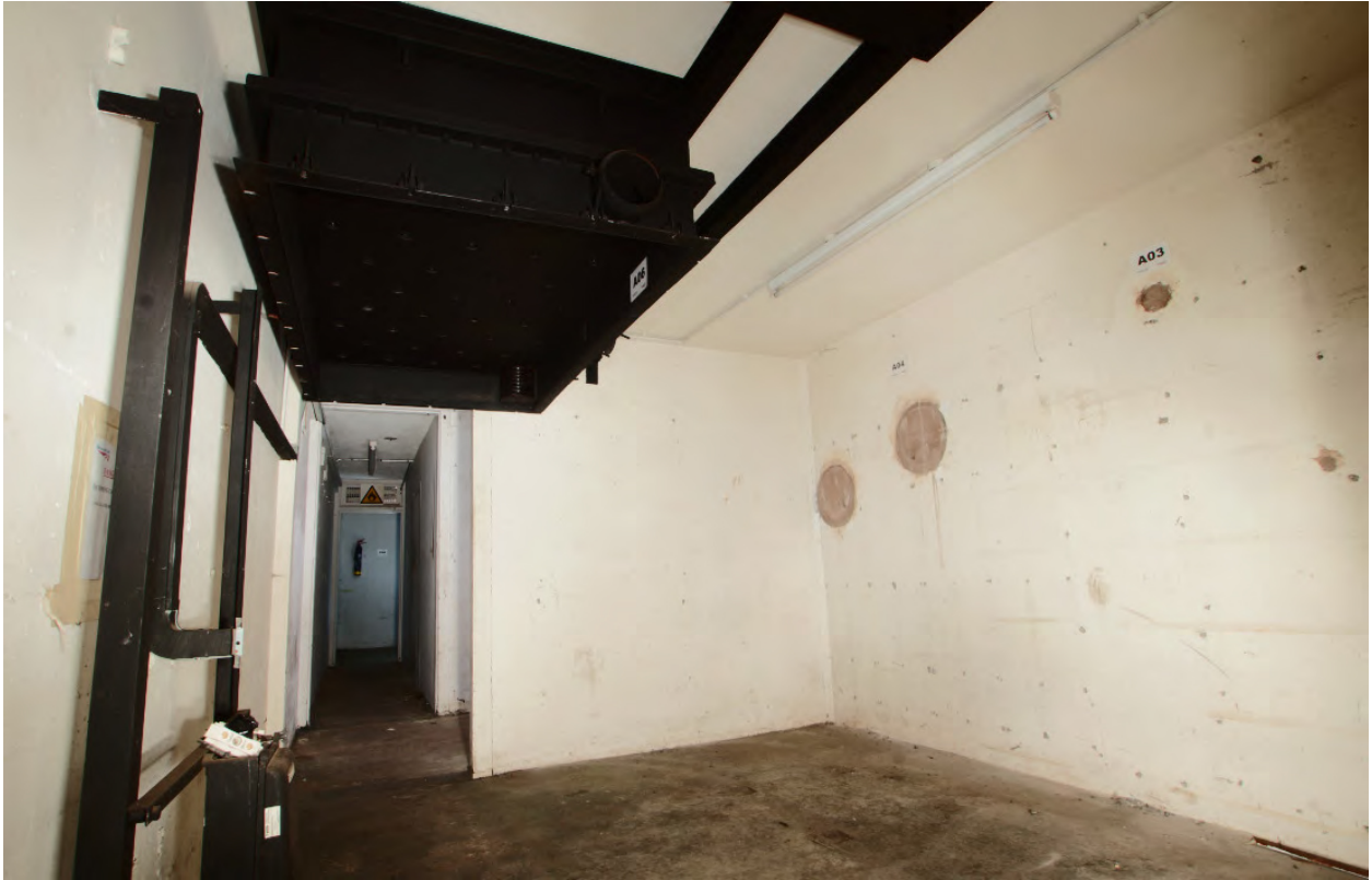
Plate 29: Auxiliary room 1 – generator room
