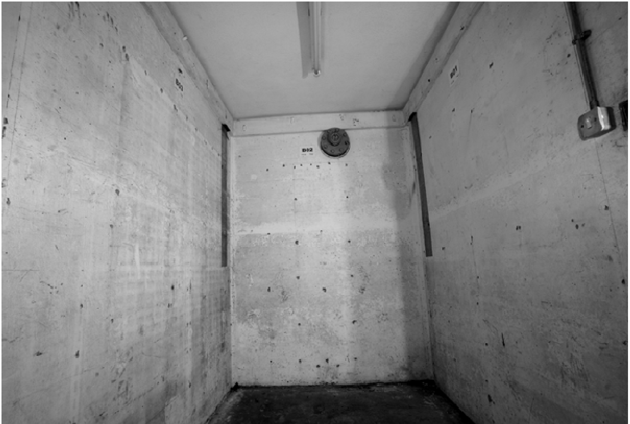
Plate 31: Auxiliary room 2 – battery room
