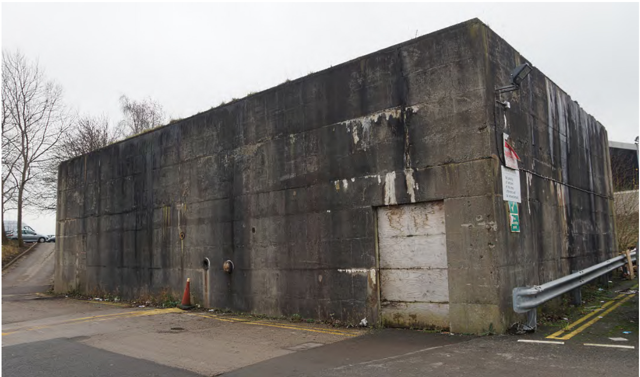
Plate 11: Type A1 Divisional Control Room, Crewe – looking at the main entrance end
