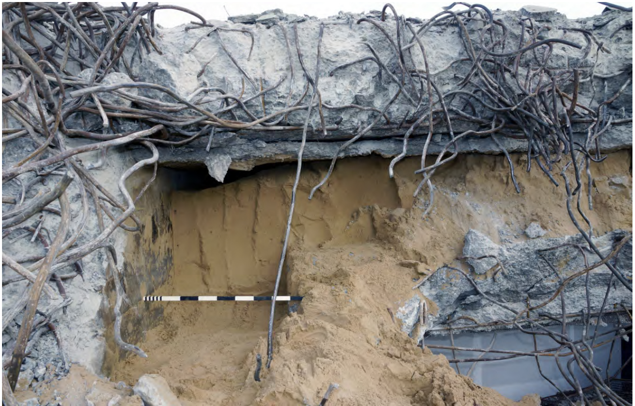
Plate 51: The wall and roof burster layer voids over the emergency exit air-lock
