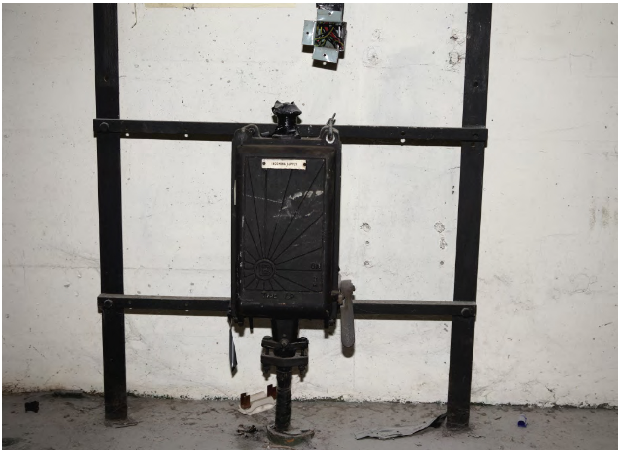
Plate 30: Auxiliary room 1 – incoming electrical mains
