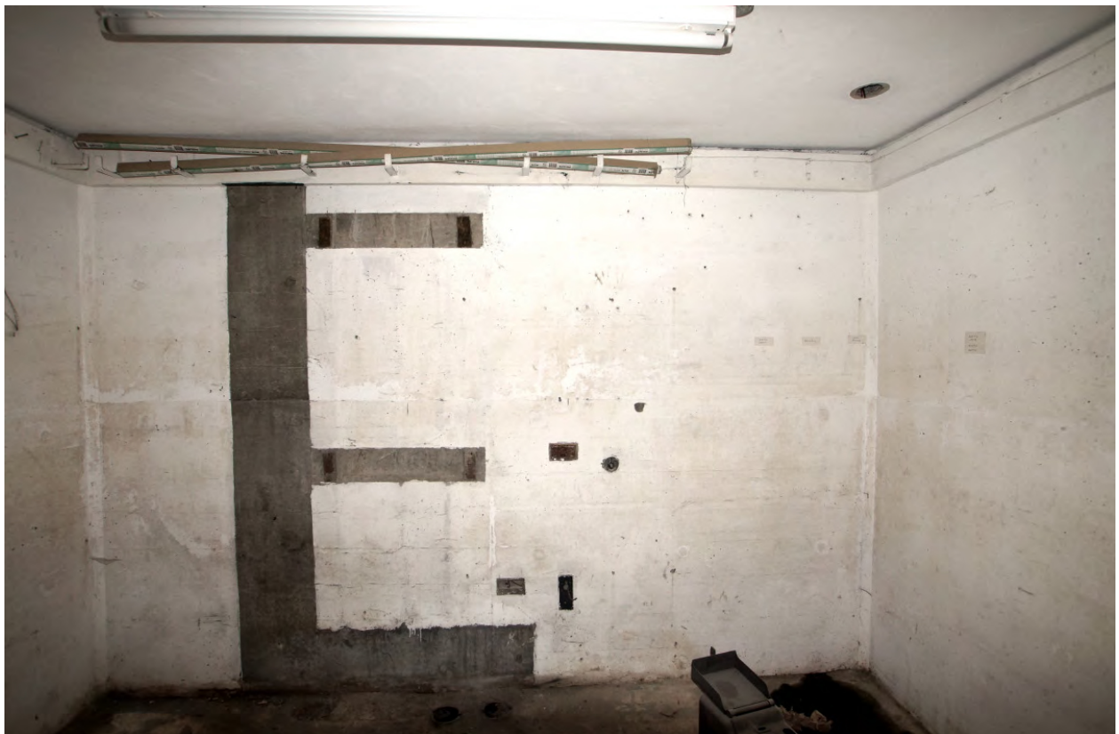
Plate 32: Auxiliary room 3 – phone and switch room Note the timber coving with steel brackets
