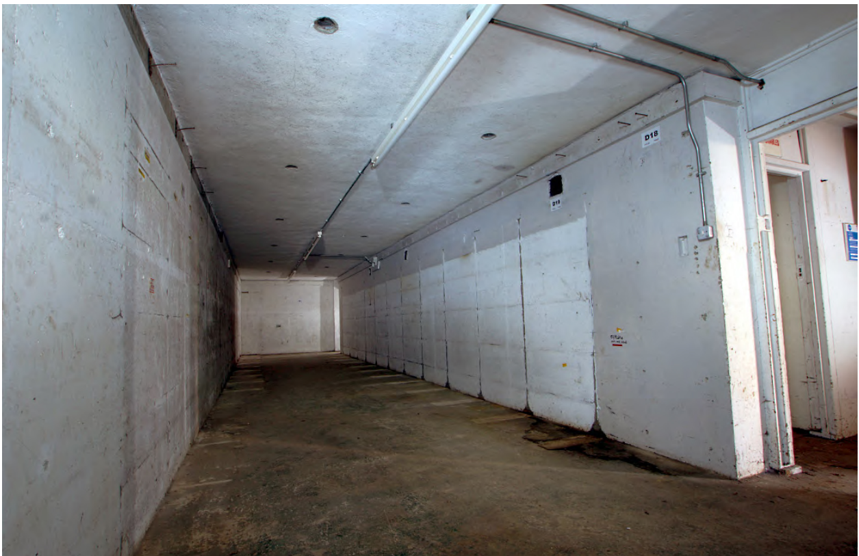
Plate 25: Wide-angle view looking south with doorway from the main entrance air-lock on the right Note the wooden coving for carrying cabling
