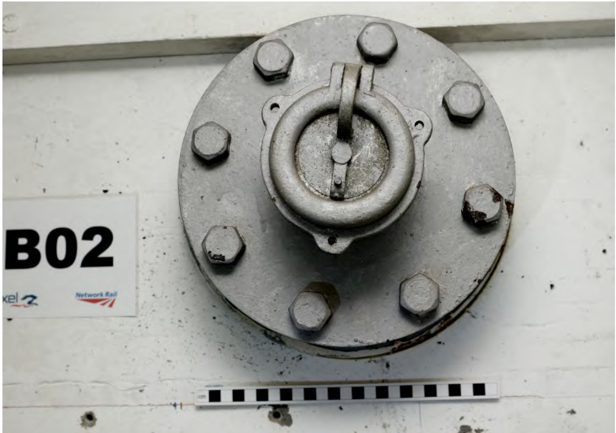
Plate 35: Auxiliary room 2 – pressure relief valve or non-return valve This and the following seven plates depict a centimetre scale
