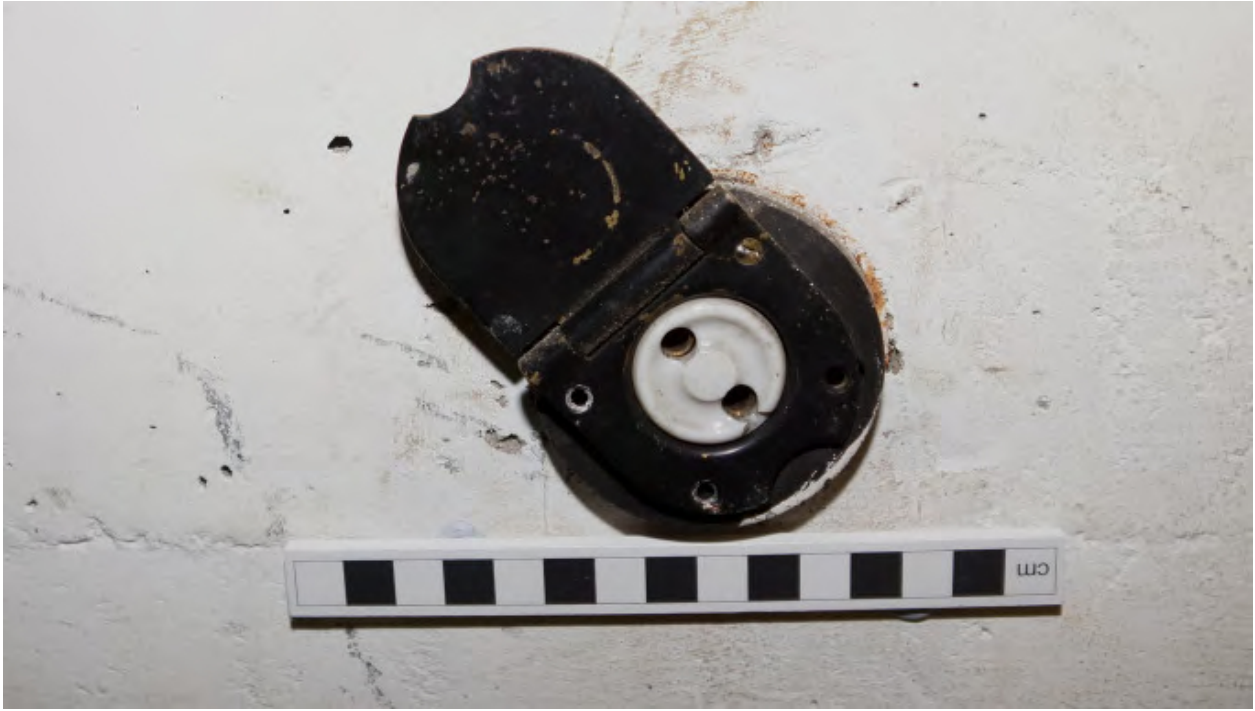
Plate 37: LMS communications wall socket inside rooms 2 and 3 -
