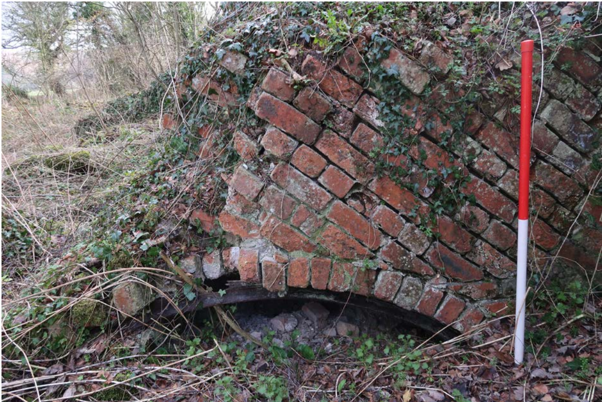
Fig 7: buttress or support for slag mill flue, looking south-east, showing iron lining in arch
