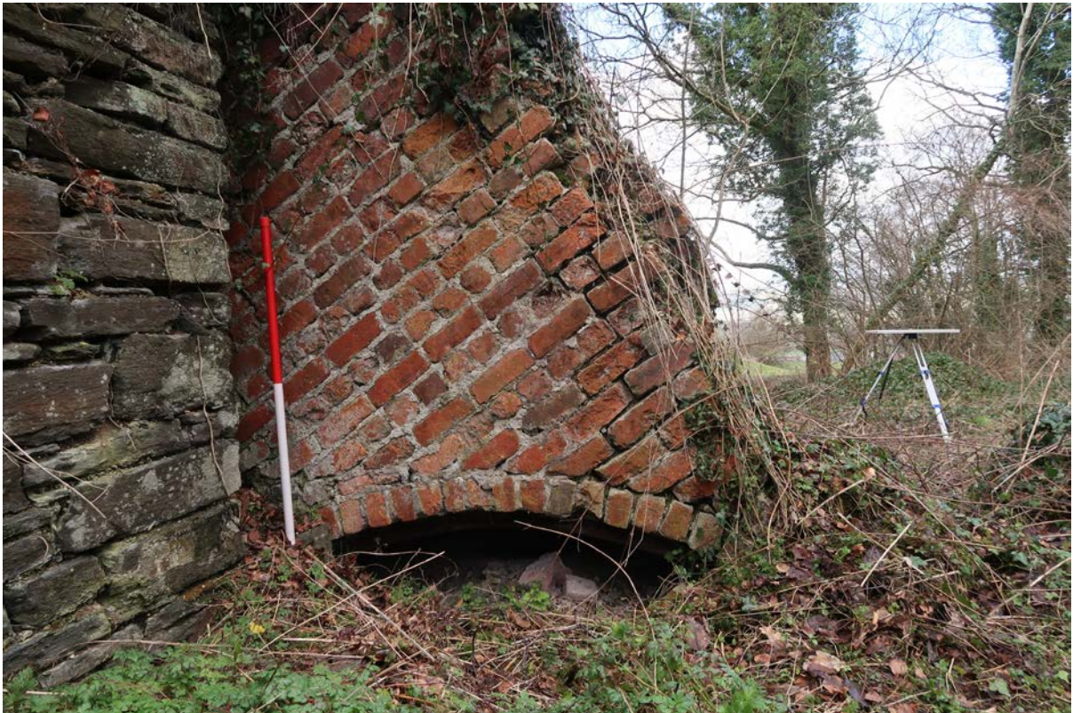
Fig 6: buttress or support for slag mill flue with arched hollow below, looking north-west
