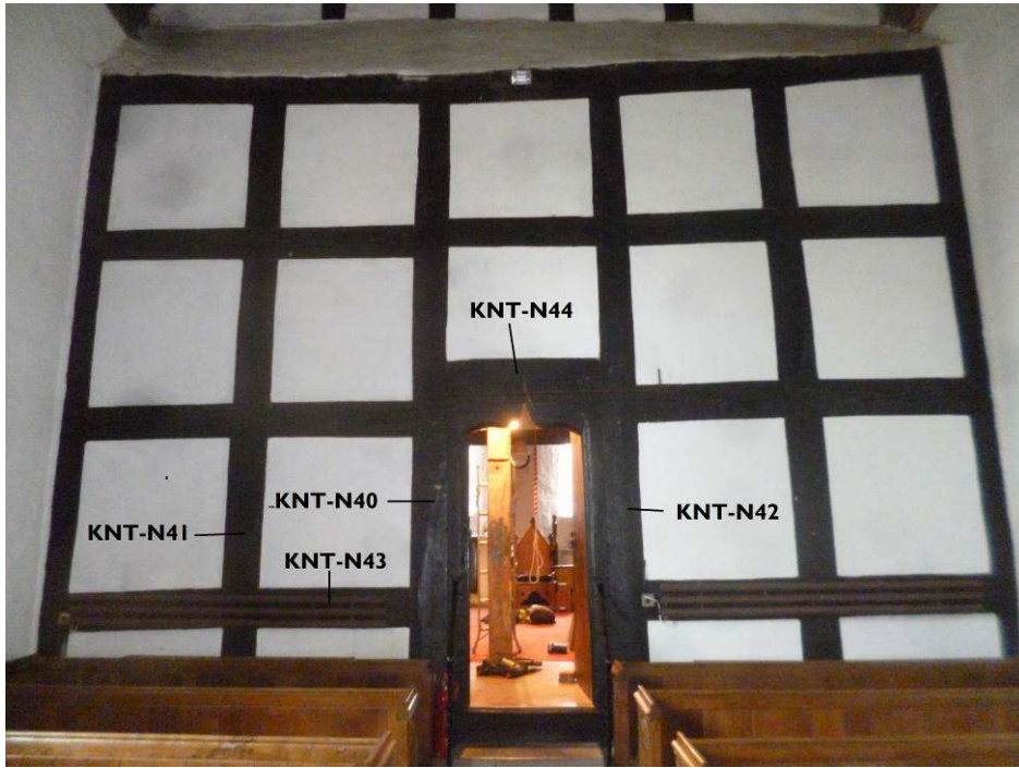
Figure 15: Lower portion of nave partition, showing the location of samples KNT-N40–44, photograph taken from the east (Alison Arnold)
