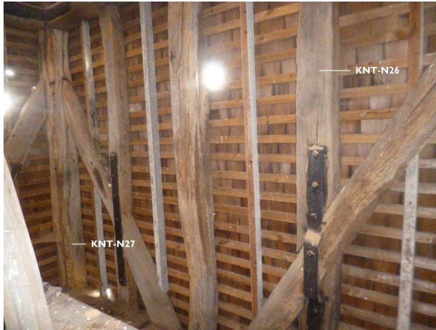
Figure 13: North wall of tower at bellframe level, showing the location of samples KNT-N26 and KNT-N27
