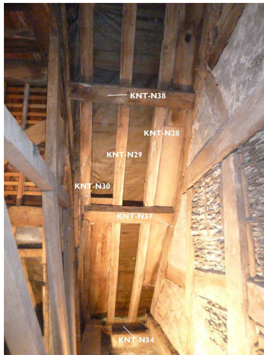
Figure 8: Portion of roof between the tower (to the left) and the nave partition (to the right); location of samples KNT-N28-30, KNT-N34, KNT-N37, and KNT-N38, photograph taken from the south (Alison Arnold)
