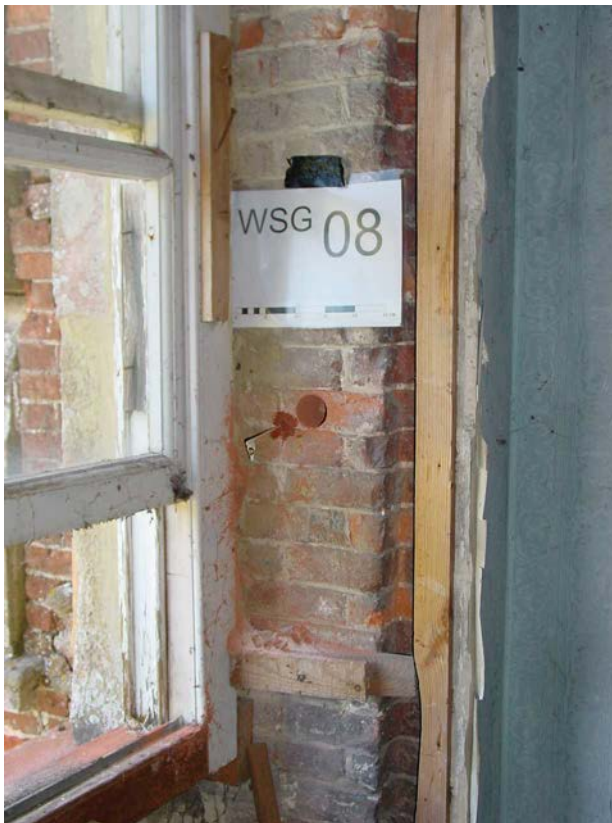
Figure 20: section of interior wall on upper floor adjacent to south-facing window showing locations WSG-08 and dosemeter below (flag D)
