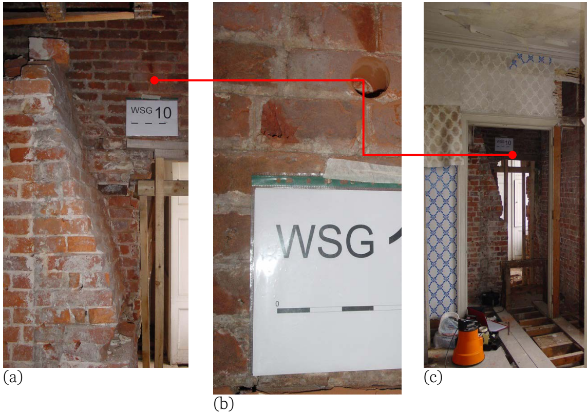
Figure 22: (a) north-facing interior wall on bedchamber floor adjacent to chimney stack in the Southampton Room, showing location of WSG-10, (b) close-up of sampling location WSG-10, (c) general view of location of WSG-10 in relation to west-facing exterior wall
