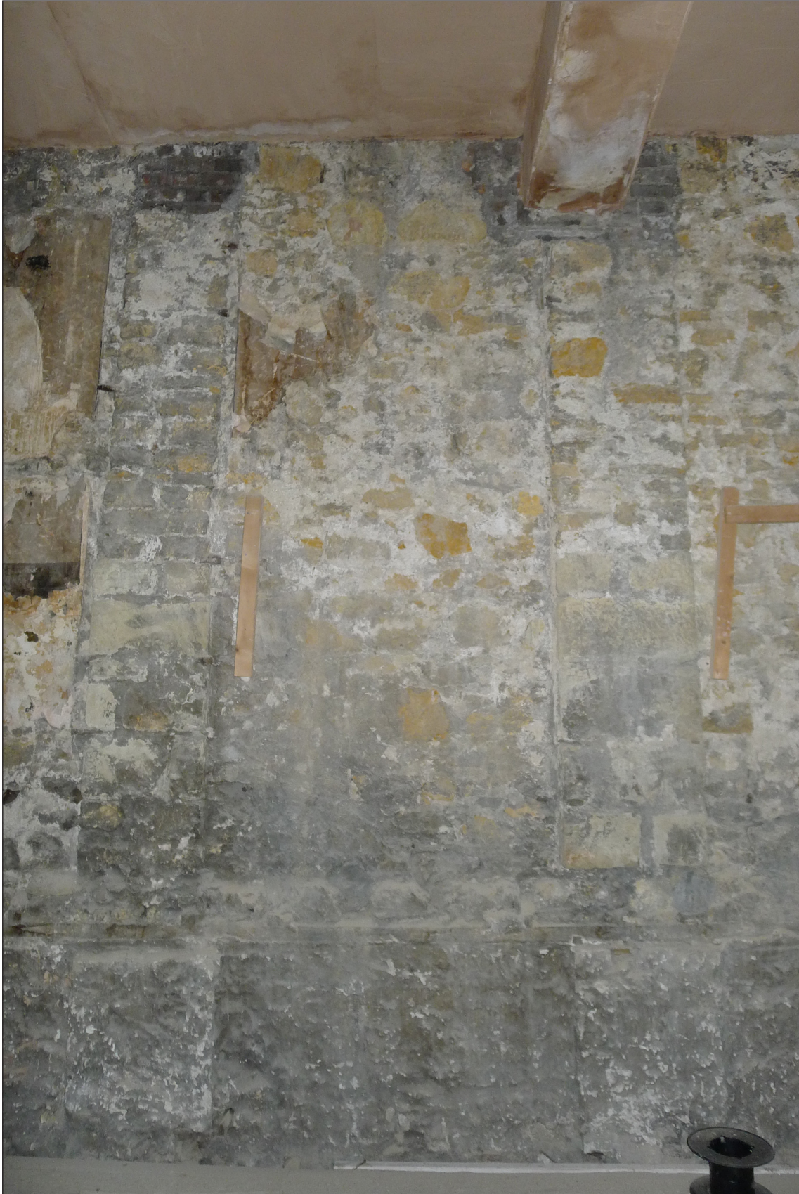
Fig 13: The rubble and ashlar party wall on the ground floor of the Athenaeum, part of the remaining 1840s fabric.. © Historic England / Lucy Jessop.
