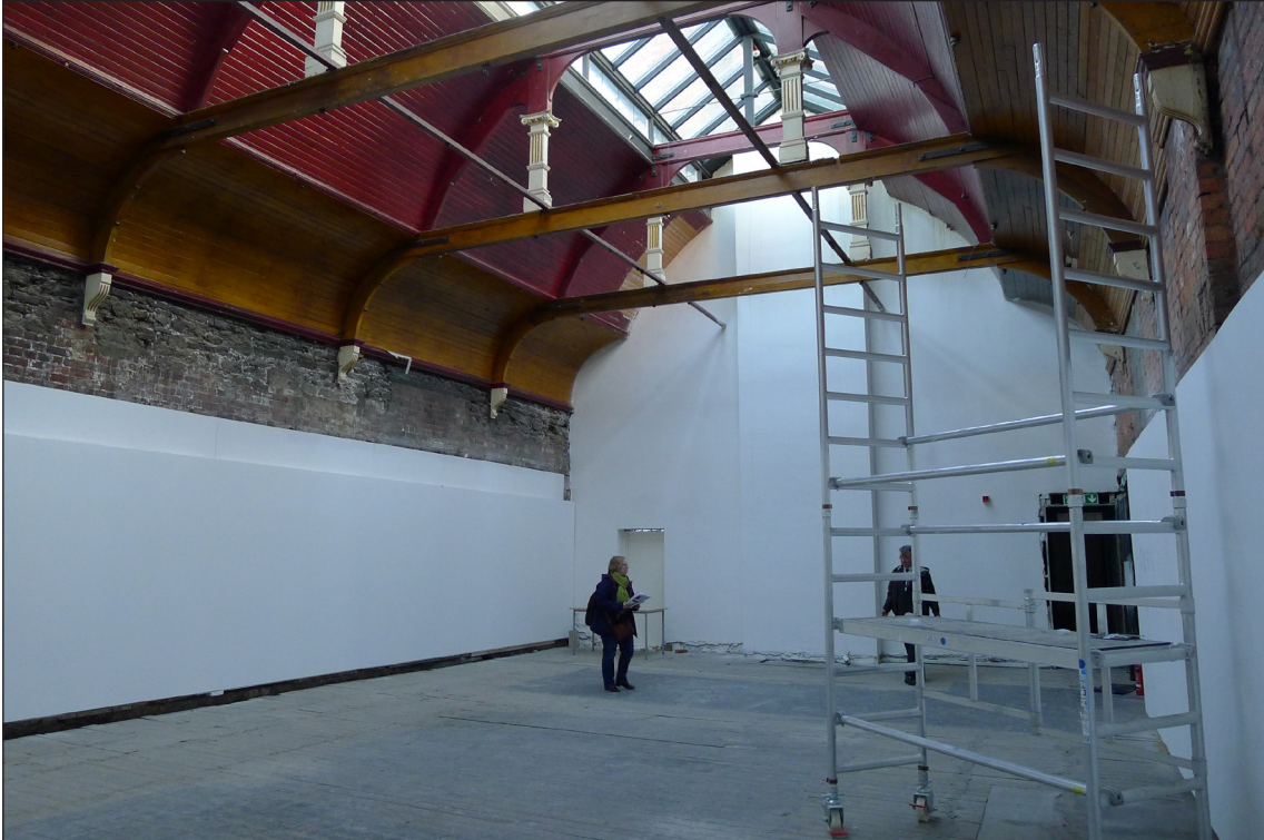
Fig 15: The 1900 billiard room, with its timber trusses with metal strapping, slender reinforcement bars, Ionic queen posts, fluted consoles and the boarded, double coved ceiling. © Historic England / Tristan Wilson.
