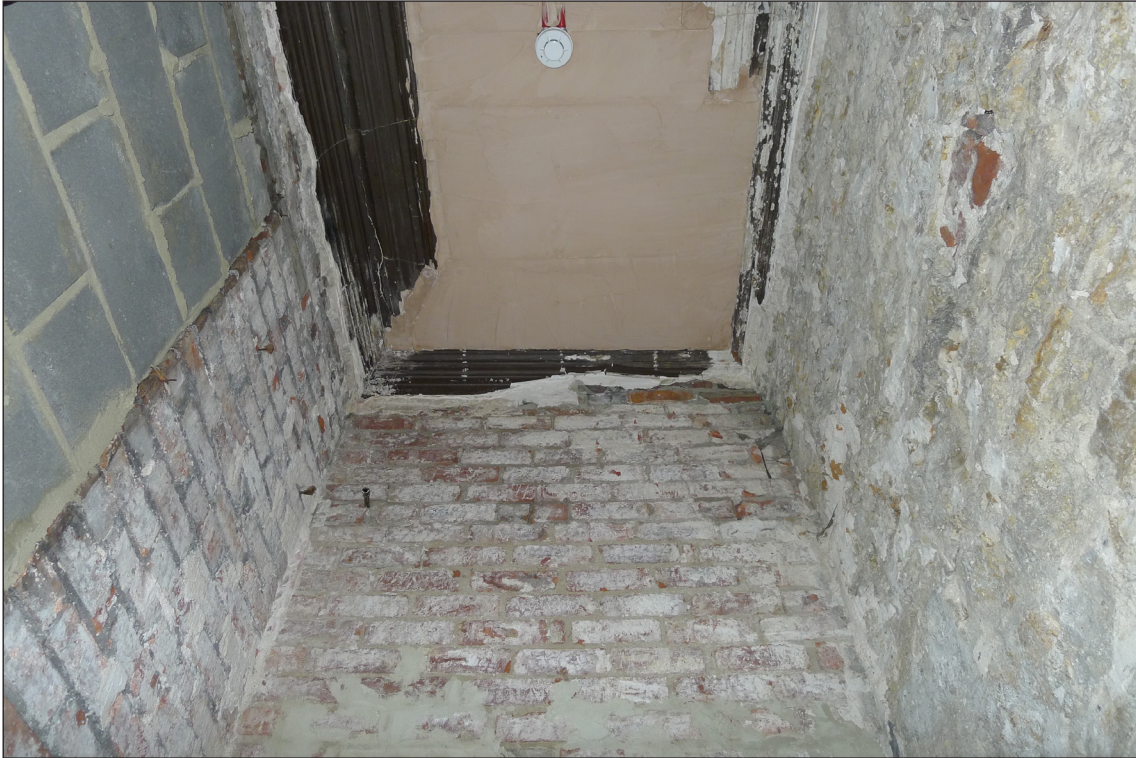
Fig 14: The end of the 1900 corridor on the first floor, looking up above the doorway to the billiard room. To the right is the surviving 1840s rubble internal wall; to the left is a tall blocked window which would have looked onto the middle light well. © Historic England / Lucy Jessop.
