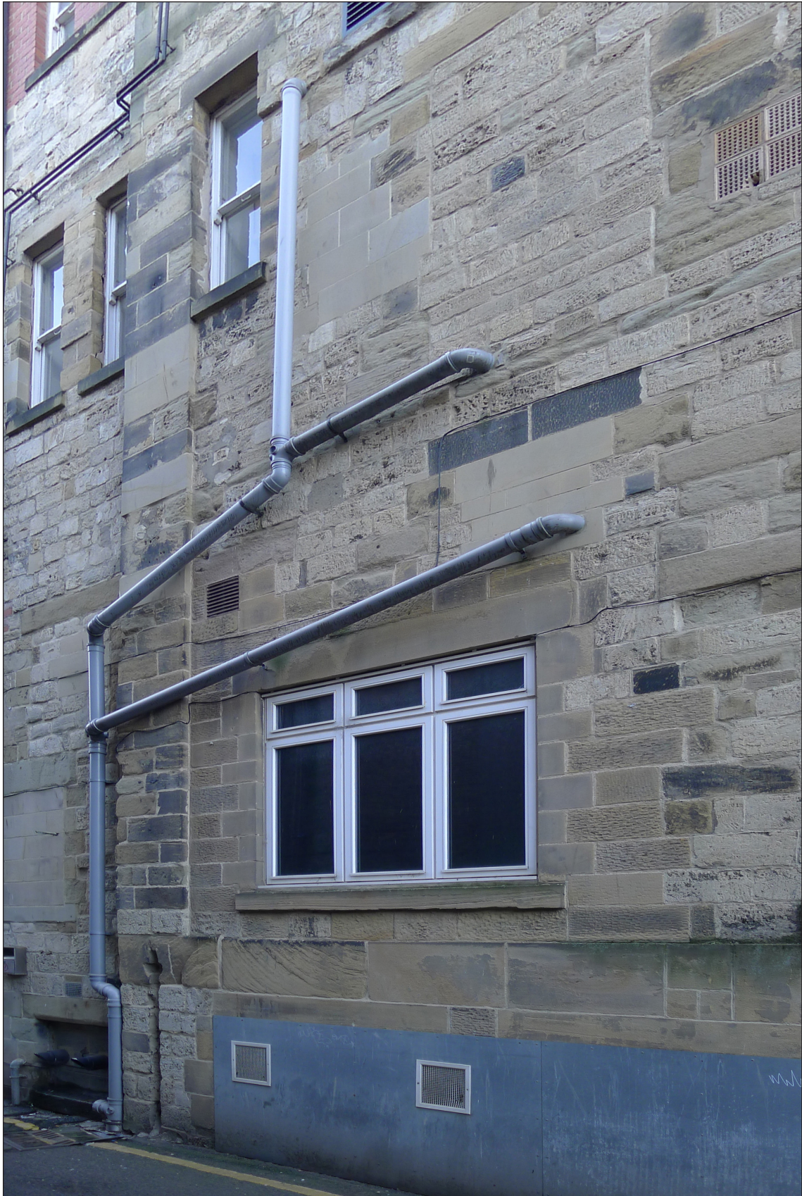
Fig 7: Detail of the eastern elevation facing the rear alleyway, Athenaeum Buildings. The open-textured limestone and sandstone ashlar of the 1840s building, with its projecting corners, can be clearly seen, with later blocked and refenestrated openings. © Historic England / Lucy Jessop.
